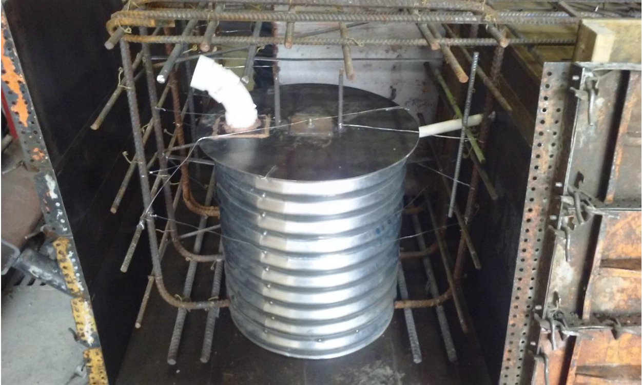
Figure 44. Side view of CMP void
