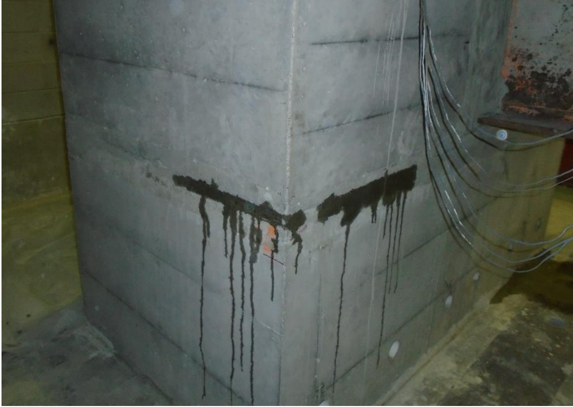
Figure 52. Bleed water passing through the grout bed
