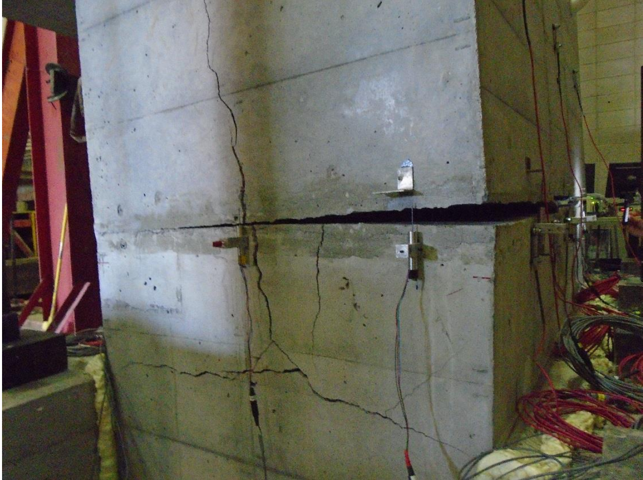
Figure 76. Pile coupler damaged west side
