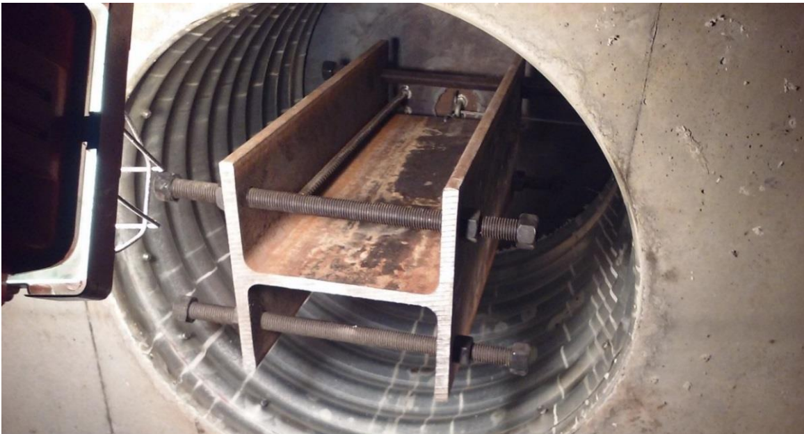
Figure 47. Suspended HP sections
