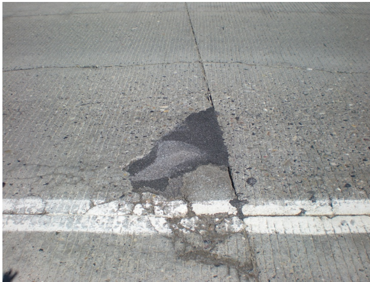
Figure 40 – Nevada, I-80 Typical Distress and Repair
