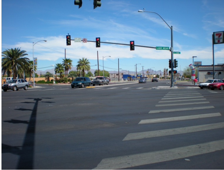
Figure 39 - Lake Mead Boulevard Typical Pavement Condition
