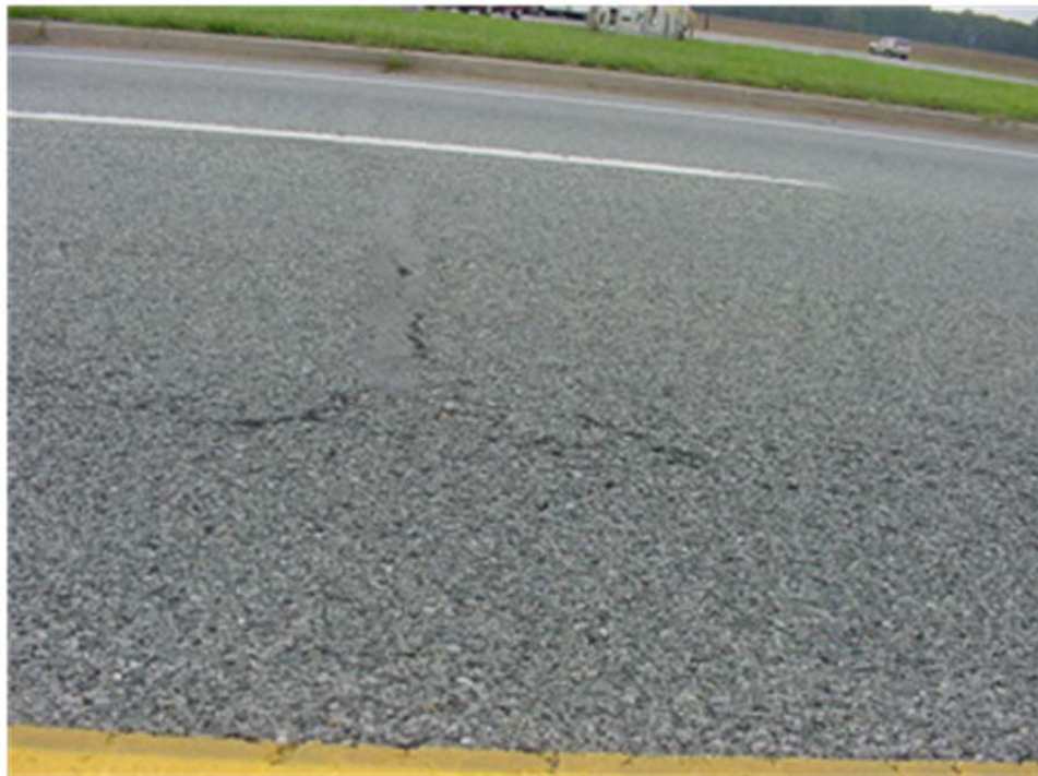
Figure 16 – US-13 Existing Pavement Condition
