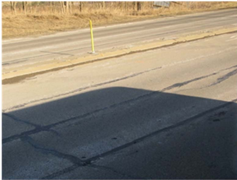
Figure 11 – Typical Existing Distresses on Pennsylvania SR-119 (fatigue cracking, moderate rutting)
