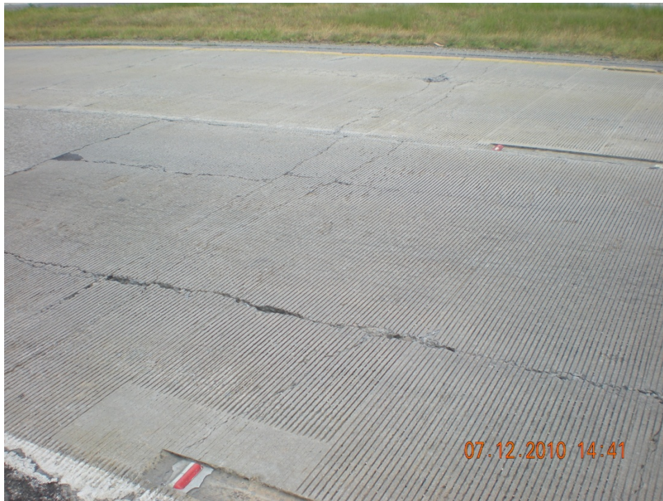
Figure 33 – Distressed Pavement on US-58 in Southhampton County, Virginia
