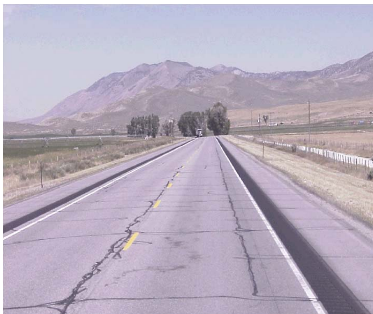
Figure 43 – Wyoming US-30 Existing Roadway Condition
