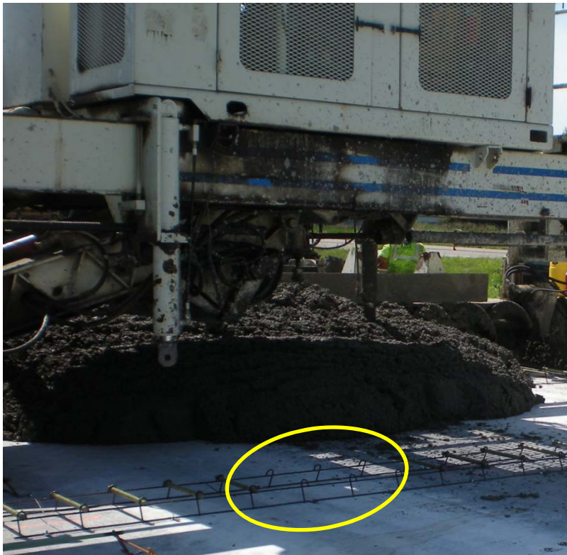
Figure 5 – SD Route 50 Dowel Bar Configuration (note omitted dowels between the wheel paths)
