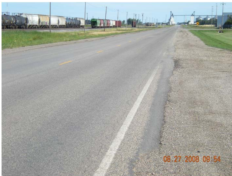
Figure 19 – North Dakota Route 200 Existing Pavement Condition
