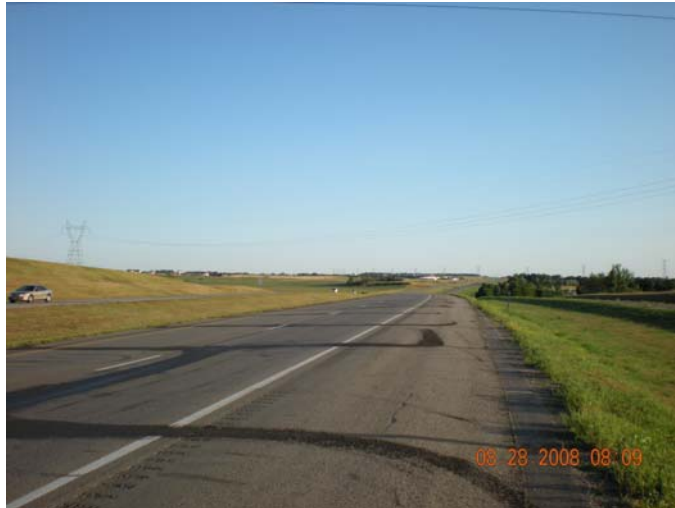
Figure 25 – Existing Condition of US-83 North of Bismarck, ND
