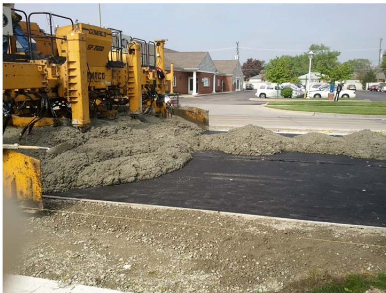
Figure 49 – Placing the 4” Thick Unbonded Concrete Overlay (existing concrete was milled and a geotextile separation layer used)
