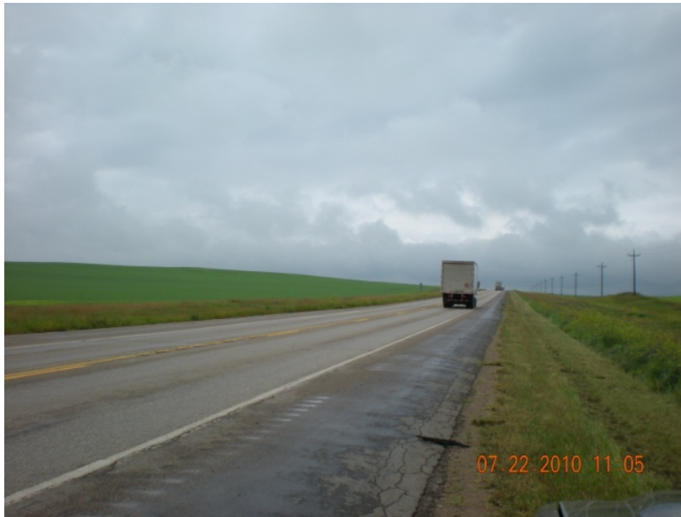
Figure 28 – ND Route 85 Watford City to Alexander, Representative Pavement Condition
