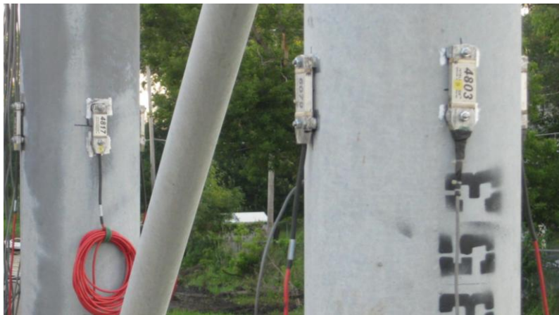
Fig. 27 View of a strain gage attached on a large member of the truss
