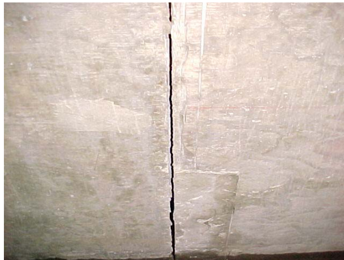
Figure 85. Crack Opening at Construction Joints in Box Culvert
