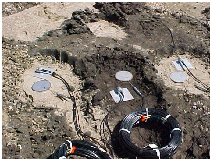
Figure 33. Settlement Cells and Total Stress Cells at Geopier Site
