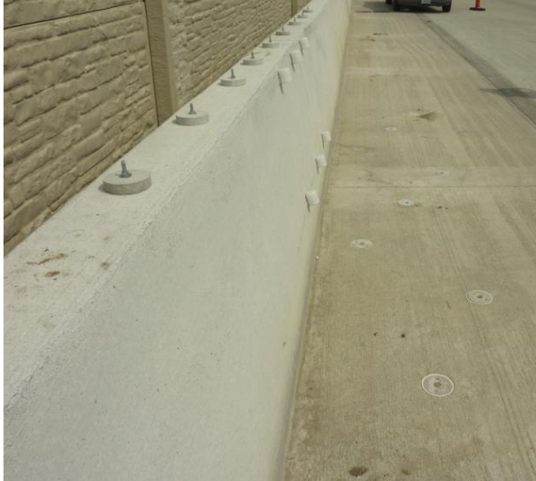
Figure 62. Coupon placement at both paved shoulder (nine each) and top of crash barrier locations (nine each)
