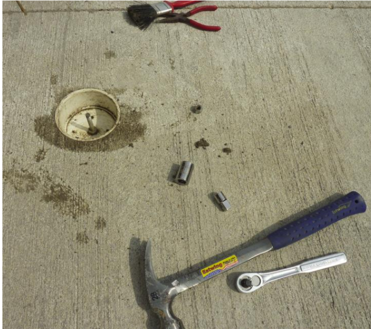
Figure 65. Coupon sample collection underway showing open pavement coupon mounting hole with accompanying mounting bolt
