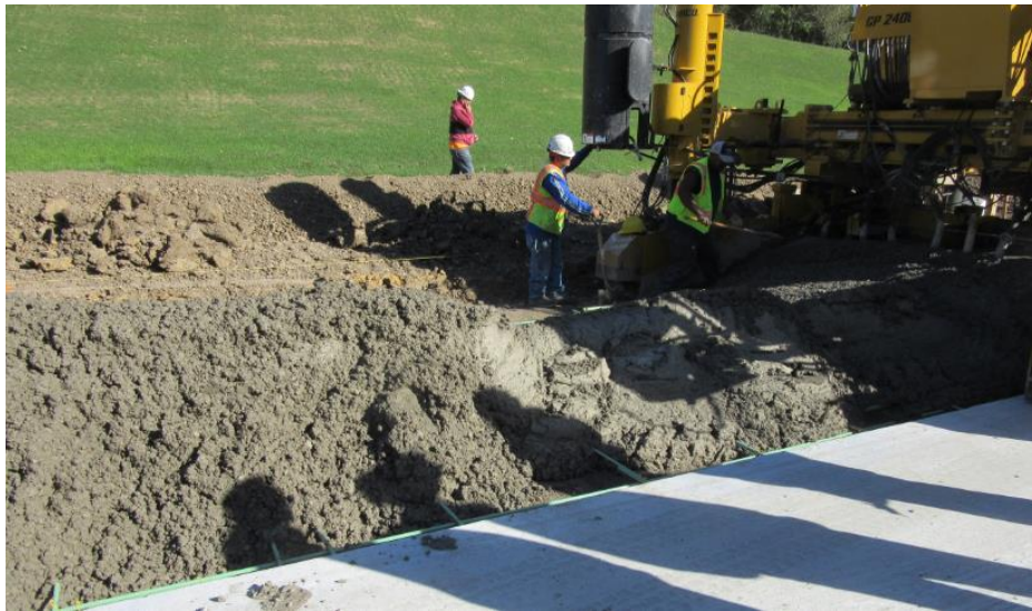
Figure 11. Comparison between two batches of concrete used on Site 2 (wet on the right and dry on the left)
