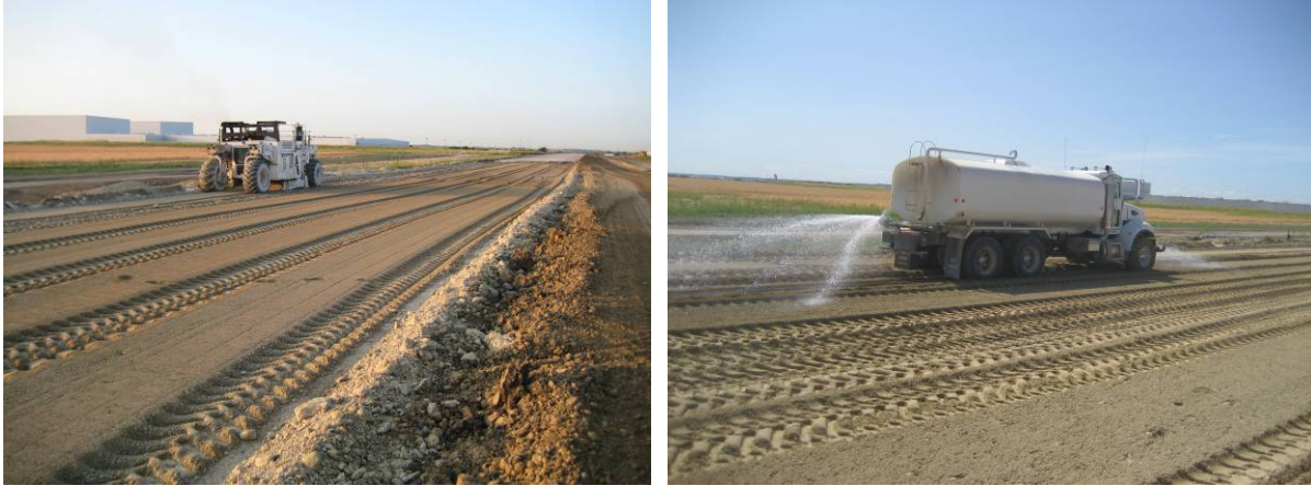
Figure 26. Picture showing soil reclaiming (left) and moisture conditioning process on TB 5 (picture taken 07/23/2008)
