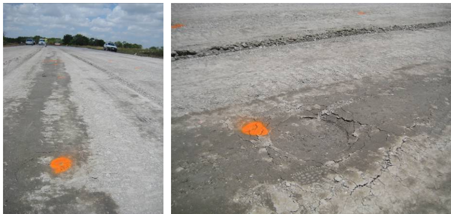
Figure 40. Moisture segregation on flex base material during testing (TB 7)
