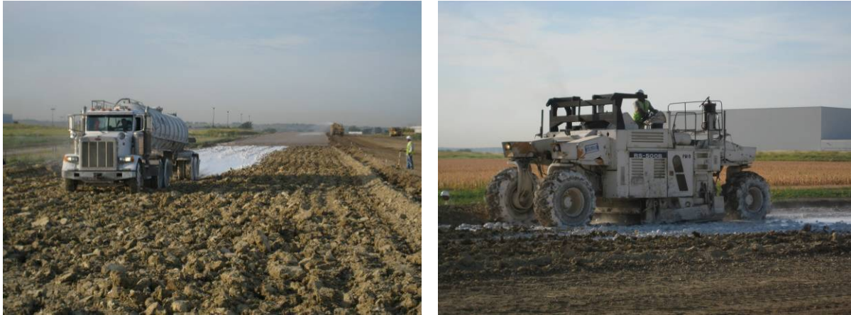
Figure 24. Photos showing placement (left) and reclamation (right) process of lime slurry with existing subgrade material (pictures taken 07/21/08)
