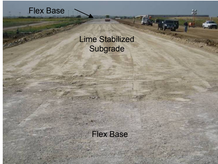
Figure 19. Picture of TB2 with flex base (on both ends of the test bed) and lime stabilized subgrade
