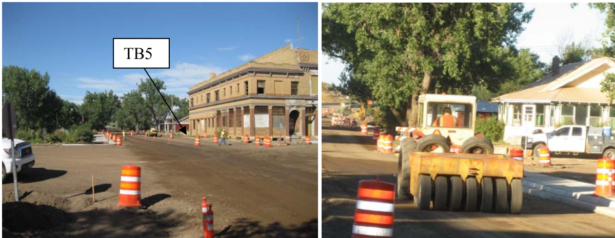
Figure 45. TB5 location (left) and pneumatic roller used for compaction of base layer on TB5 (right)
