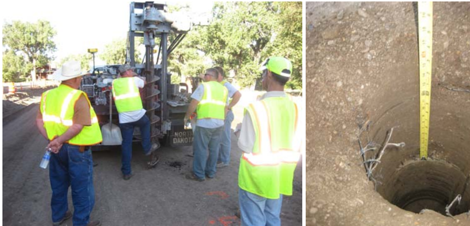
Figure 44. Photographs of drilling equipment and bore hole drilled for BST on TB4
