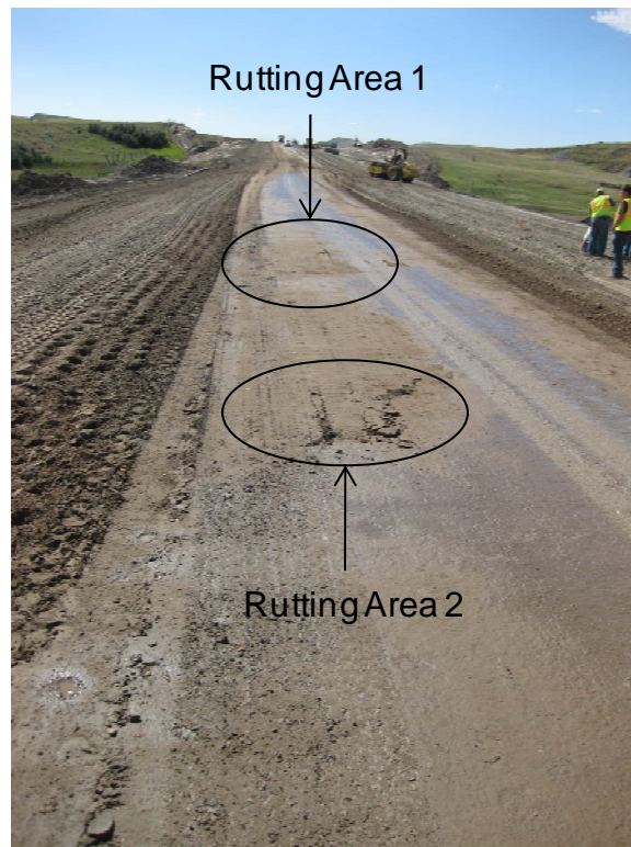
Figure 29. Picture of TB2 showing visually identified soft areas
