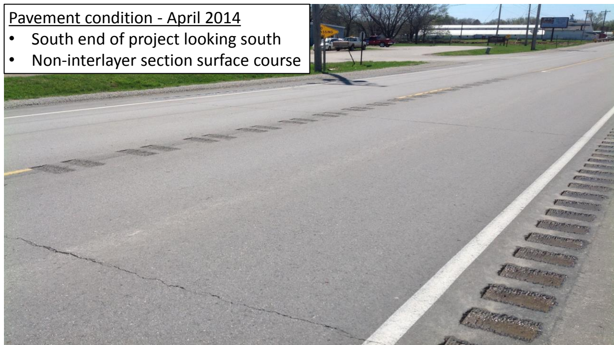
Figure 12. Reflective cracks in non-interlayer overlay on US 169 in April 2014
