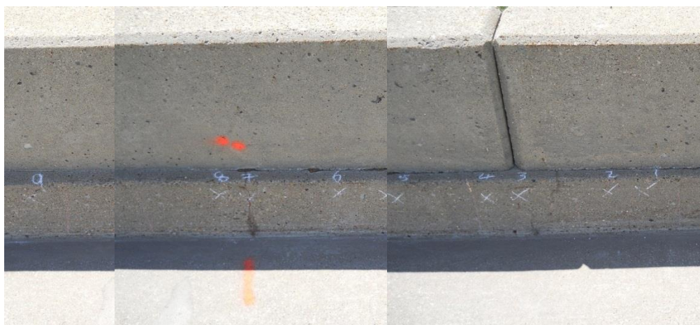
Figure 57. Suspect locations on the east end of the bridge
