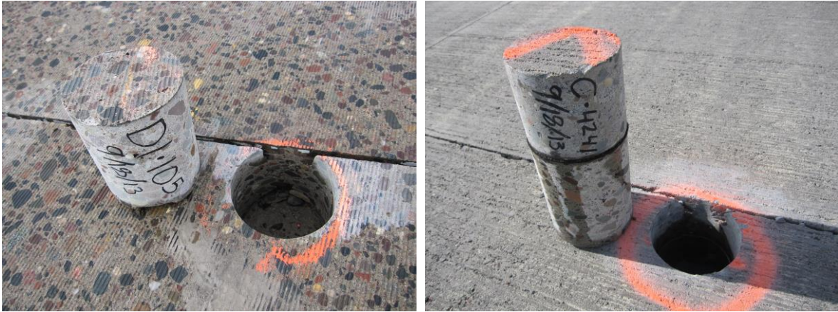
Figure 4. Example cores retrieved in 2013 showing the relationship of the core next to the joint: Joint 105, Cell 9 (left) and Joint 4241, Cell 505 with fabric bond-breaker (right)
