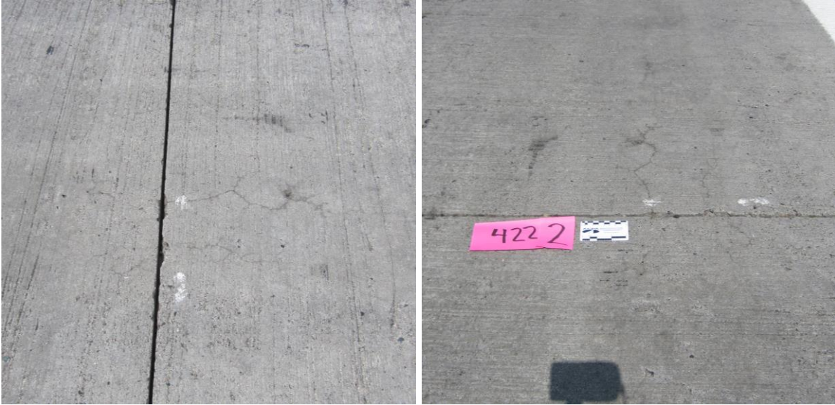
Figure 47. Cracking in the wheel path observed in Cell 505, an unbonded concrete overlay
