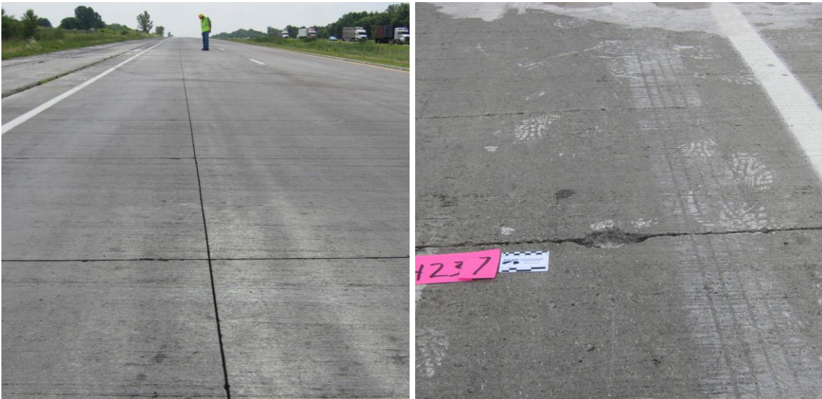
Figure 48. Edge breaks observed just outside the wheel path in Cell 505, an unbonded concrete overlay
