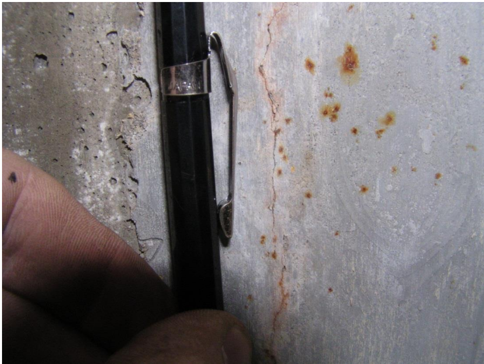
Figure 4.16. Close-up of cracking and efflorescence observed between modules 2 and 3 on bottom of deck
