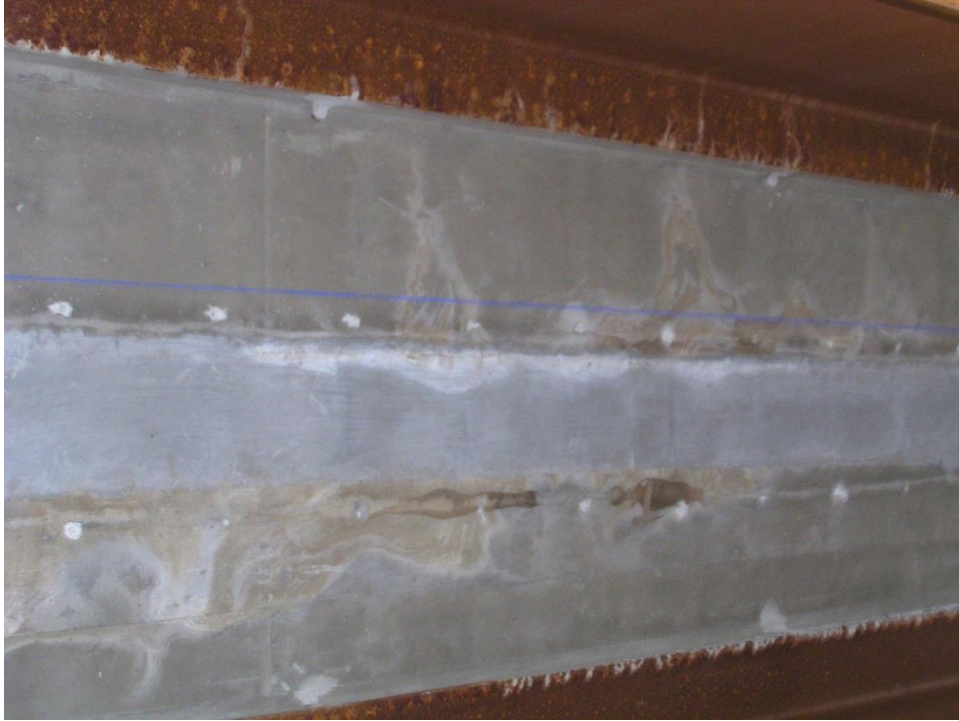
Figure 4.15. Observed efflorescence between modules 2 and 3 on bottom of deck
