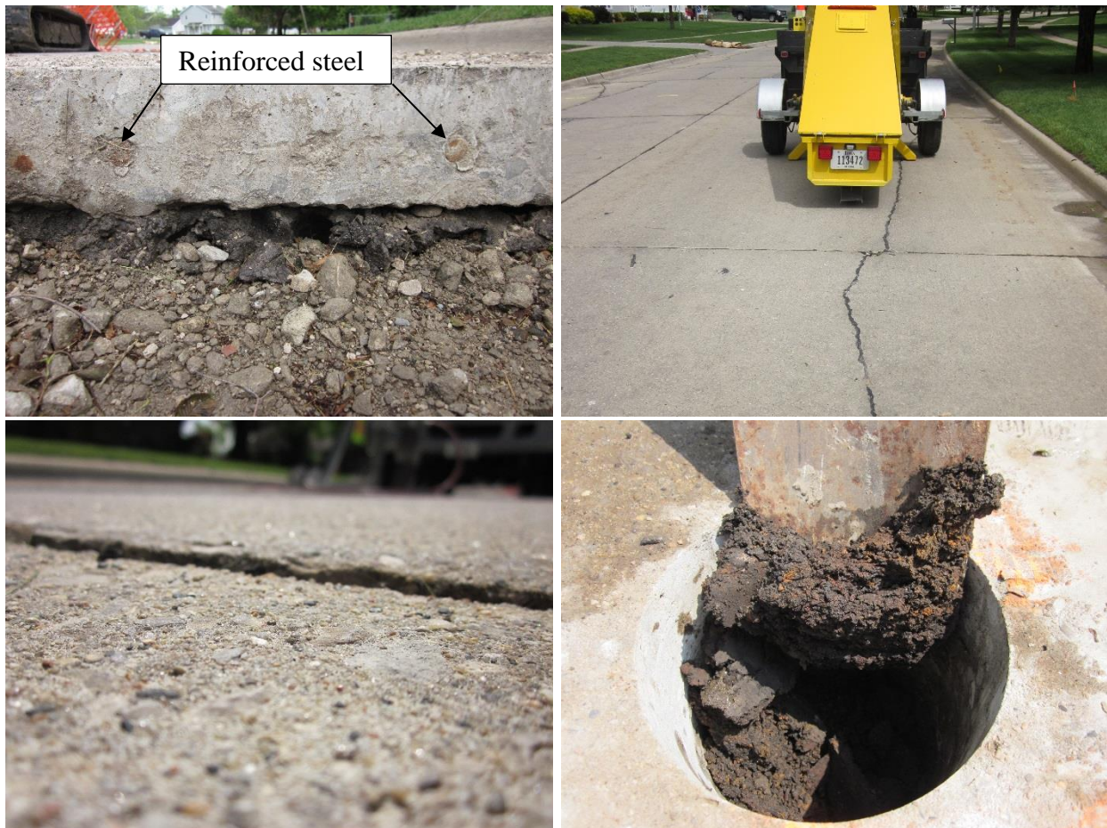
Figure 41. Photographs of field test site during testing — NW 5 th Street and Greenwood Drive, Ankeny
