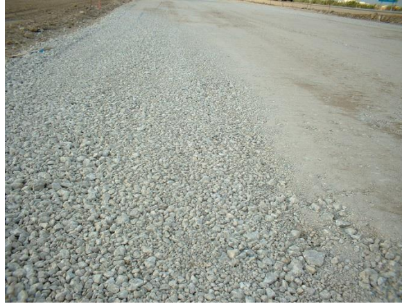
Figure 2. Visual indication of aggregate segregation following trimming and compaction operations on a recycled PCC material on I35 in Hamilton County, Iowa
