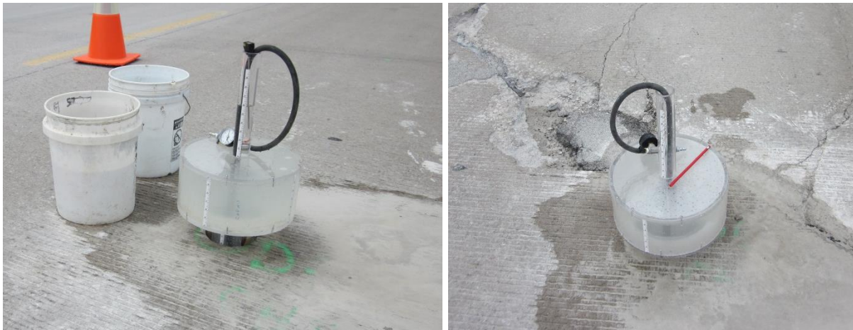
Figure 59. Photographs of good panel with CHP#1 test (left) and cracked panel with CHP#2 test (right) —Riverside Road, Ames
