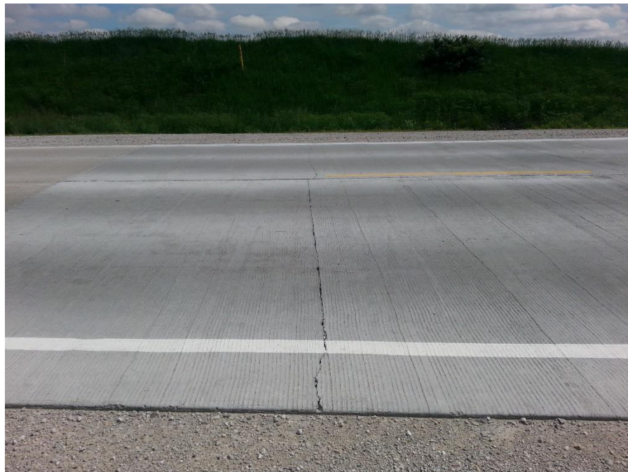
Figure 60. Photographs of panel # 4 with mid-panel transverse crack during testing (top on June 7, 2012) and after patching (bottom on June 10, 2013)—Riverside Road, Ames
