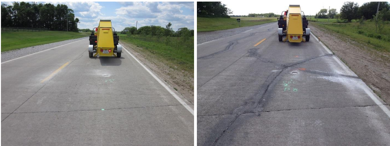
Figure 52. Photographs of good panel with CHP#1 test (left) and cracked panel with CHP#2 test (right) — E63, Story County
