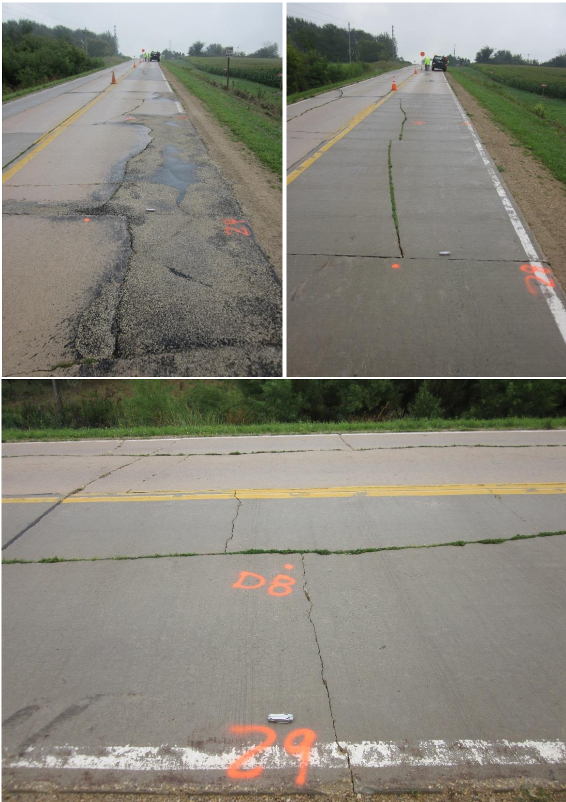
Figure 129. Photographs of new patching areas — 175 th Street, Winneshiek County
