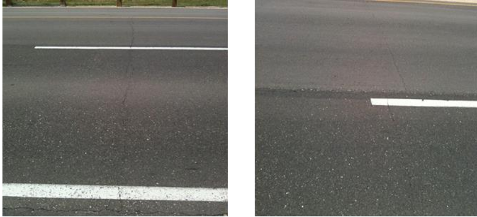
Figure 44. Longitudinal joint performance for the IA 13 project
