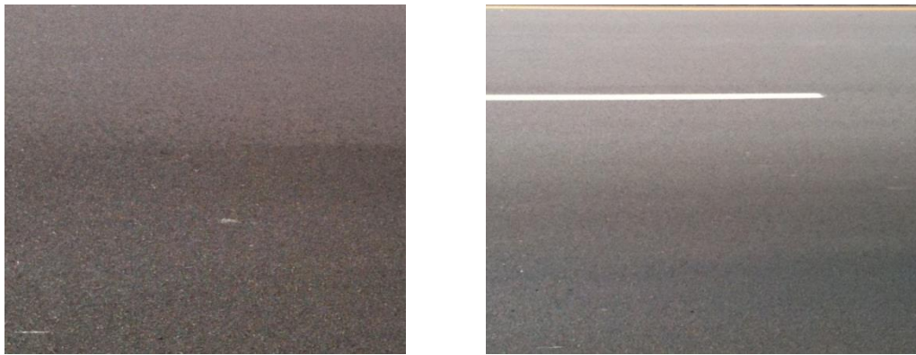
Figure 45. Longitudinal joint performance for the I-35 project
