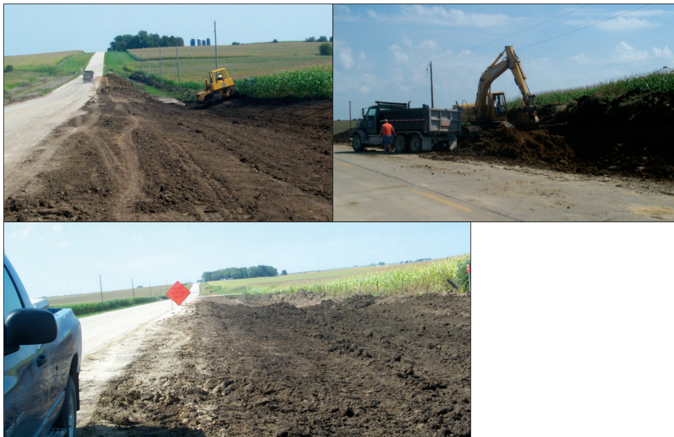
Work in progress on Buchanan County local road (photos courtesy of Brian Keierleber)
