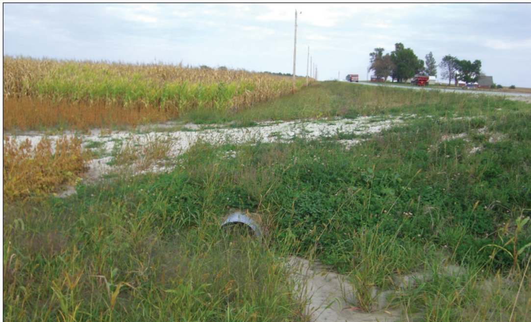
Additional culvert provided to flatten entrance slopes (photo courtesy of Bob Sperry)
