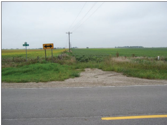
Entrance provides safety ramp at T intersection (photo courtesy of Bob Sperry)
