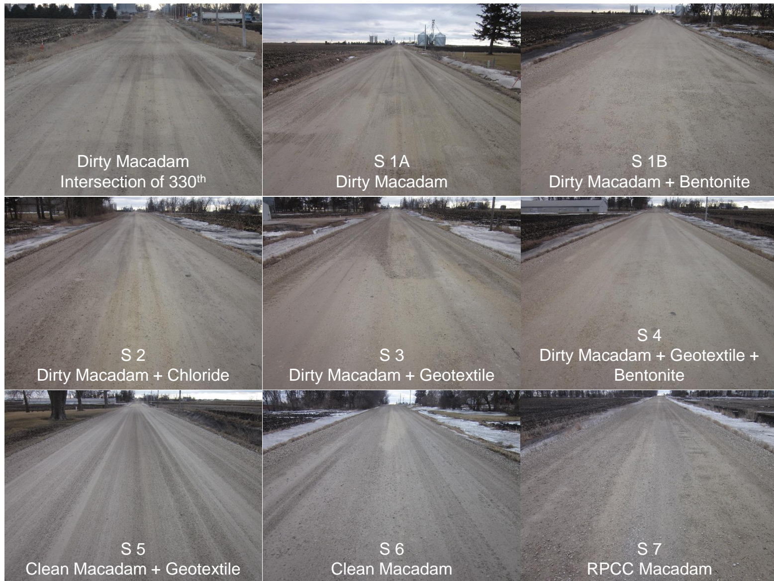
Figure 130. Survey photos of Vail Avenue demonstration sections (January 20, 2015)
