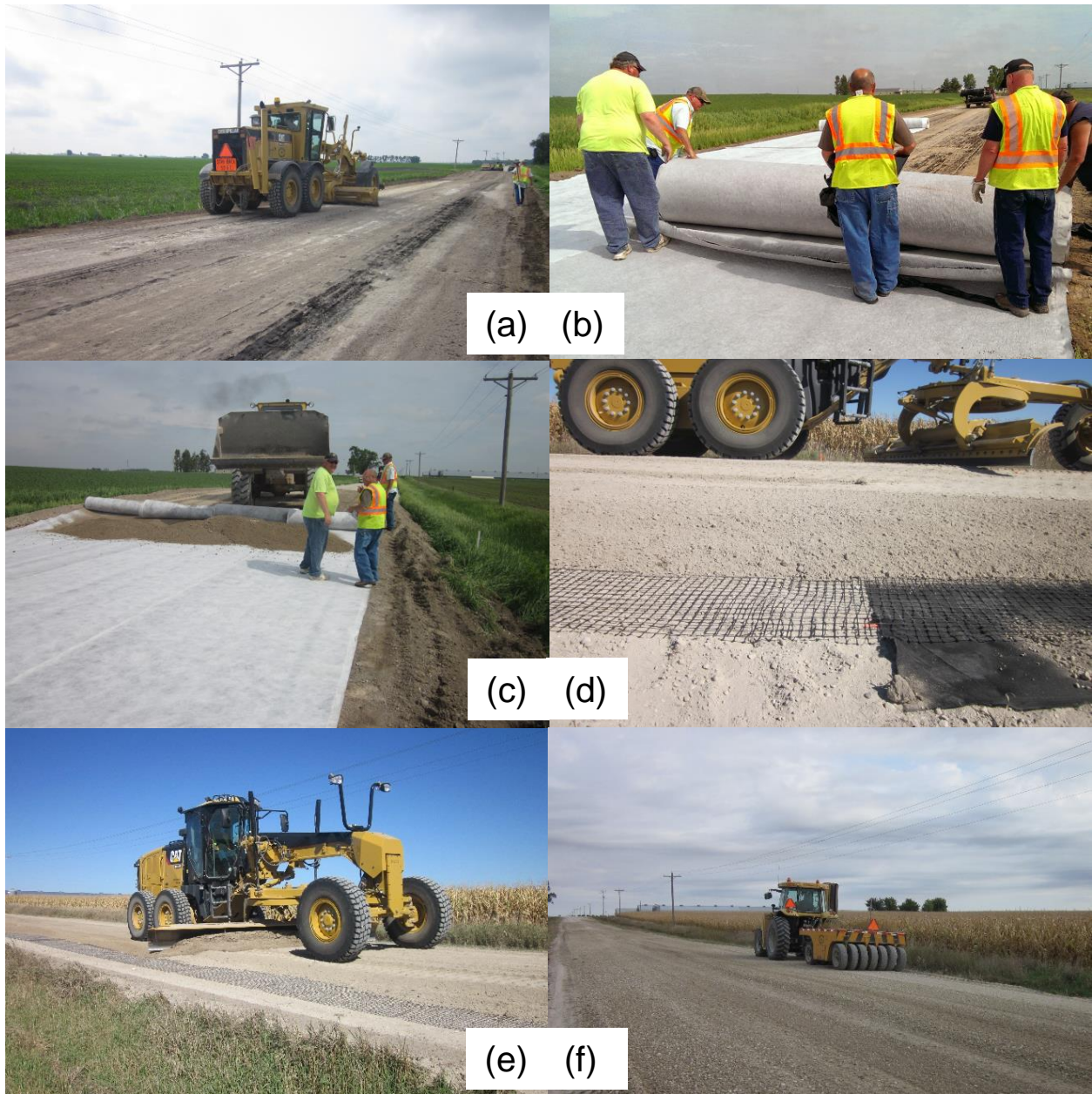
Figure 42. Construction procedures and equipment for geosynthetically stabilized sections: (a) removal of existing surface, (b) geocomposite in Section 18, (c) replacement of surface course by earth mover for geocomposite Section 18, (d) BX geogrid in Section 19B on left with added non-woven geotextile in Section 19A on right, (e) replacement of surface course by motor grader for Sections 19A and 19B, and (f) compaction by rubber-tire compactor
