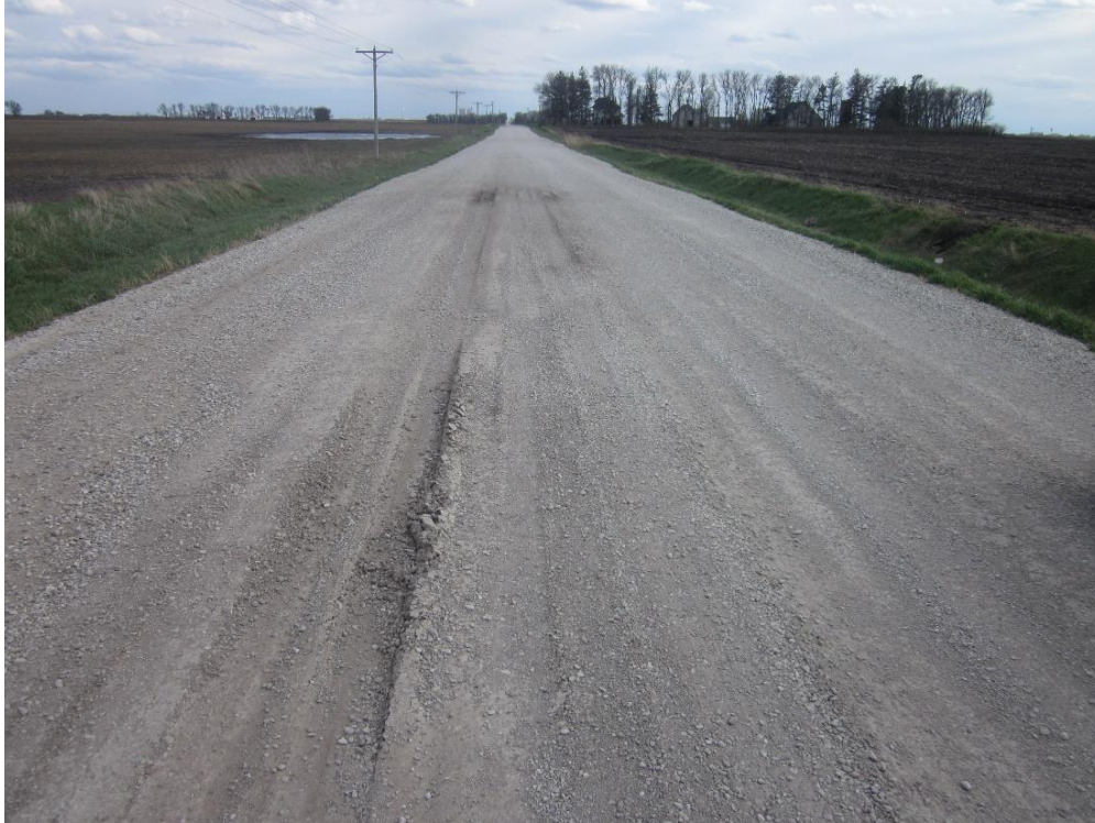
Figure 102. Surface condition of geocomposite drain Section 18 showing rutting (April 21, 2015)
