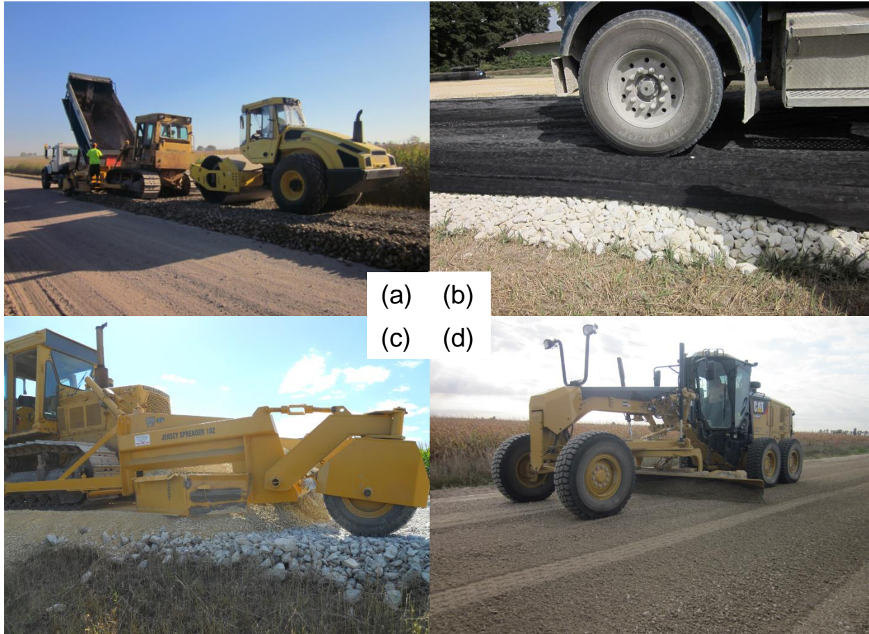
Figure 37. Construction procedures and equipment for Sections 1-8 with macadam base courses: (a) placing macadam with Jersey spreader, (b) non-woven geotextile interlayer, (c) spreading choke stone with Jersey spreader, and (d) shaping with motor grader
