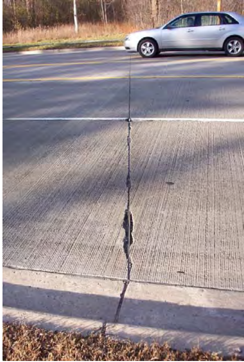
Figure 1. 12 Mile Road in Franklin, six years old
