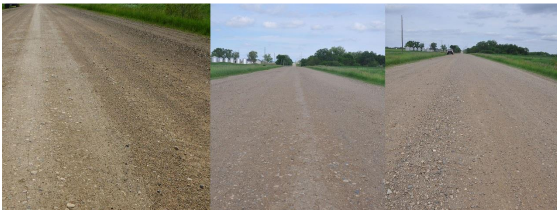
Figure 11. West section of 210th Street at different times: May 28 (left), June 3 (middle), and June 4 (right); blading occurred before May 28 and after June 4
