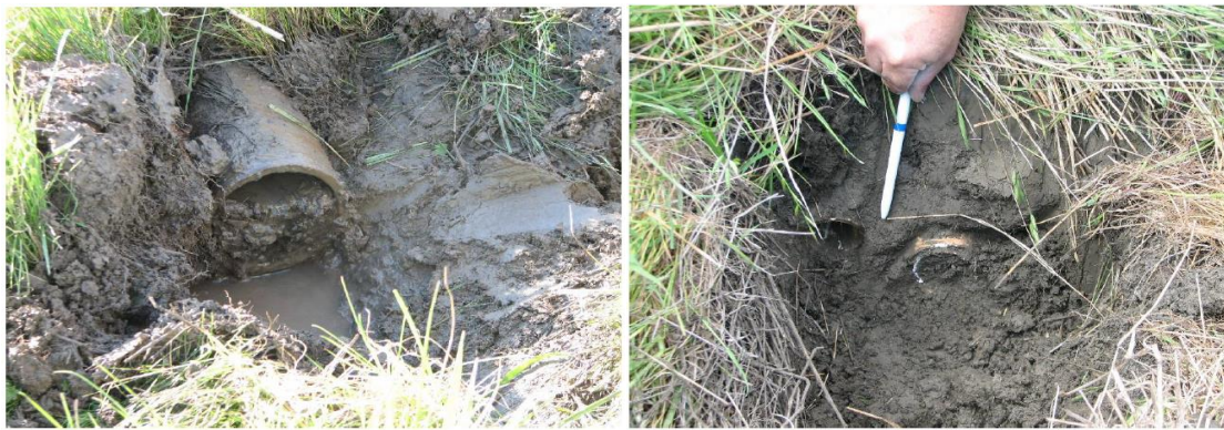
Figure 7. Clogging of edge drain outlet pipes in California PCC pavements (Bhattacharya et al. 2009)
