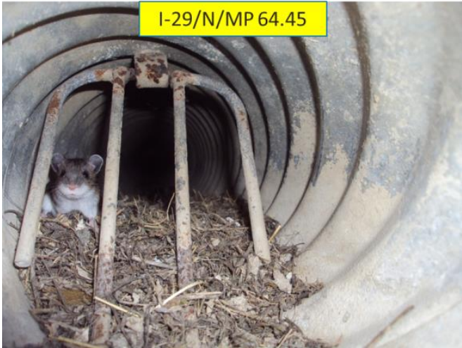
Figure 24. Rodent evidence inside a subsurface drainage outlet during field investigations
