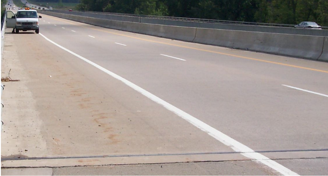
Figure 28. M 45 westbound bridge deck (note snow plow abrasion on shoulder)
