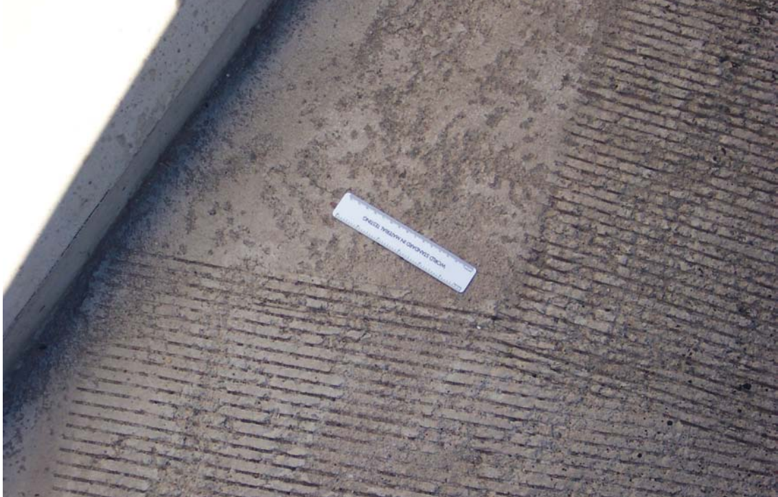
Figure 11. Scaling noted on bridge deck #1863, ramp to Whitehead Highway, SR 598
