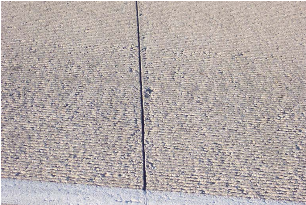
Figure 1. Highway 520 eastbound at mile post 156.45 (note features parallel to joint)
