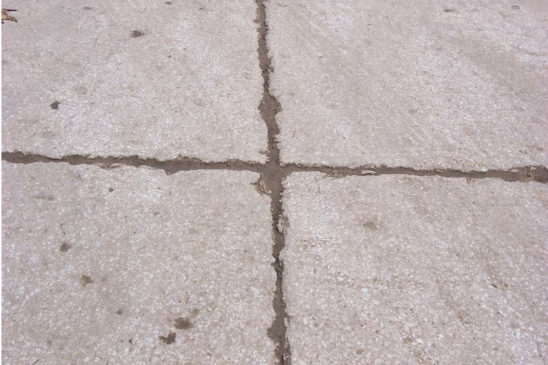
Figure 24. Close-up view of Figure 23 showing abrasion and joint breakage in the slab
