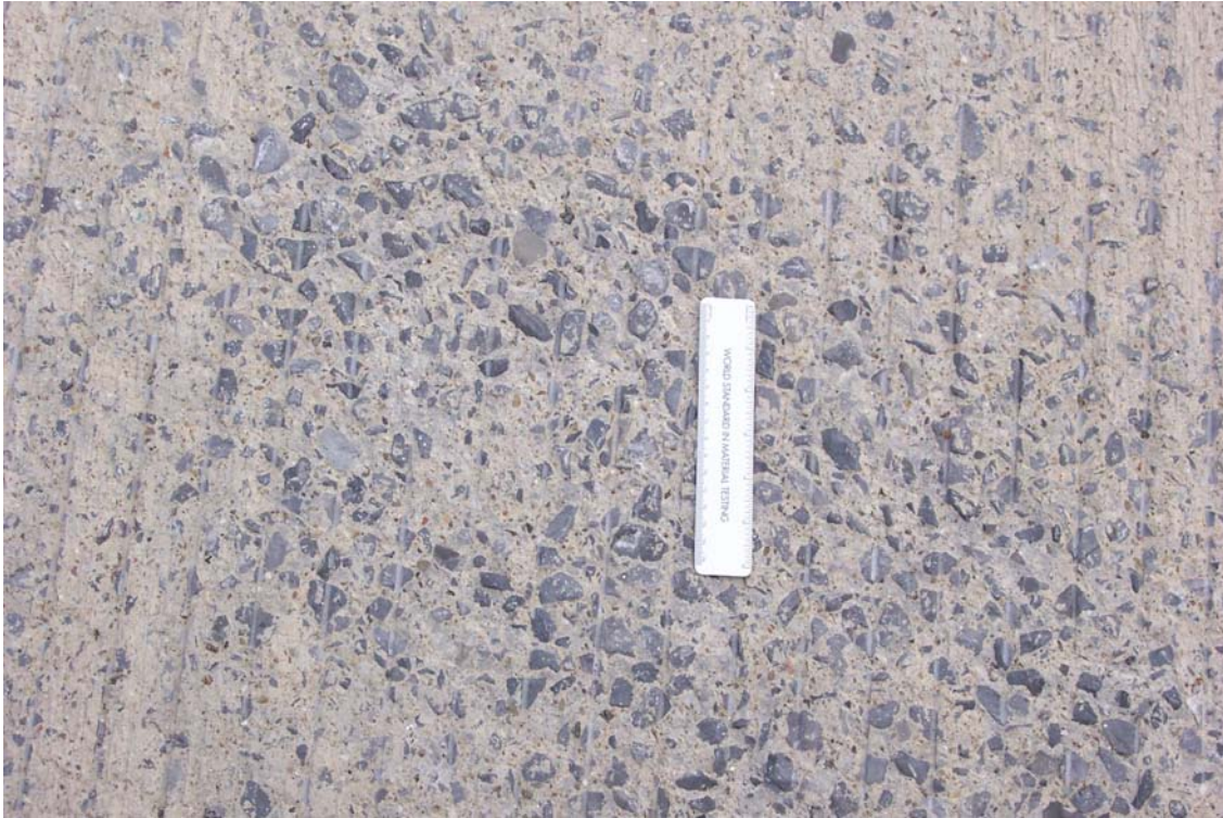
Figure 38. Close-up of scaling on Taconic St. Parkway bridge, southbound deck
