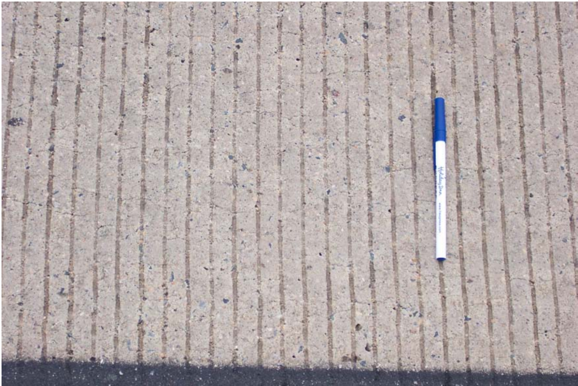
Figure 16. Delaware SR 896 southbound (between US 40 and Highway 71) (note faint cracking)
