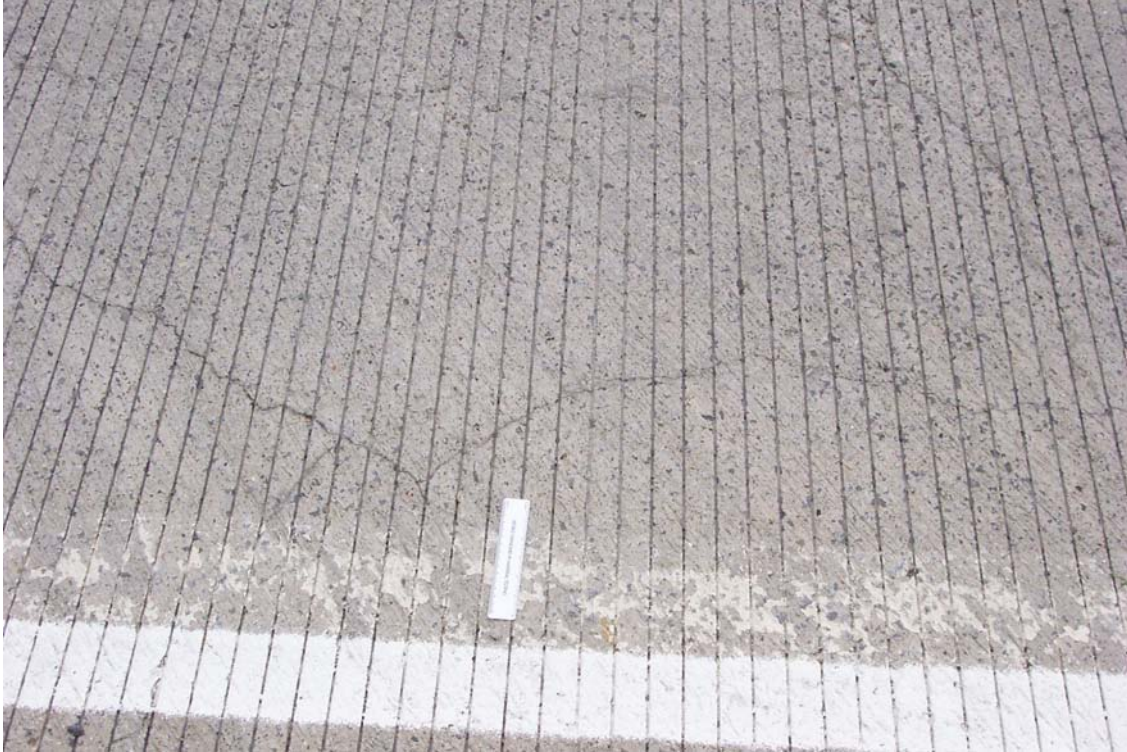
Figure 35. Close-up of exposed aggregate and random cracking on the Route 351 deck
