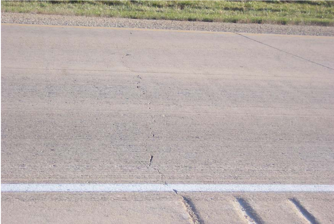
Figure 5. Highway 151 southbound at mile post 45.75 (note transverse cracking through panel)
