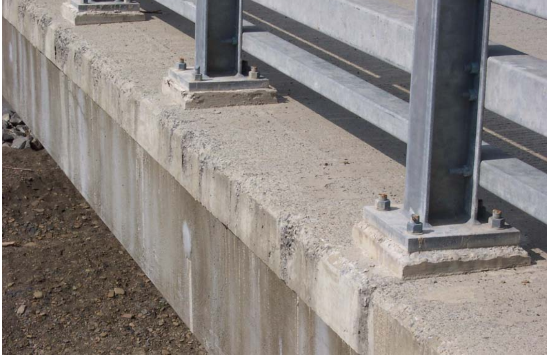
Figure 31. Closeup view of durability issues on the deck
