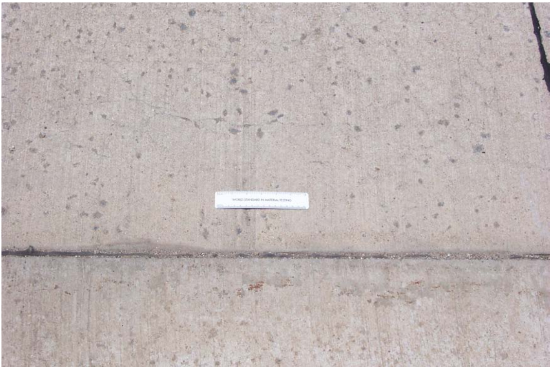
Figure 20. Close-up view of Figure 19 showing faint random cracking in the slab
