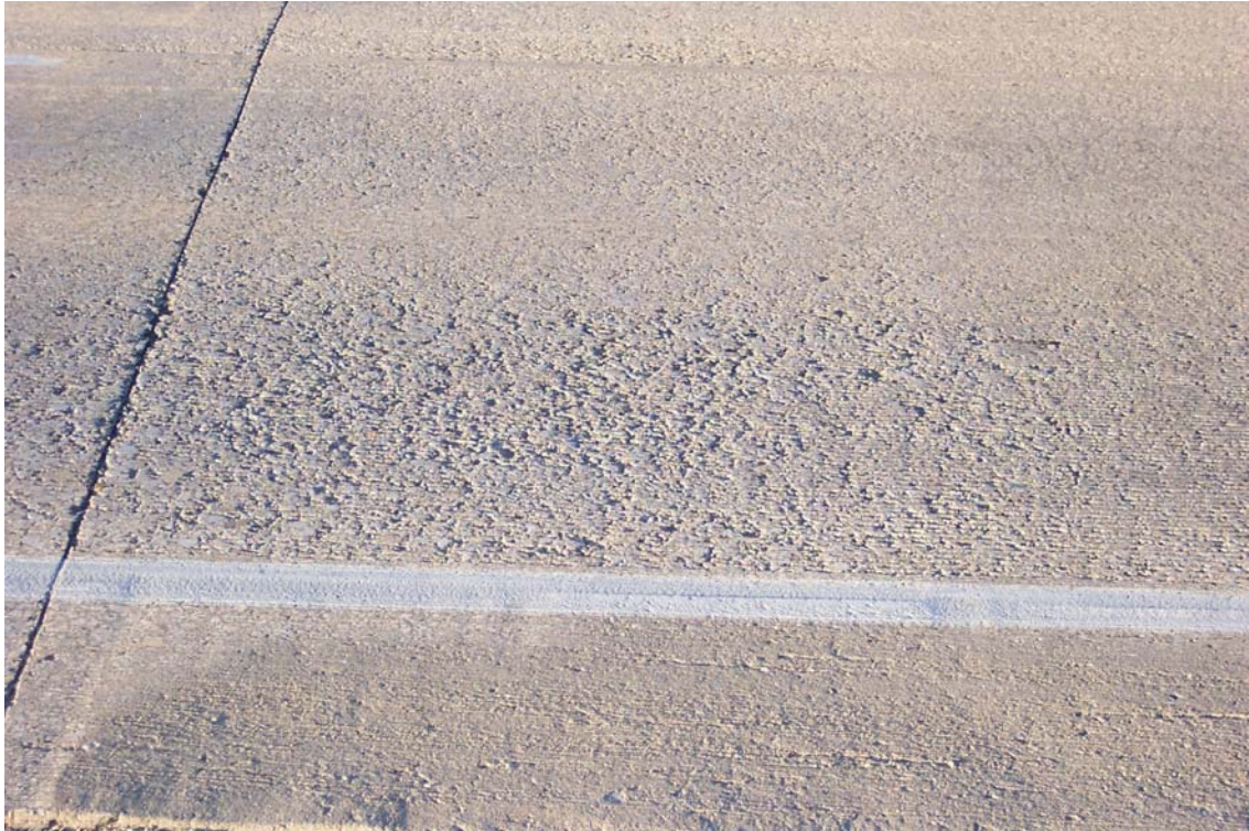
Figure 2. Highway 520 eastbound at mile post 157.20 (note poor surface finish in driving lane)
