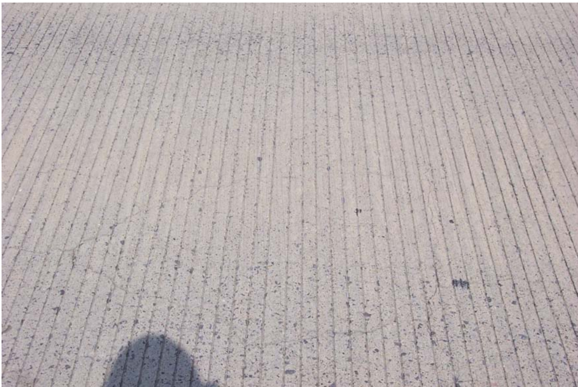
Figure 30. Close-up view of Figure 29 showing wheel abrasion on the slab
