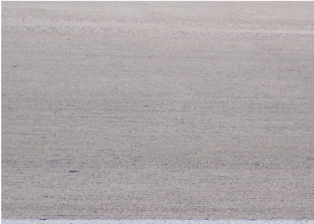
Figure 4. I-35 northbound at mile post 143.45 (note snow plow abrasion on crown)
