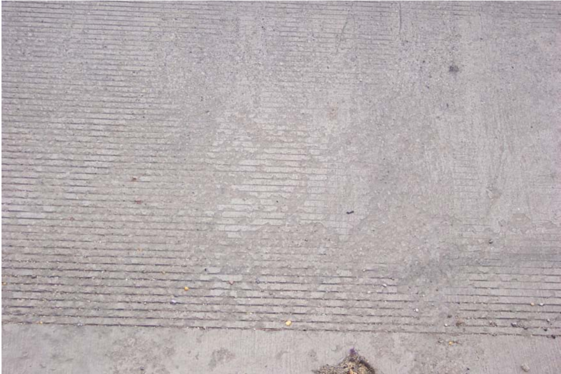
Figure 8. Euclid bridge, eastbound gutter driving lane (note scaling in the tined deck)
