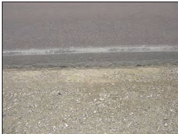
(a) Delaminated strip near pavement edge
