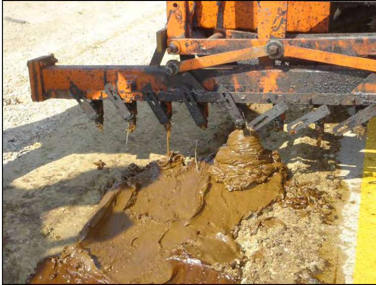
Figure 114. Distributor plugging after separation of emulsion and soybean oil, August 22, 2006
