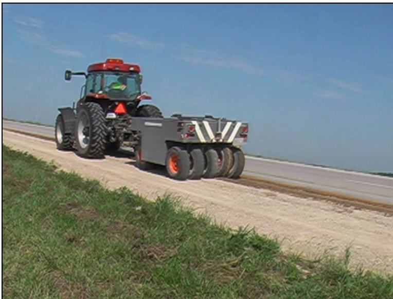
Figure 113. Compacting the stabilized section using a pneumatic roller on Hwy 18 milepost 202.50 Rudd, IA, on August 22, 2006
