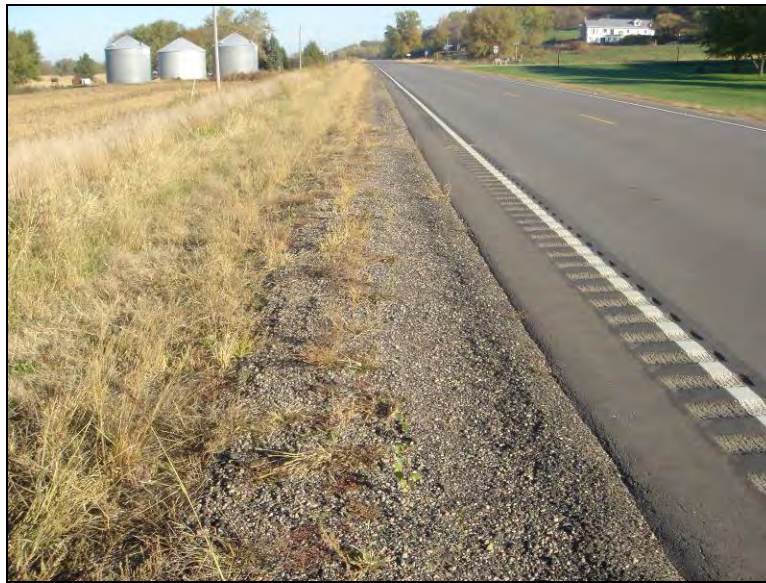
Figure 52. Granular shoulder section (southbound shoulder looking north) on Hwy IA 12 Station 1080+00', October 14, 2005
