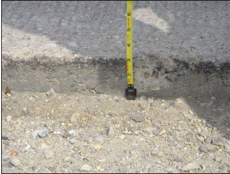
Figure 38. Shoulder edge drop-off on Hwy 65 exit ramp to Hwy 27, May 10 2006
