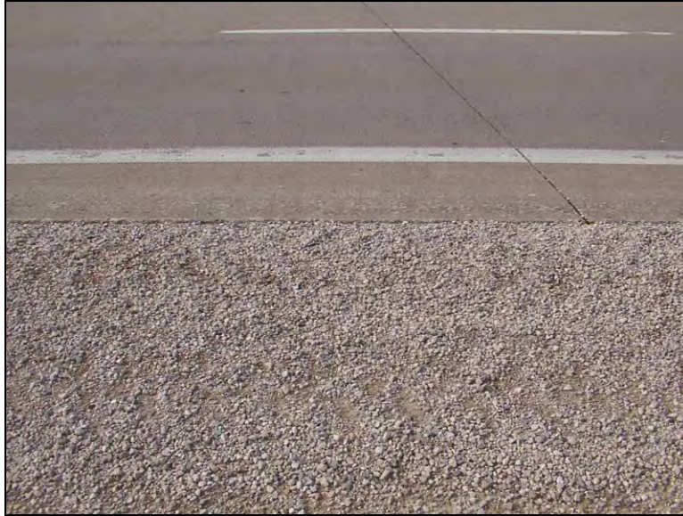
Figure 13. Granular shoulder section on U.S. 30 (milepost 156.0 W.B.), September 2, 2006
