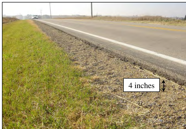
Figure 9. Shoulder drop-off along the shoulder section of Hwy 164, October 27, 2005
