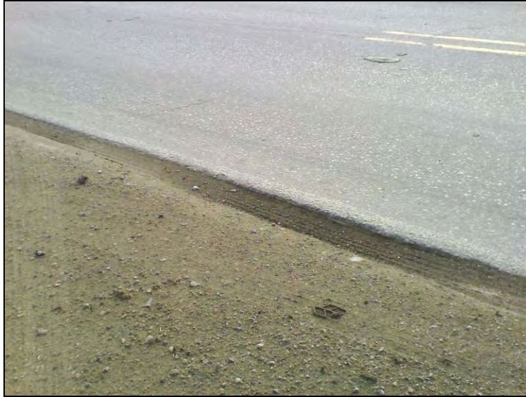
Figure 131. Three-inch edge drop-off adjacent to pavement after eight months, May 18, 2007
