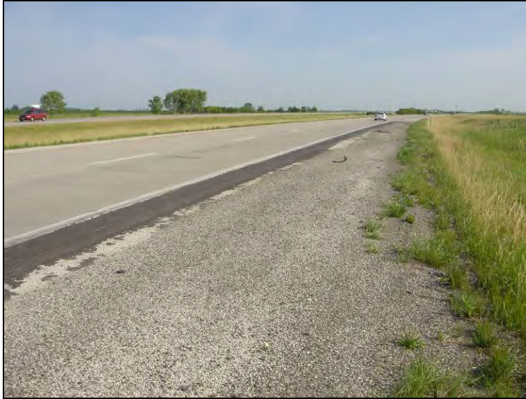
Figure 103. Asphalt patch placed on the deteriorated shoulder adjacent to a horizontal curve, I-35 milepost 150 northbound, July 7, 2006
