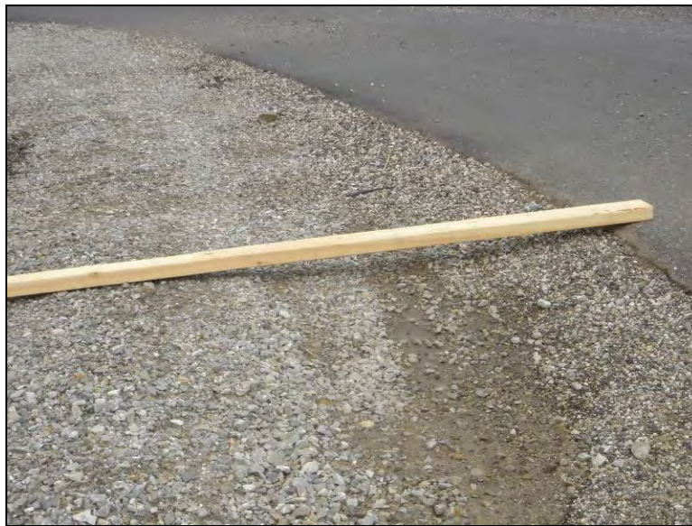
Figure 44. Cross slope damage at the intersection with Larke Ave. on Hwy 122, July 26, 2005
