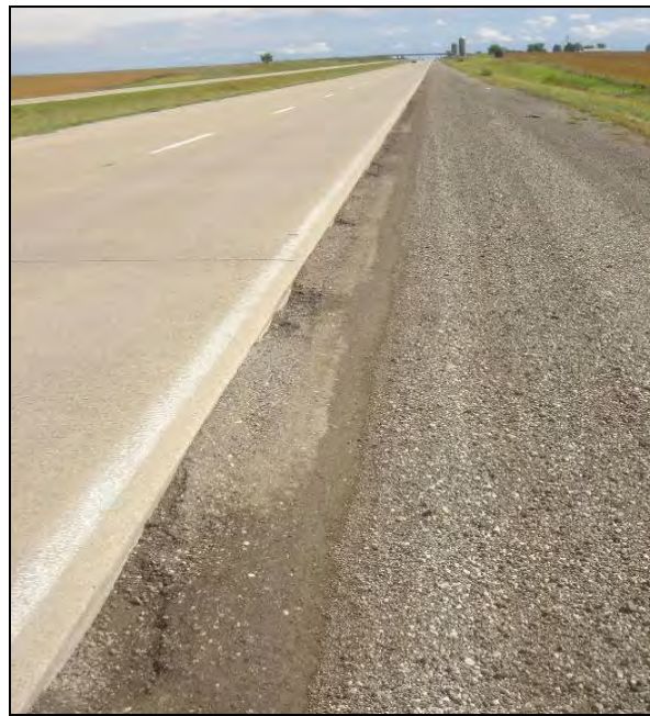
Figure 47. Granular shoulder section maintained with asphalt millings on Hwy 20 milepost 242 E.B., September 23, 2006
