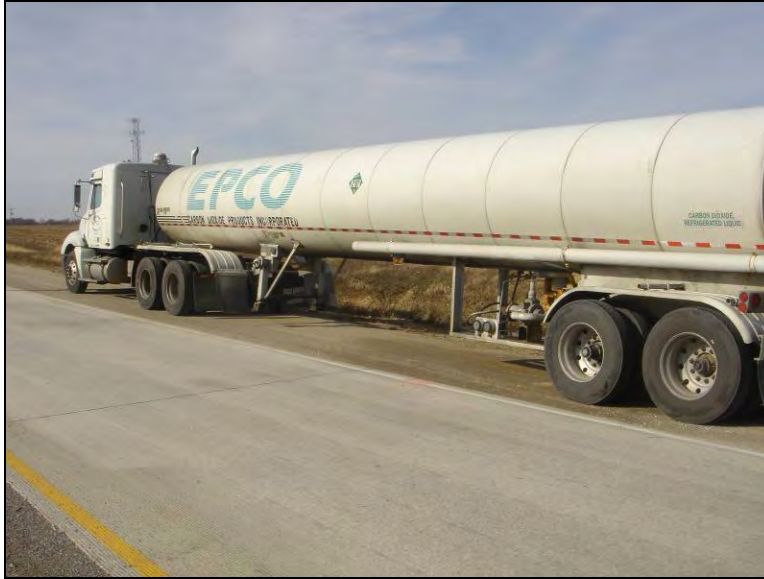
Figure 160. Stabilized shoulder along the exit ramp showing no rut under heavy traffic load, June 8, 2006
