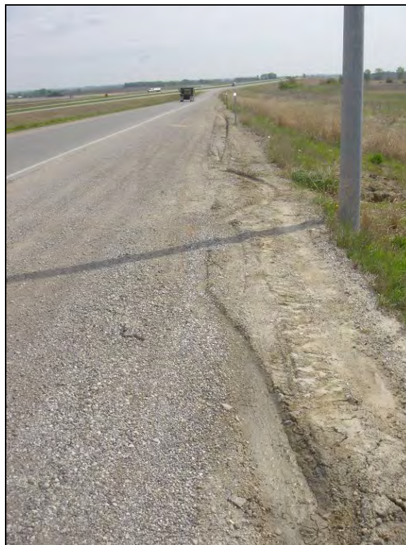
Figure 39. Shoulder rutting caused by soft subgrade and absence of granular layer on Hwy 65 exit ramp to Hwy 27, May 10, 2006
