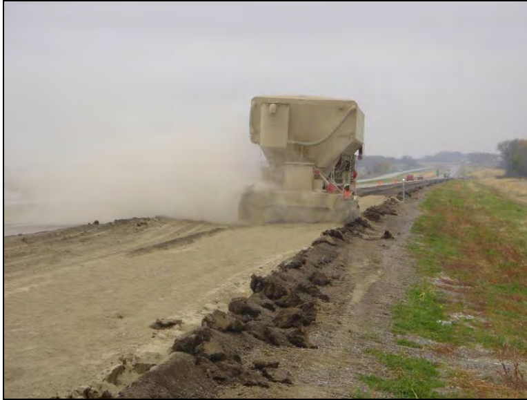
Figure 148. Semi trailer bottom dump truck spreading fly ash on top of subgrade layer, October 31, 2005
