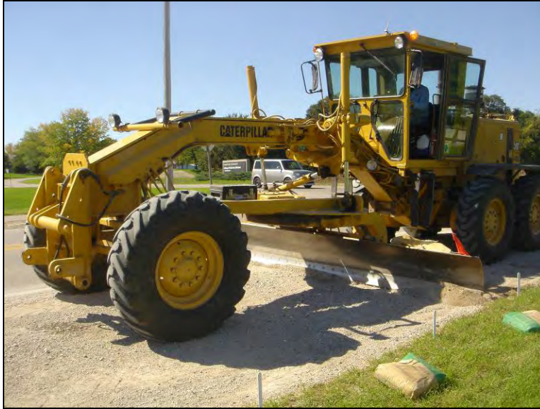
Figure 122. Blading of the shoulder section on 16th St. in Ames, IA, September 26, 2006
