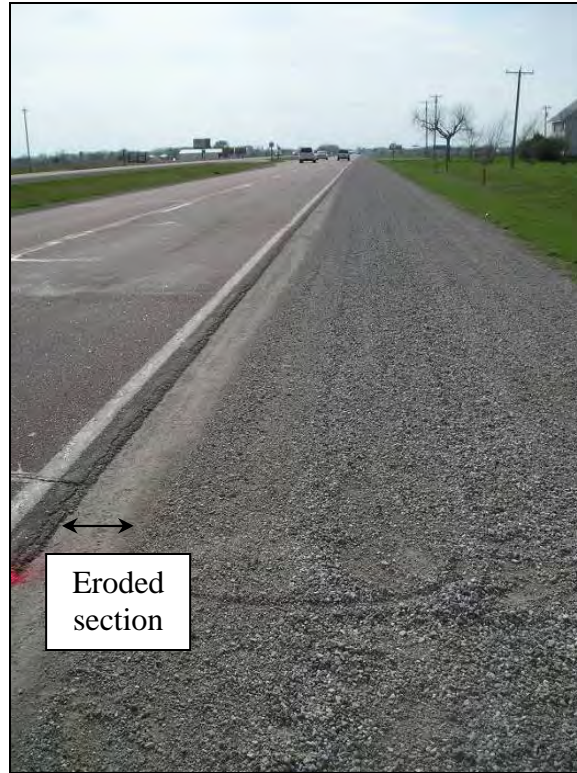
Figure 82. Erosion of the granular shoulder adjacent to the pavement edge on Hwy 122, April 18, 2005
