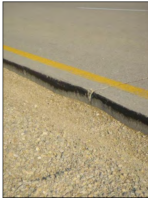
(b) Tire marks along pavement edge
