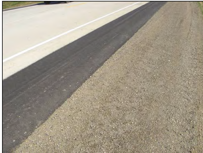
Figure 71. Shoulder section with 4 ft. of HMA and 4 ft. of blended limestone and crushed concrete on Hwy 60 St. 149+00', October 14, 2005
