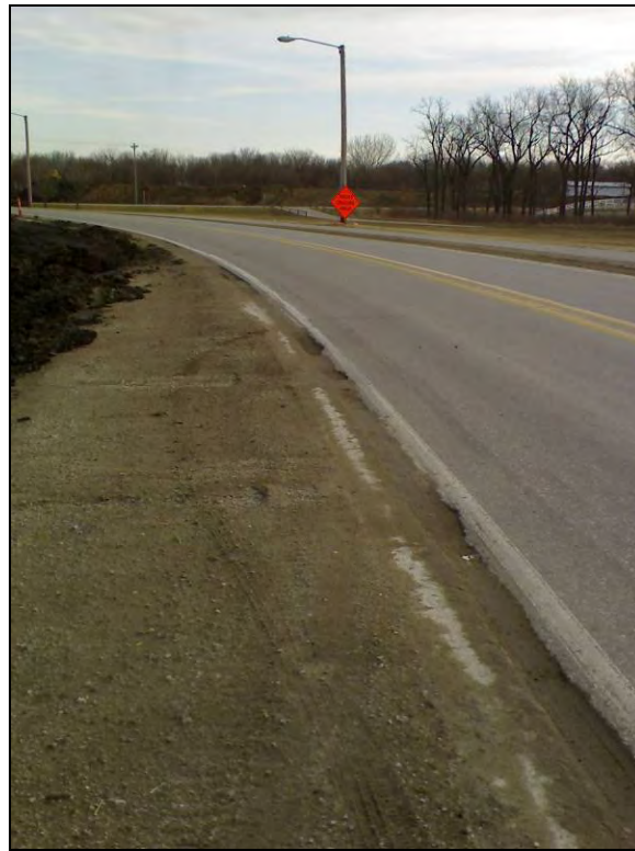
Figure 130. Significant edge drop-off observed after four months on 16th St. Ames, IA, December, 2007
