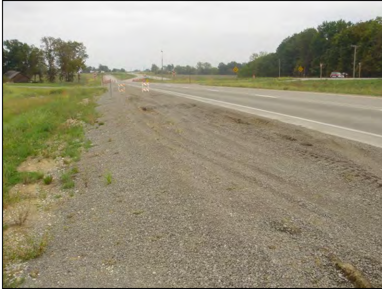
Figure 133. Severe rutting at the shoulder section, Milepost 207.8-90' Westbound, September 22, 2005
