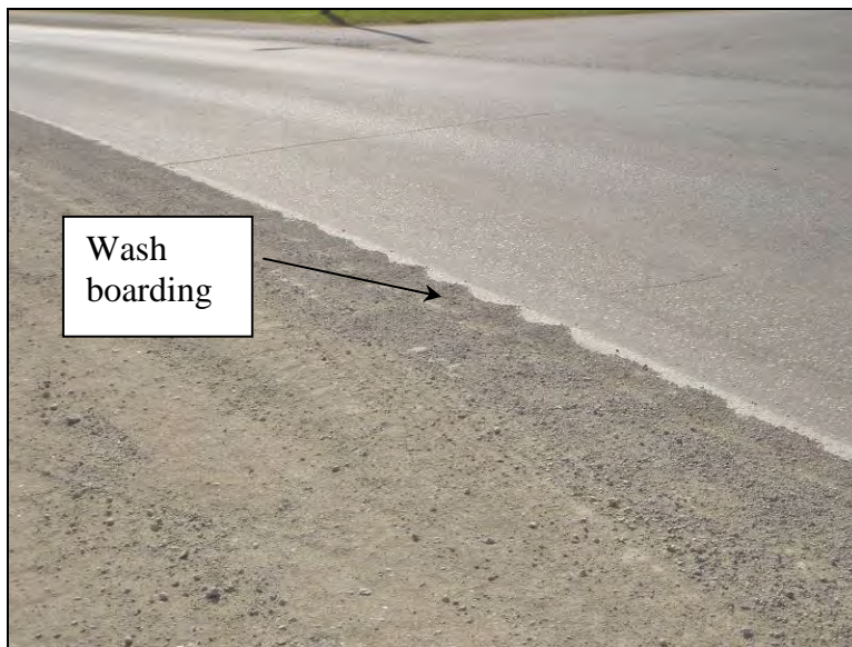
Figure 128. Development of wash boarding towards the end of the section (seven days after construction), October 3, 2006
