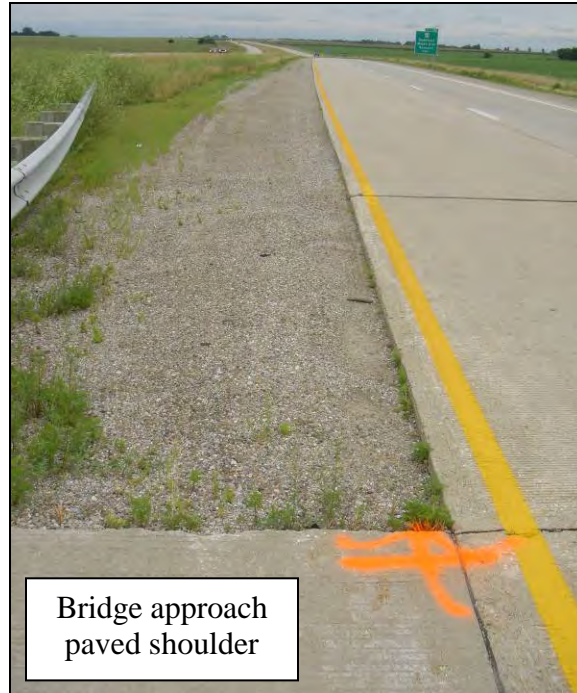
Figure 17. Granular shoulder section following a paved bridge approach shoulder, Hwy 18 milepost 184.55 E.B., July 26, 2005
