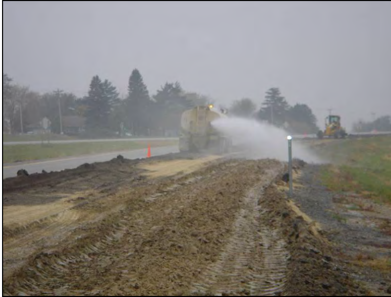
Figure 150. Water truck used to increase moisture content of clay-fly ash mixture, October 31, 2005
