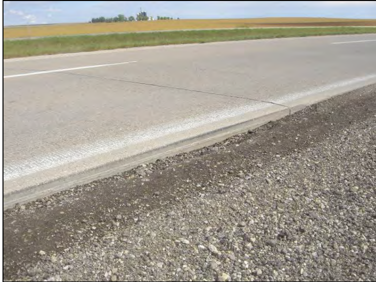
Figure 48. Four in. shoulder drop-off on Hwy 20 milepost 242 E.B., September 23, 2006
