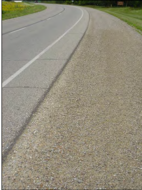
Figure 33. Granular shoulder section located on a super-elevated curve on Hwy 65 milepost 198.3 N.B., July 26, 2005
