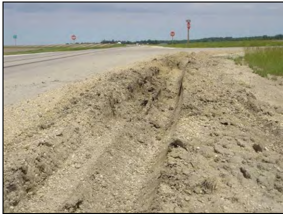
(a) Rutting extending to the underlying clay layer
