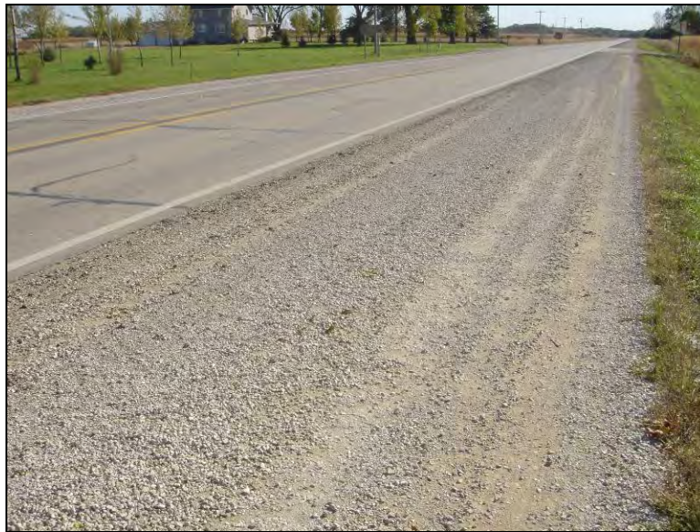
Figure 67. Granular shoulder section on Hwy 71 crossing Hwy 10 S.B., October 14, 2005
