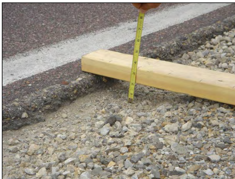
Figure 34. Shoulder drop-off adjacent to the pavement on Hwy 65 milepost 198.3 N.B., July 26, 2005
