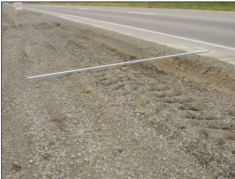
Figure 134. Closer image of the shoulder rutting shown in Figure 133, September 22, 2005
