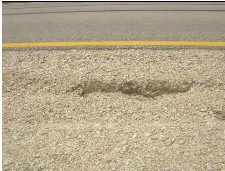
Figure 181. Development of shoulder rutting one month after shoulder construction, July 25, 2006
