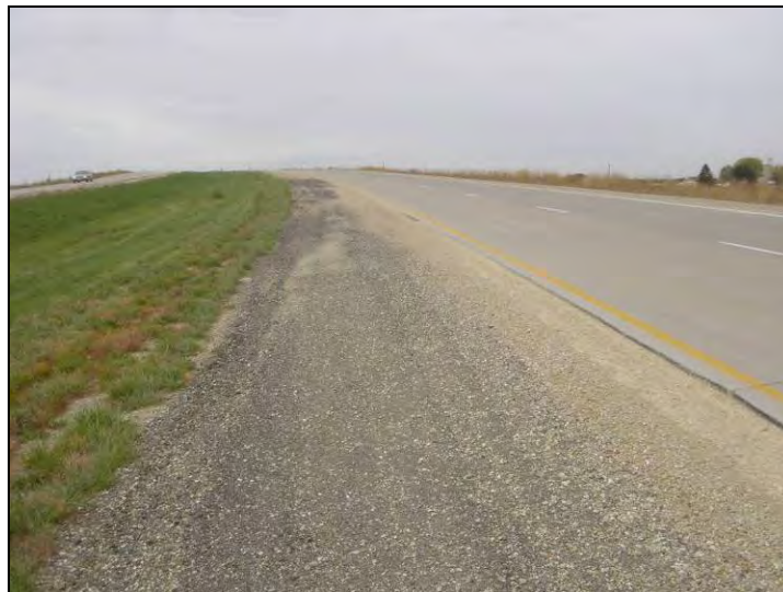
Figure 117. Asphalt millings placed at the shoulder test section and a 2 in. edge drop-off developed after two months, October 10, 2006
