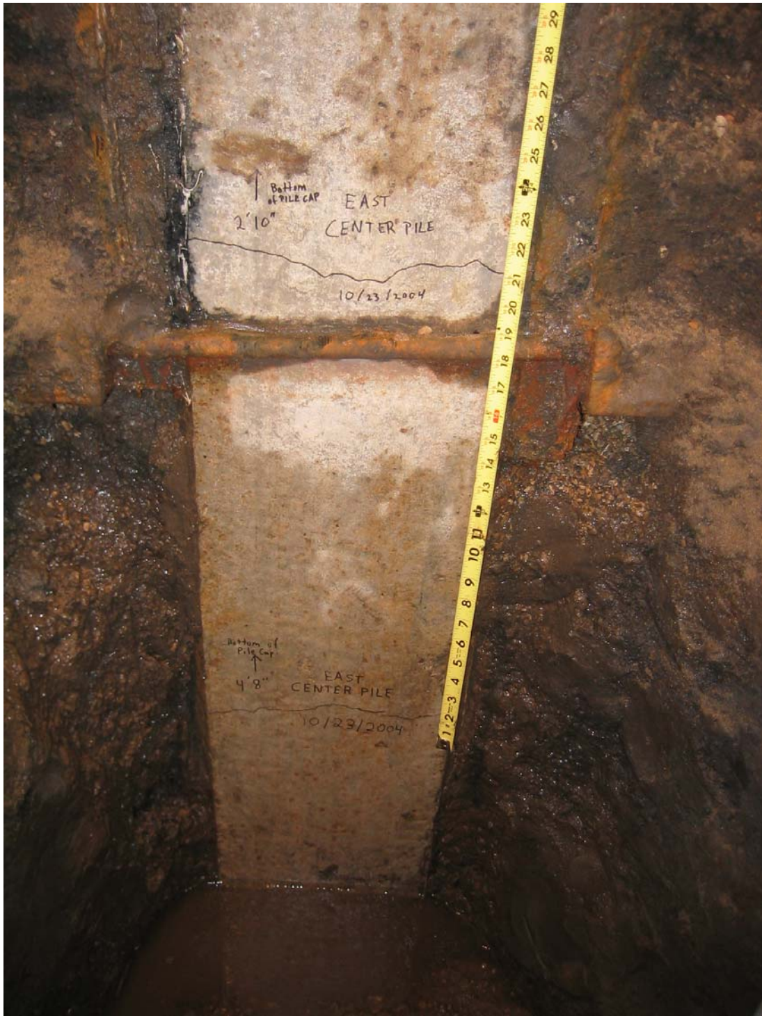
Figure 4.21. East abutment center pile excavated for crack exploration
