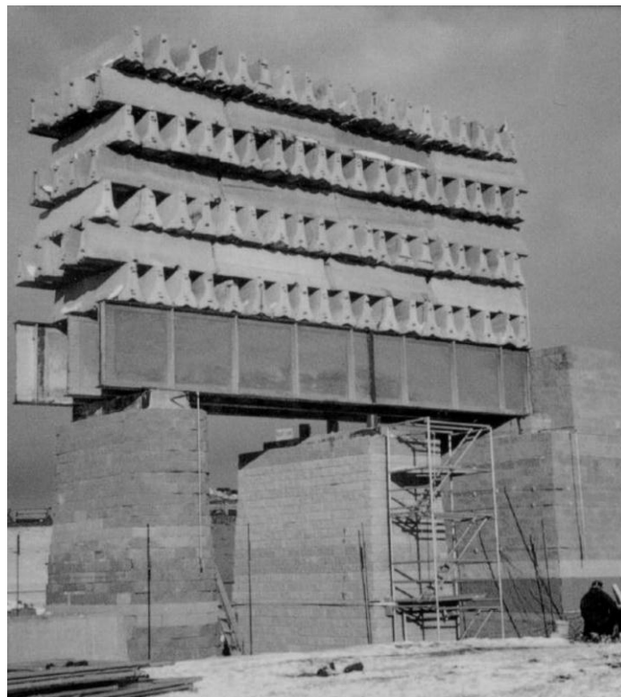
Figure 2-7. Full-scale GRS bridge abutment and two bridge piers (Abu-Hejleh et al., 2001b)
