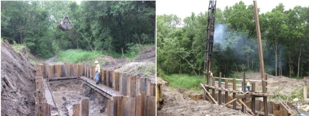
a.) Cofferdam placement and excavation b.) Placement and driving of battered piles
