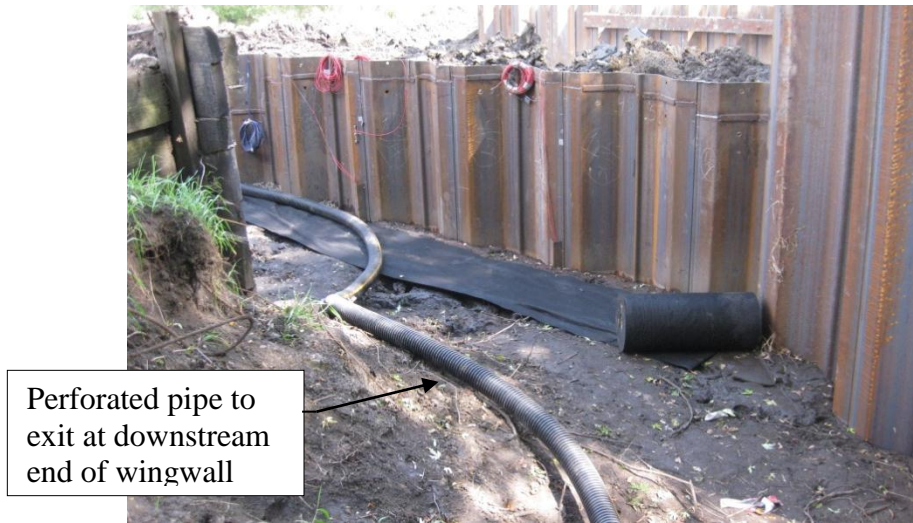
Figure 5-18. Drain tile installation on backfill side of west abutment in BHC, Iowa
