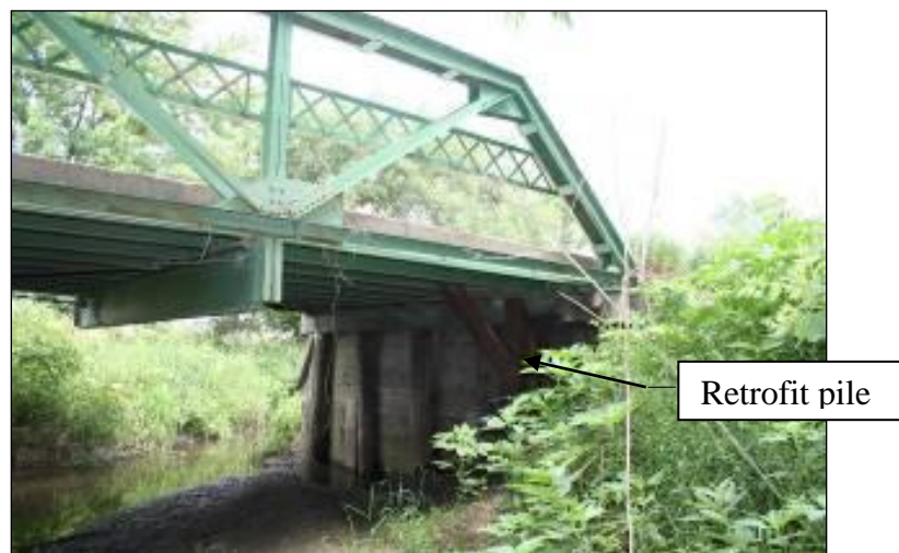
Figure 5-2. Previous bridge structure at demonstration project site in BHC, Iowa with retrofit pile
