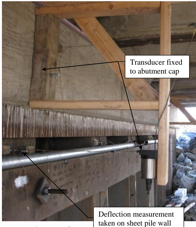
Figure 5-39. Instrumentation setup for measuring displacement of abutment cap relative to sheet pile wall (Disp 003)
