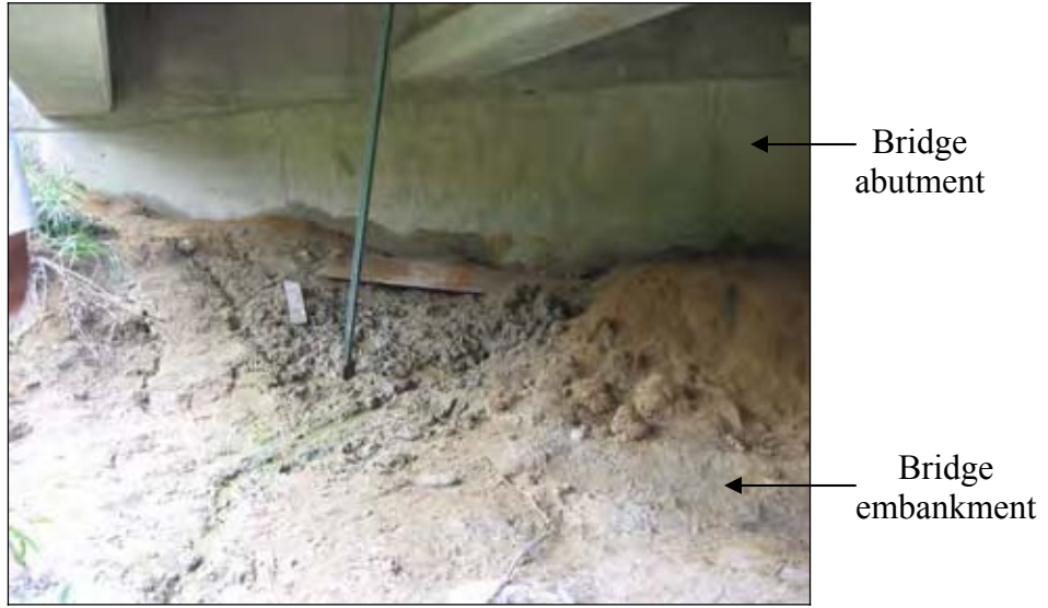
Figure 172. Soil erosion of the embankment under the bridge
