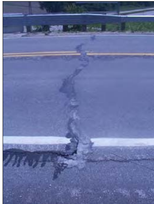
Figure 48. Transverse cracks of asphalt overlay (East end)
