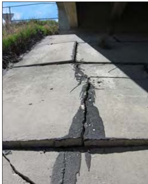
Figure 77. Fractured concrete slope protection
