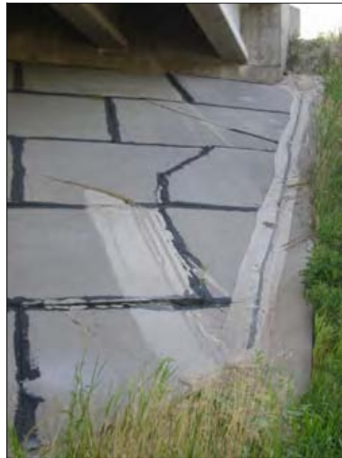
Figure 169. Cracking of the concrete slope protection overlay
