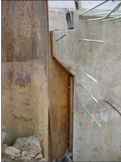
Figure 234. Declined paving notch
