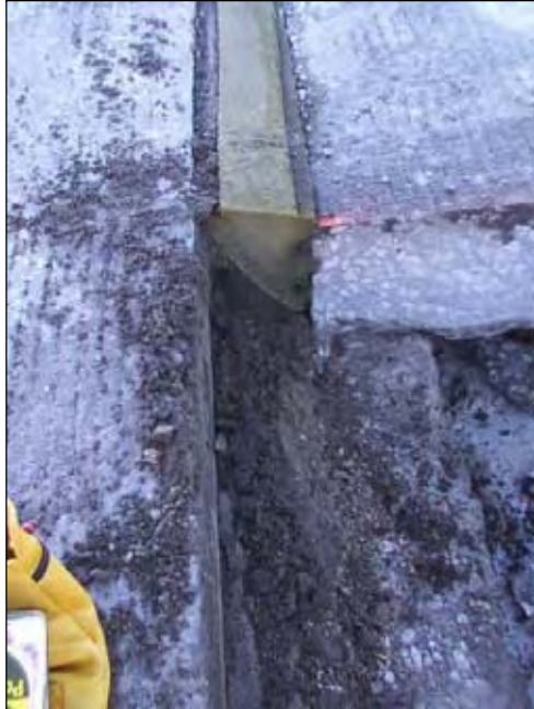
Figure 59. Contaminated expansion joint
