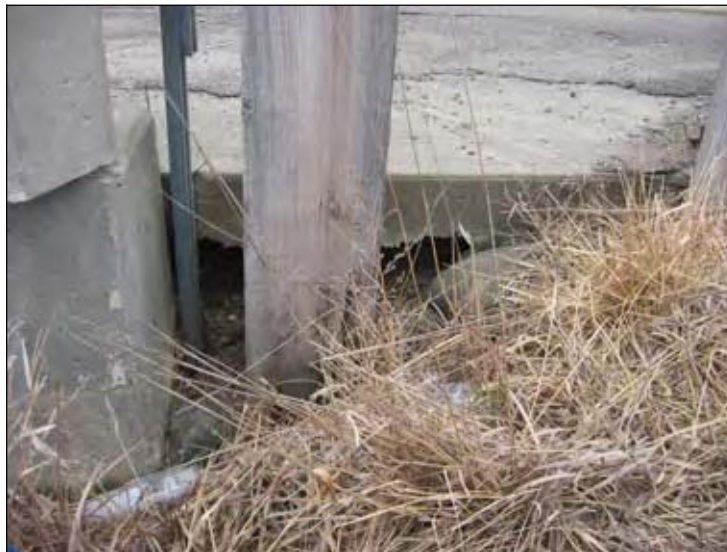
Figure A2. Void developed under approach slab
