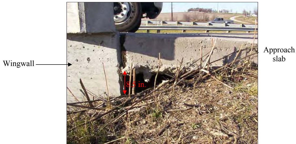
Figure 239. Void under approach slab (North end of SBL)
