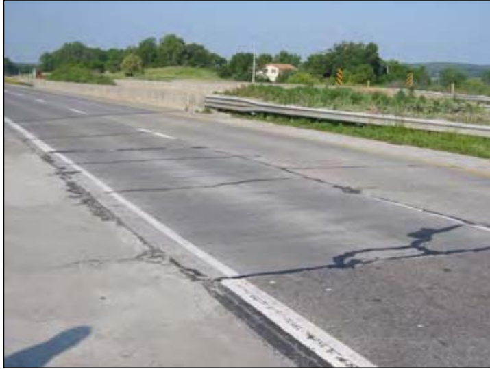
Figure 112. Cracking and settlement of recently replaced approach slab
