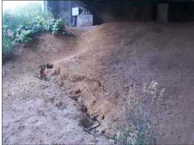
Figure 150. Erosion of the embankment under the bridge (North end of NBL)
