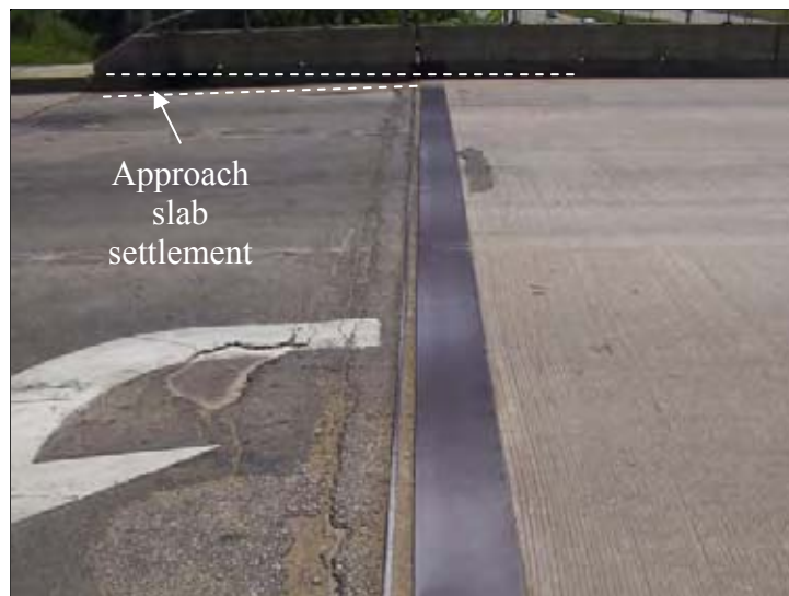
Figure 208. Cracks at asphalt approach with visible differential settlement
