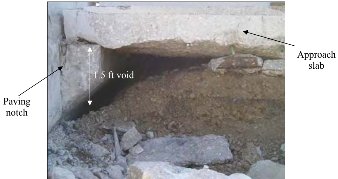
Figure 294. A void developed under the left lane approach slab which was 1.5-foot-deep at the bridge abutment (South end of SBL)
