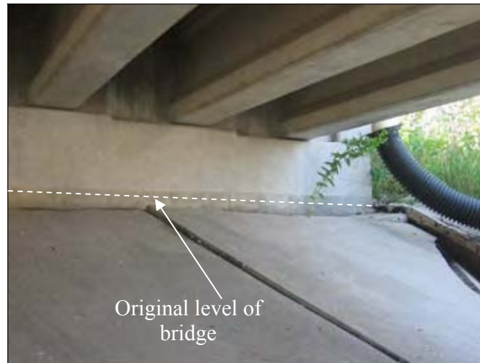
Figure 123. Concrete cover settlement of 10.5 in.
