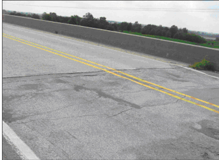
Figure 176. Transverse and map cracking at the approach slab
