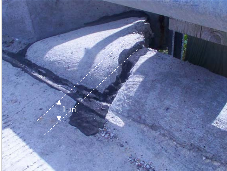
Figure 240. Differential settlement of 1 inch between the bridge slab and the bridge approach (South end of SBL)
