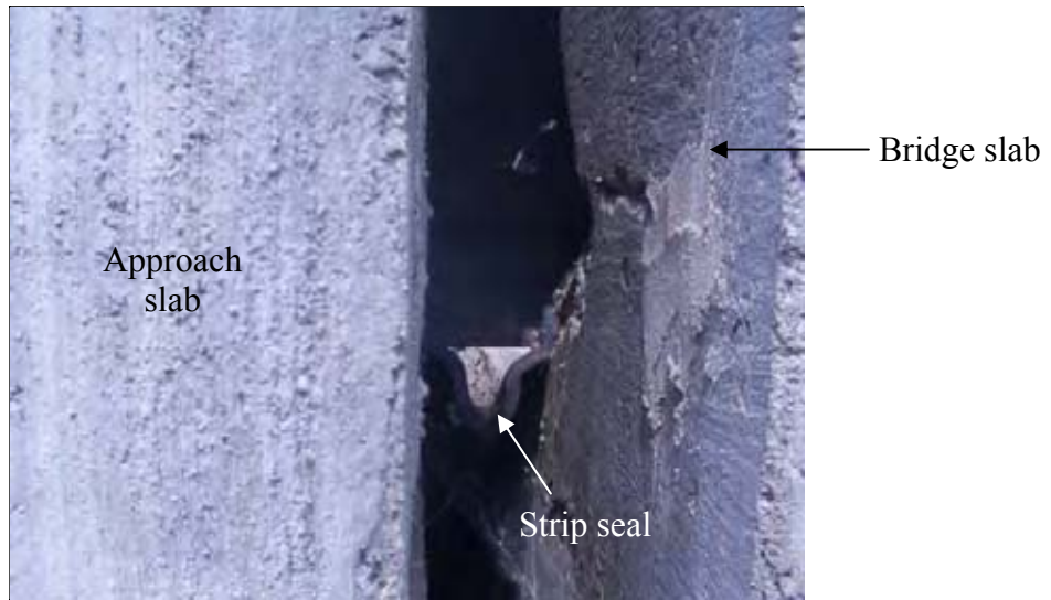
Figure 148. Side view of the strip seal which was cut short (South end of SBL)
