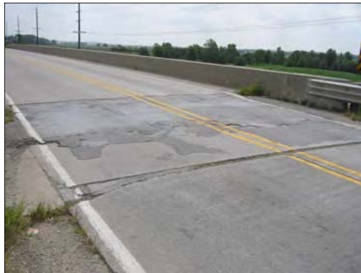
Figure 177. Deterioration of asphalt overlay at bridge approach
