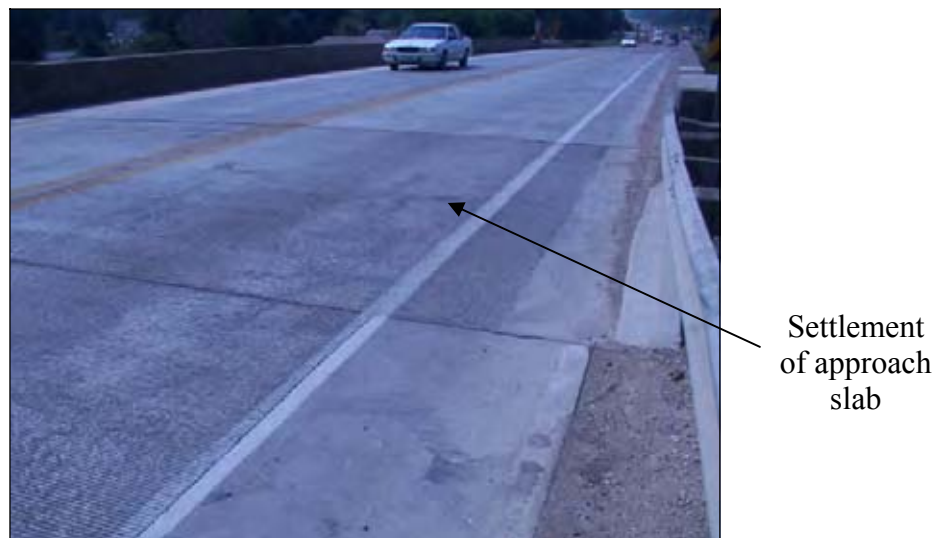
Figure 145. Differential settlement at recently replaced bridge approach
