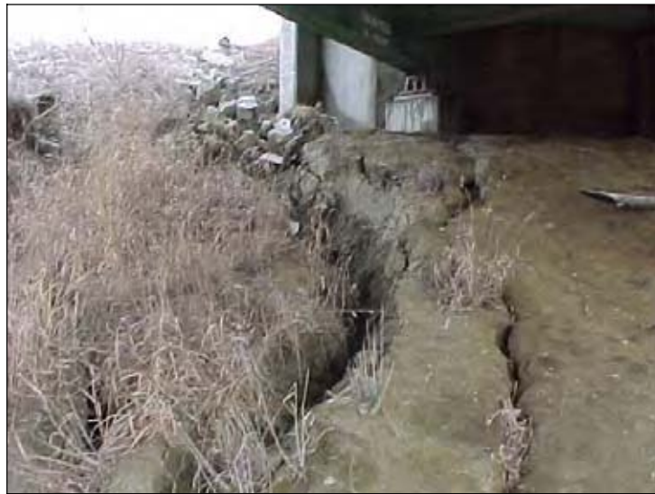
Figure 35. Soil erosion of the embankment under the bridge
