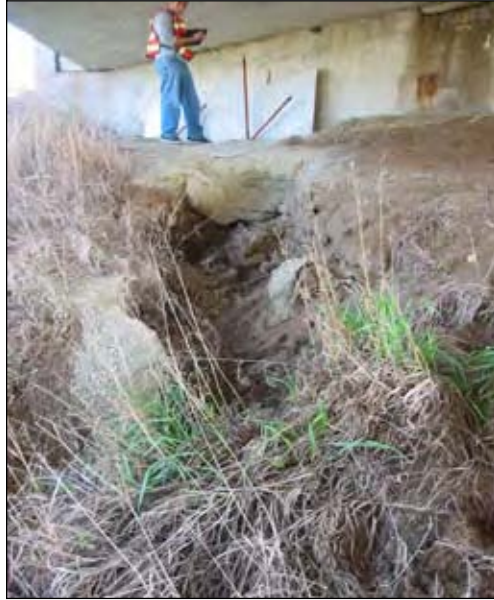
Figure 63. Erosion of the embankment soil under the bridge
