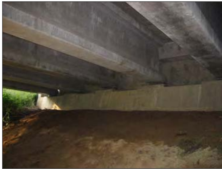
Figure 160. Wet loess soil observed at the embankment under the bridge
