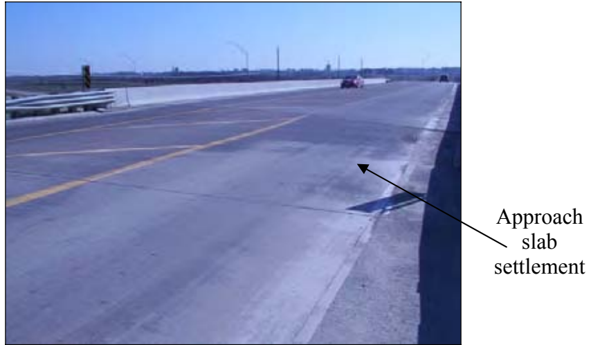
Figure 137. Settlement of approach slab
