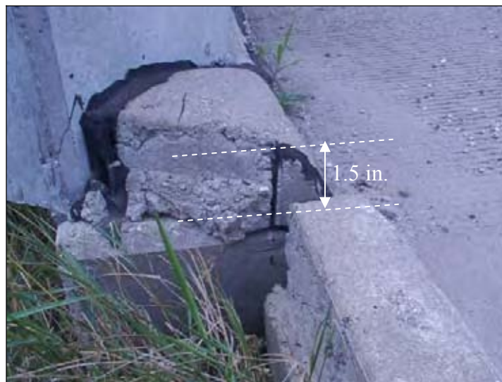
Figure 287. Differential settlement between the bridge slab and the bridge approach (North end of NBL)
