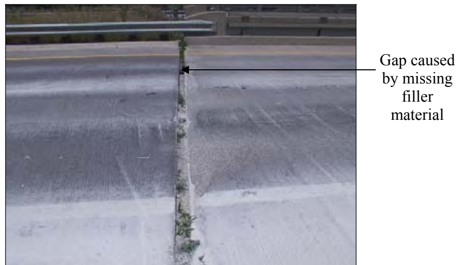
Figure 134. Expansion joint poorly sealed and filled with fines (West end of EBL)
