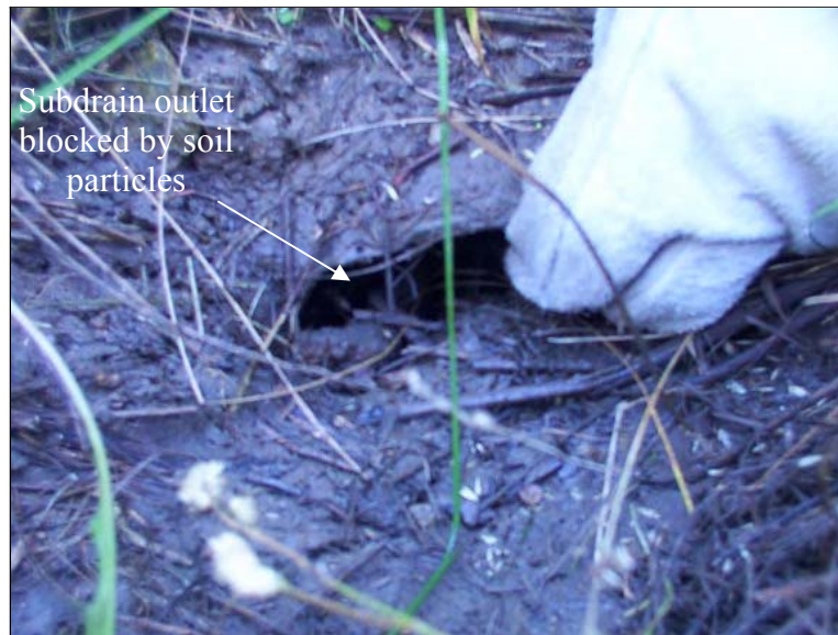
Figure 306. Subdrain outlet, located at the bottom of the embankment, blocked by soil debris
