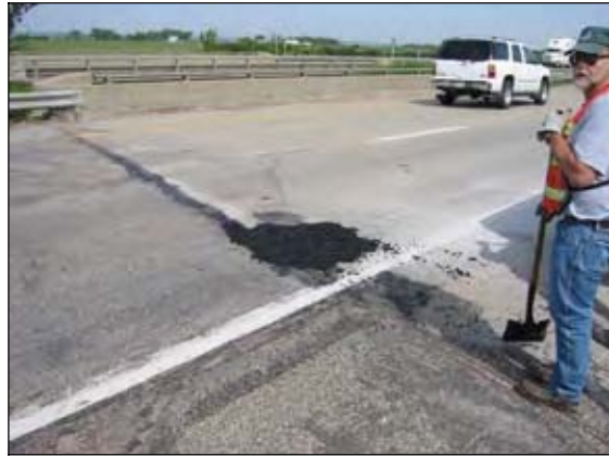
(b) Asphalt patch covering the cracks
