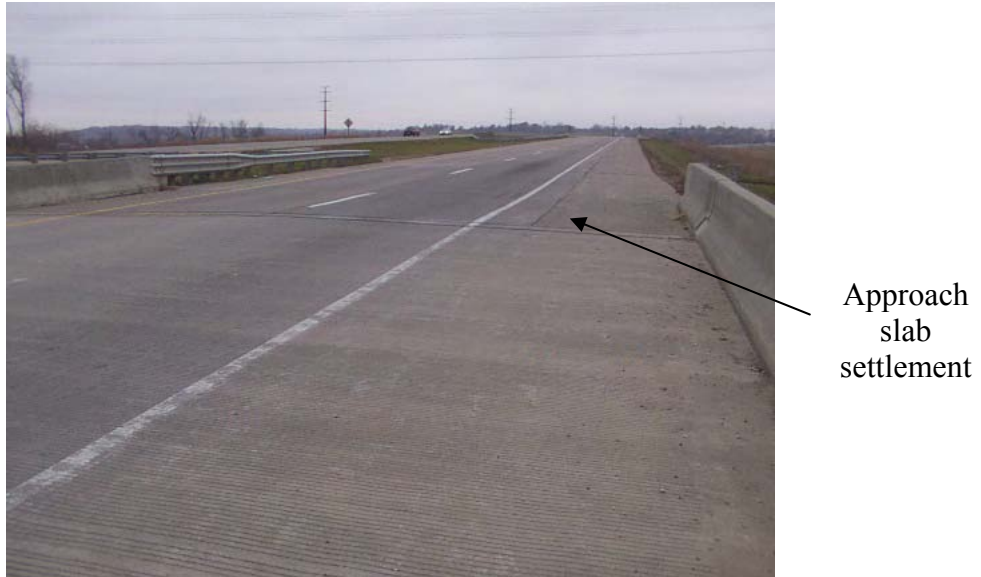
Figure 252. Settlement of approach slab (North end NBL)
