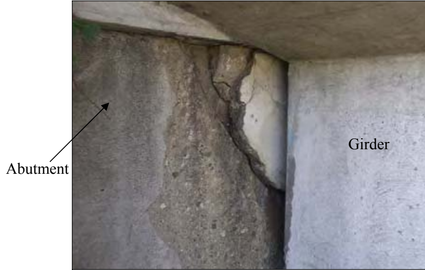
Figure 194. Concrete spalling at the abutment (SBL)
