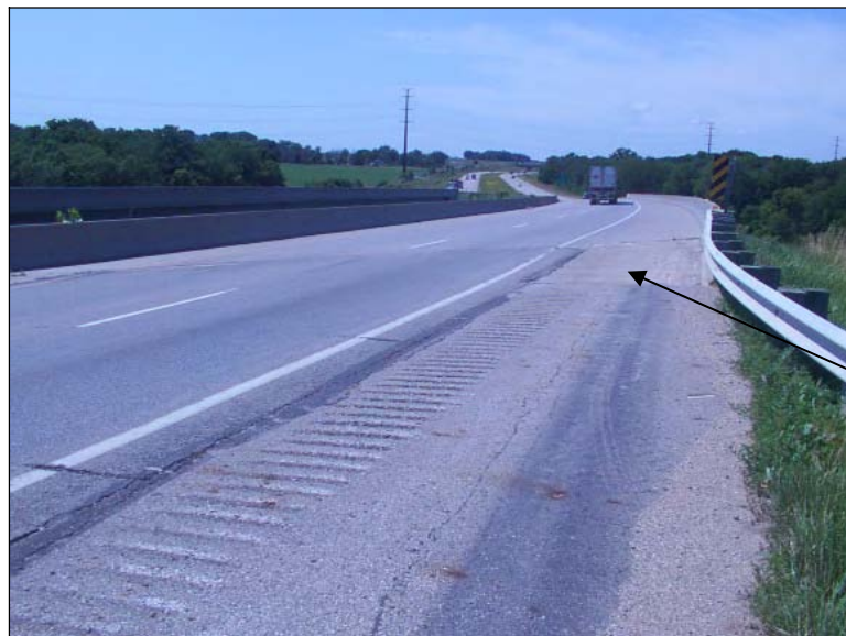
Figure 311. Settlement of bridge approach (South end of NBL)
