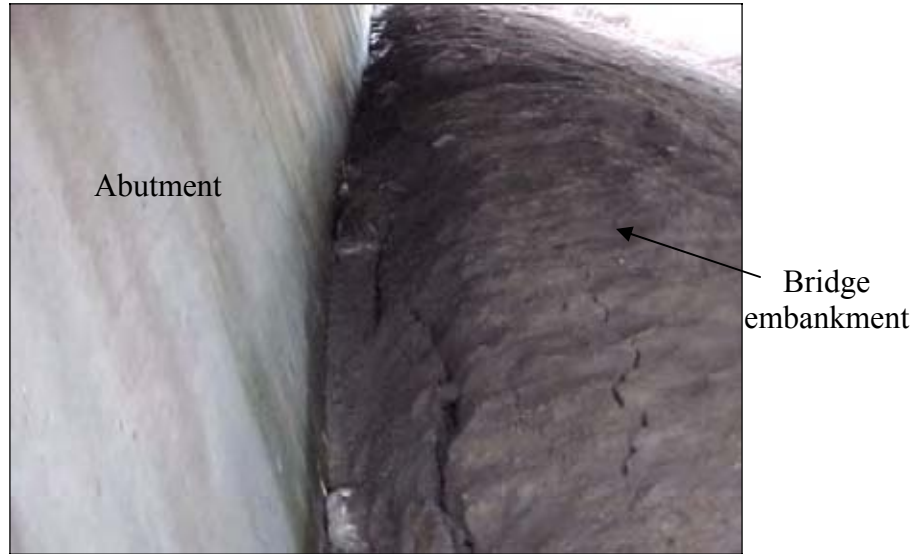
Figure 25. Erosion between abutment and embankment (North end of SBL)
