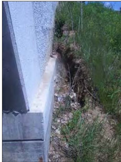
Figure 50. Soil erosion at the abutment side (West end)
