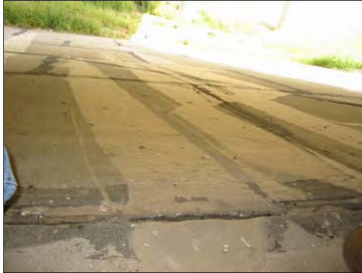
Figure 162. Grout seeping from under the concrete cover
