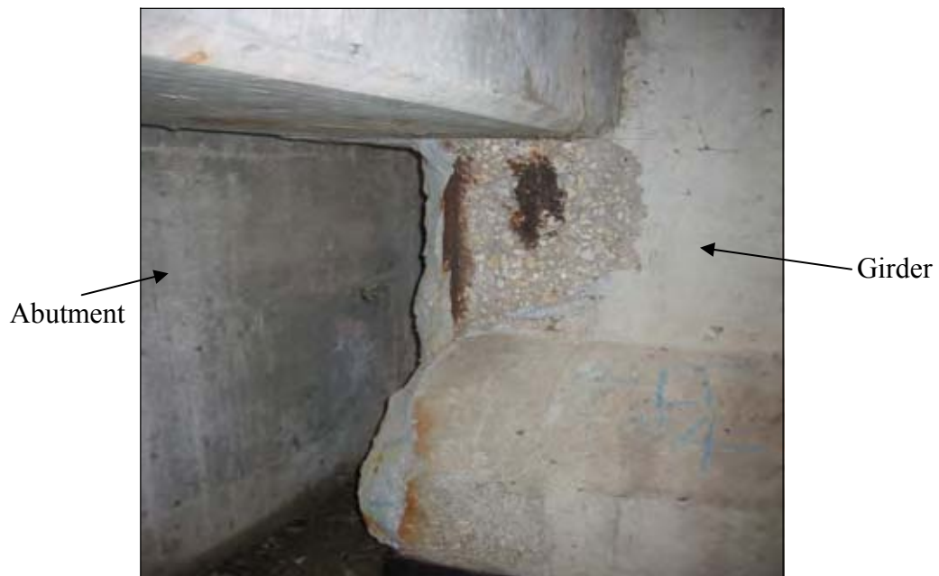
Figure 18. Deterioration of concrete with visible steel of the girders (South end NBL)
