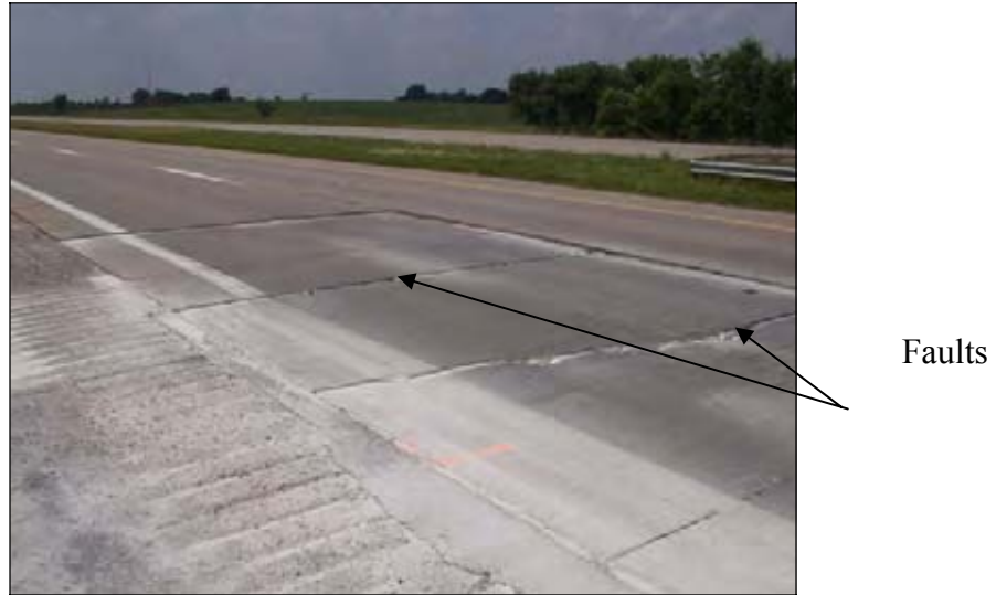
Figure 135. Faulting of bridge approach concrete panels (West end of EBL)
