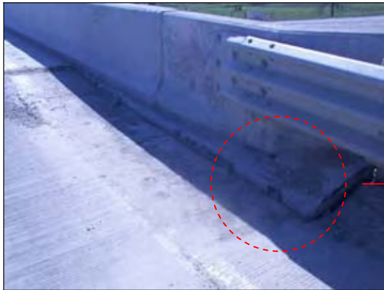
(a) Settlement of approach slab
