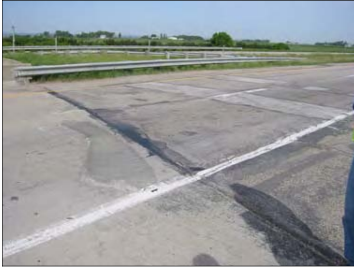
Figure 86. Significant damage of the asphalt overlay on the approach slab (NBL)
