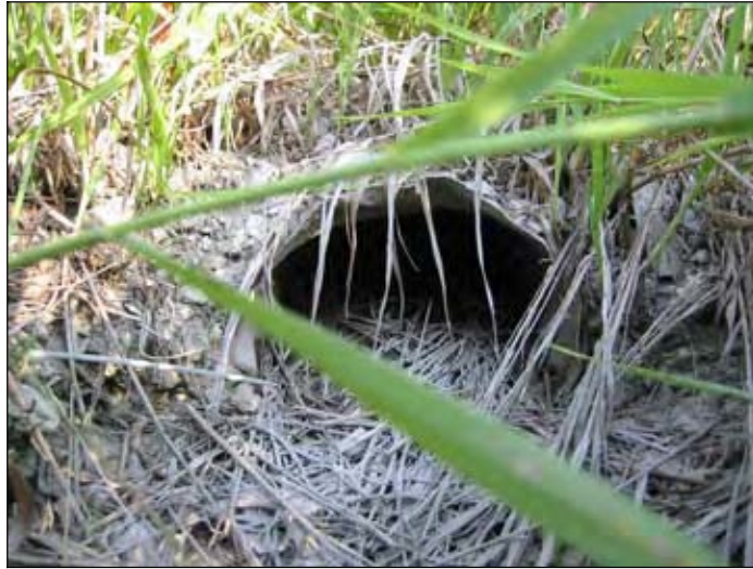
Figure 108. End drain plugged with soil
