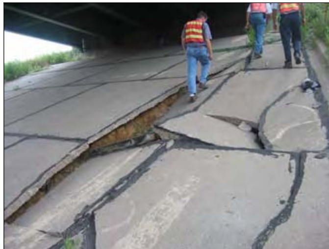
Figure 175. Severe damage of concrete slope protection due to erosion
