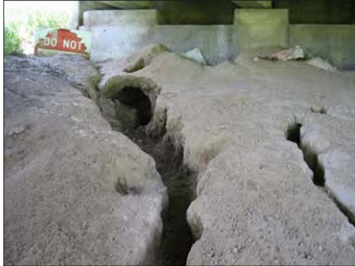
Figure 96. Severe erosion under the bridge
