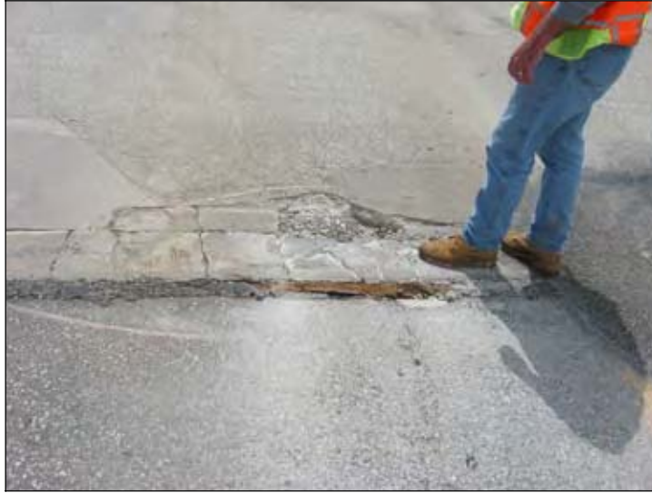
Figure 83. Cracks in the bridge deck concrete
