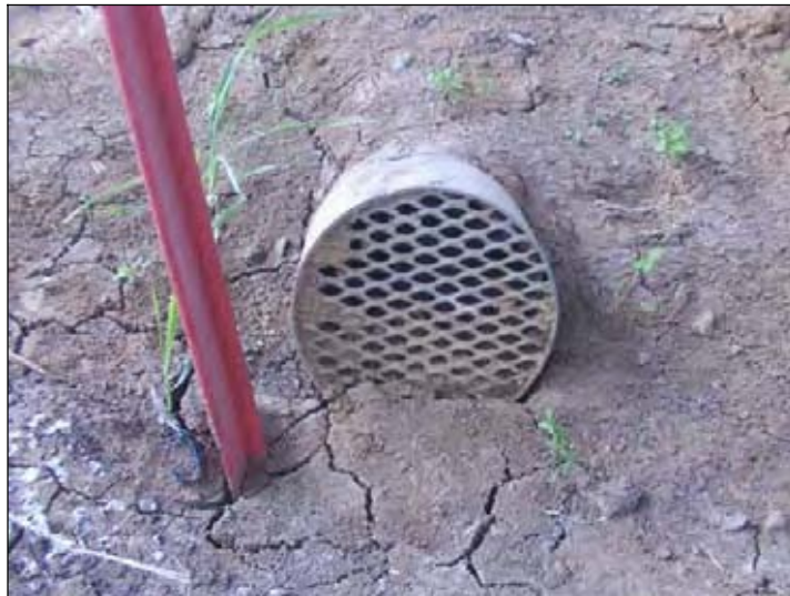
Figure 149. Perforated drain tile filled with soil (South end of SBL)
