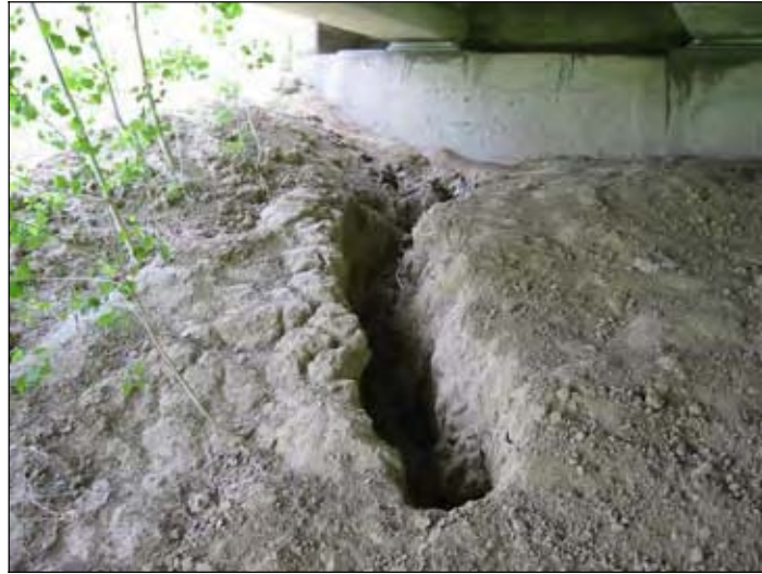
Figure 98. Soil erosion of the embankment under the bridge
