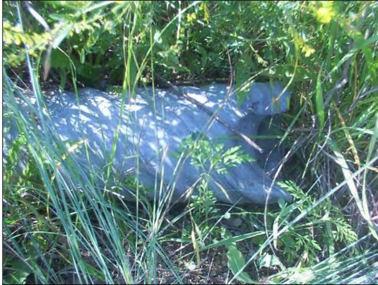
Figure 310. Damaged end drain (North end of NBL)
