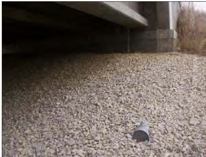
Figure 46. Aggregate used as a slope protection at the embankment under the bridge
