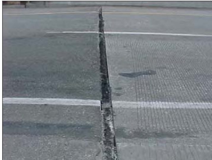
Figure 31. Poorly filled expansion joint with recycled tires used as a joint filler (North end SBL)
