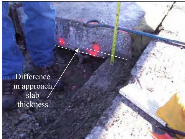
Figure 58. Non-uniform approach slab thickness with 1.5 in. increase over the backfill compared with the thickness over the paving notch
