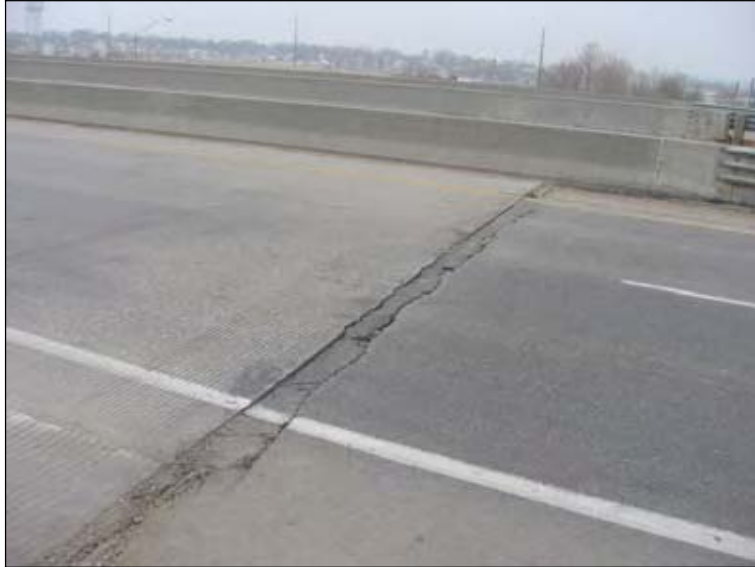
Figure A5. Cracks near the expansion joint
