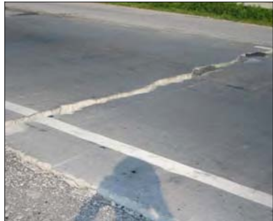
(b) Closer image of faulted approach slab
