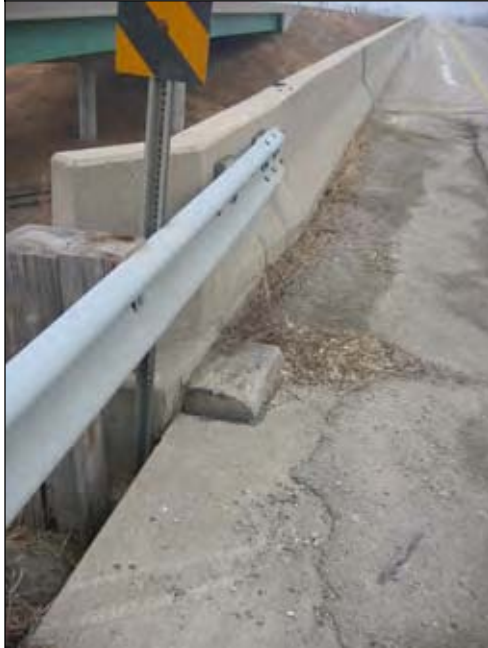
Figure A3. Differential settlement
