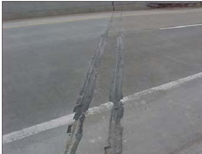
Figure 39. Deteriorated sealer at the expansion joint
