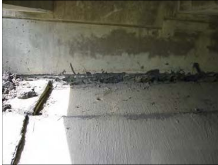
Figure 92. Uneven settlement of concrete slope protection
