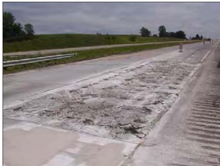
Figure 132. Approach pavement broken before replacement
