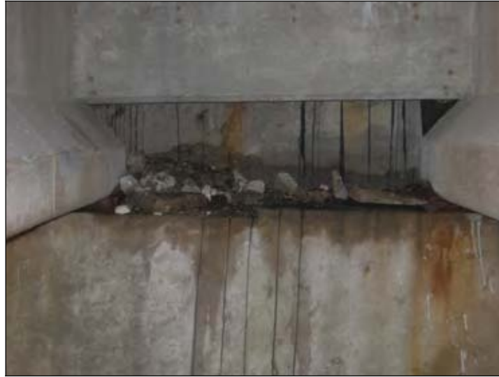
Figure A7. Water flowing down the bridge abutment
