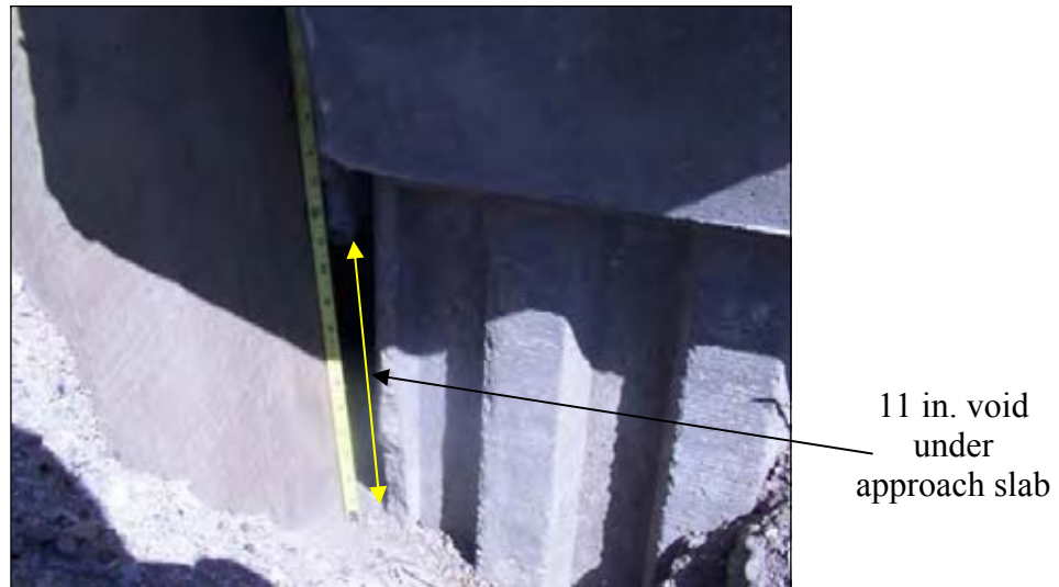
Figure 140. Void developed under the approach slab
