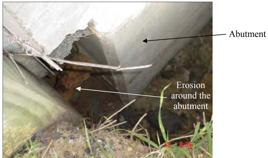
Figure 179. Soil erosion around the abutment
