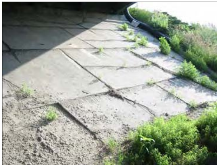
Figure 111. Cracking of concrete slope protection
