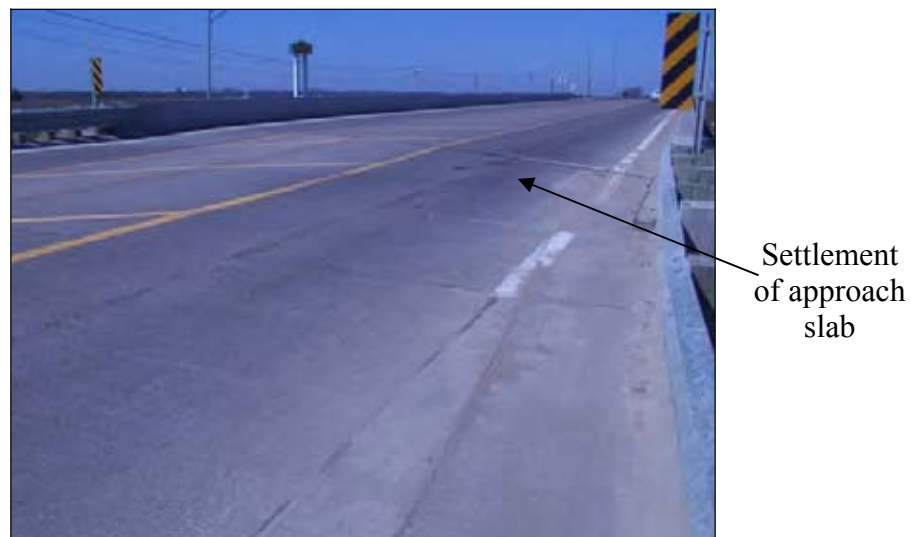
Figure 141. Differential settlement at the bridge approach (East end)
