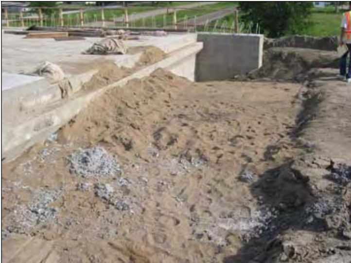
Figure 230. Poorly placed granular backfill
