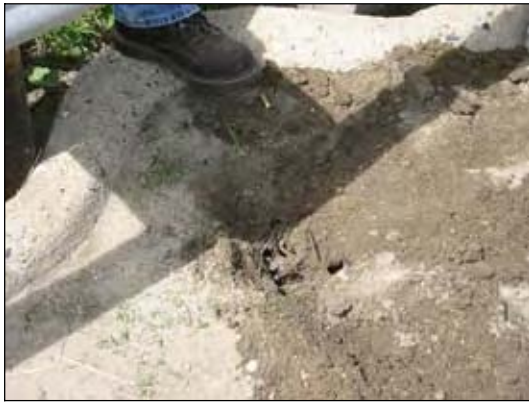
(a) Bridge approach surface drain blocked by debris
