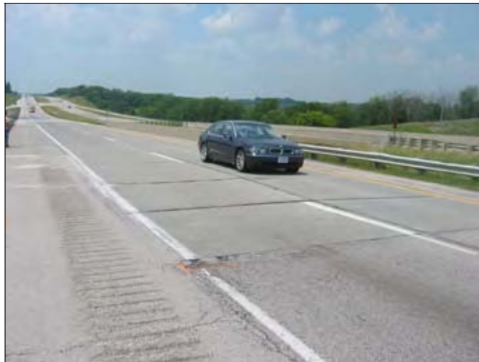
Figure 131. Damage of the approach slab section
