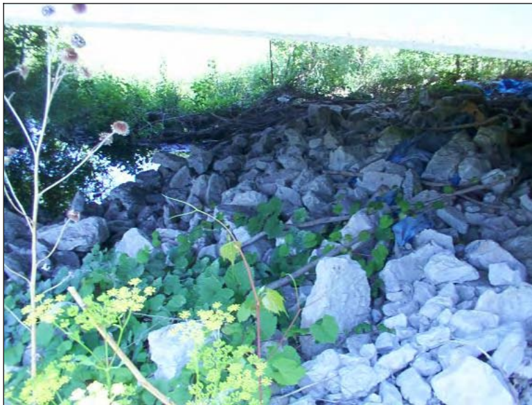
Figure 251. Rocks placed at the embankment under the bridge to prevent further erosion (South end of NBL)
