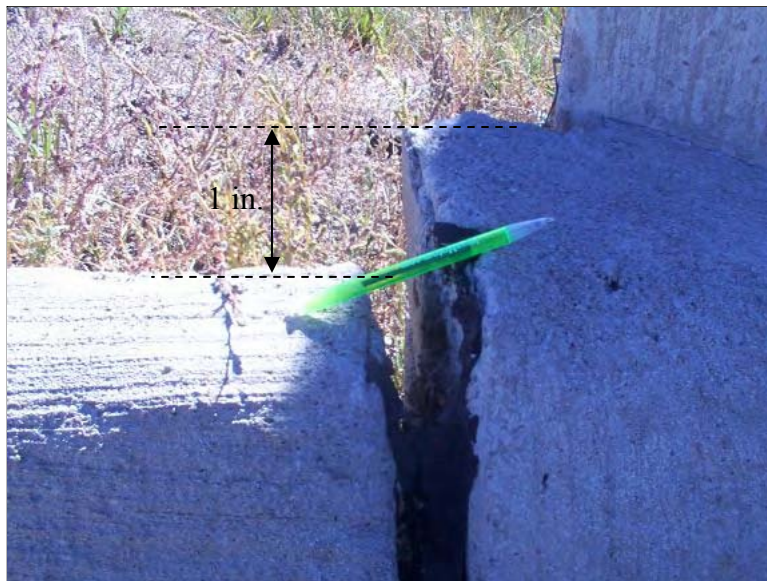
Figure 334. Differential settlement between the bridge approach and the approach slab (East end of EBL)
