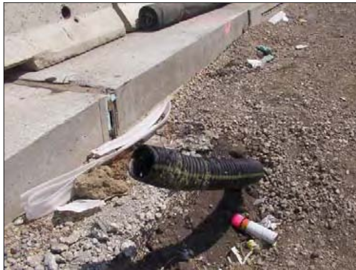
Figure 223. End drain outlet filled with soil
