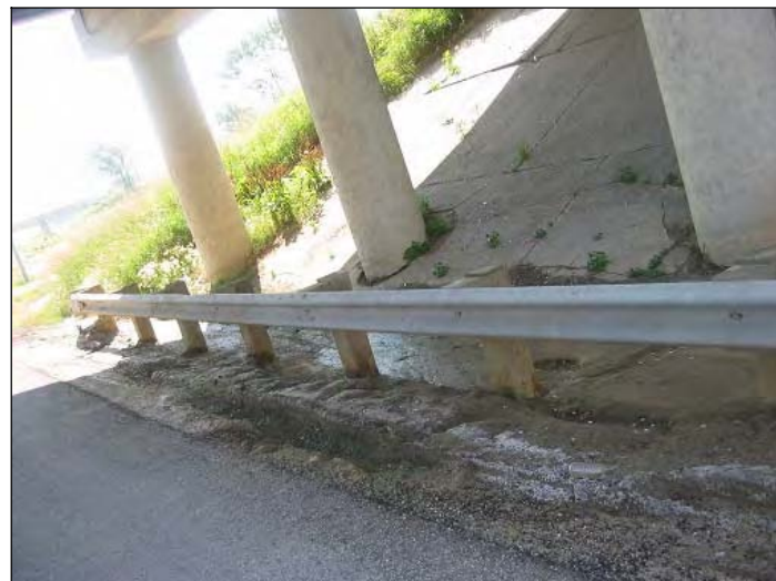
Figure 124. Ponding water and debris observed at the bottom of the embankment
