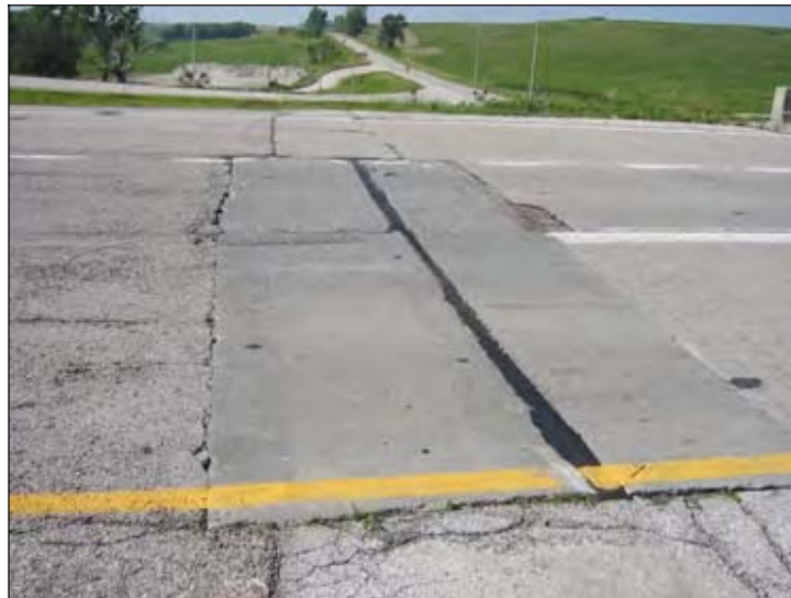
Figure 119. Various cracking at the bridge approach (EBL)
