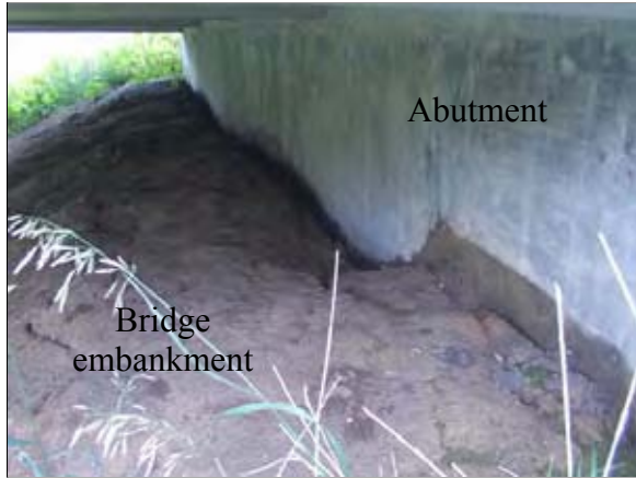
(a) Erosion at the abutment
