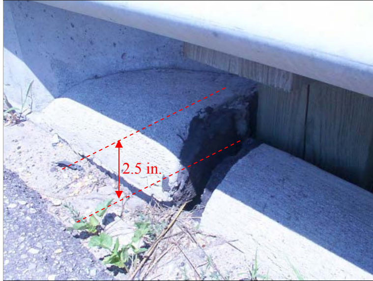
Figure 298. Differential settlement at the bridge approach (South end of NBL)
