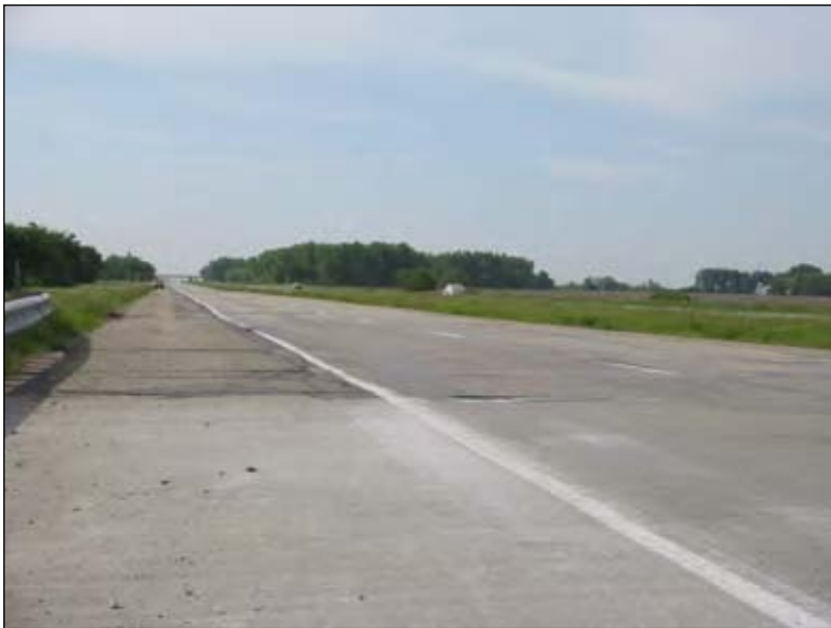
Figure 87. Wavy approach slab (NBL)
