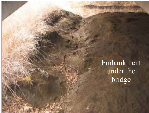
Figure 17. Soil erosion of the embankment under the bridge (South end of North bound)
