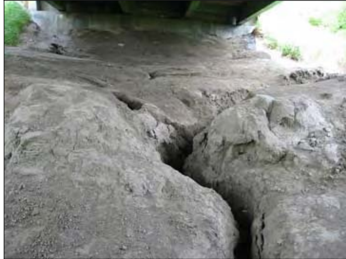
Figure 103. Soil erosion of the embankment under the bridge
