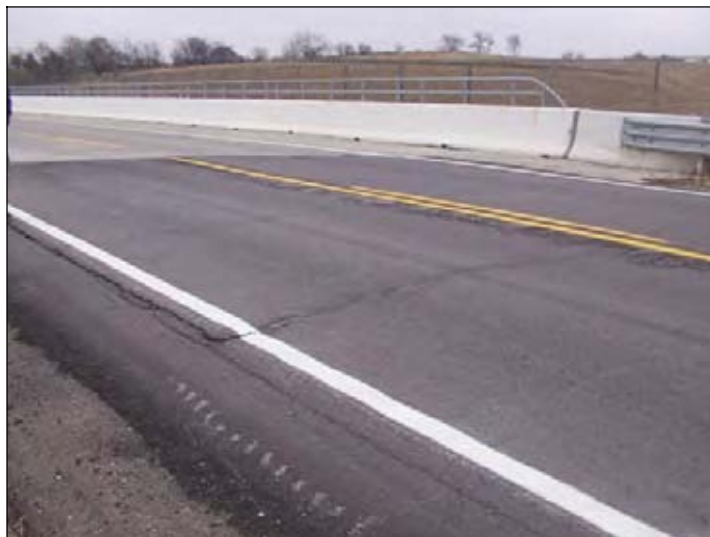
Figure 44. Cracking of the asphalt overlay (East end)
