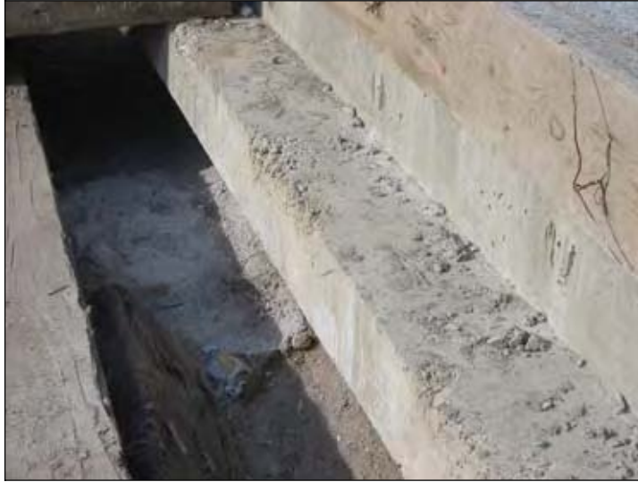
Figure 232. Poor construction of bridge paving notch
