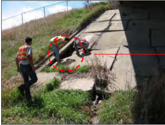
(a) Damaged slope protection
