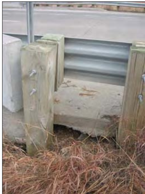
Figure A6. Void developed under the approach slab
