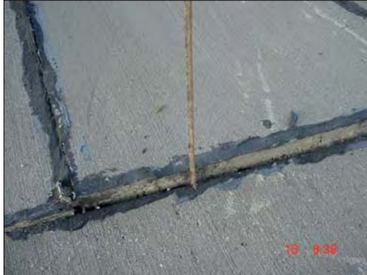
Figure 178. Uneven concrete slope protection
