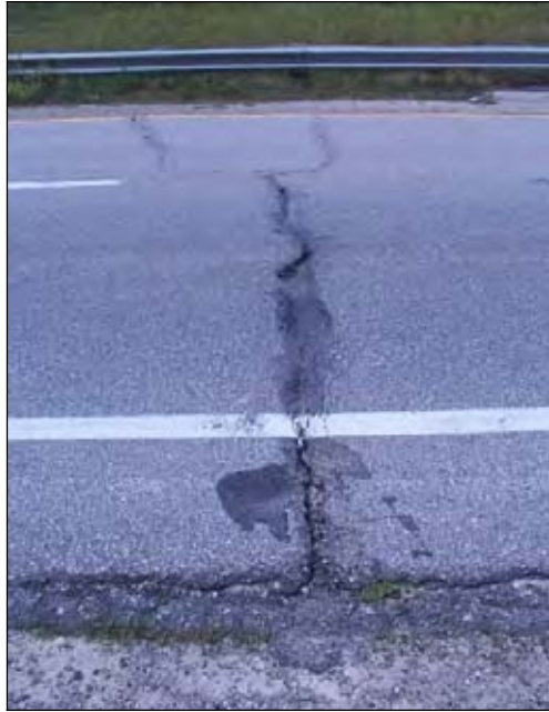
Figure 154. Transverse cracking of asphalt overlay (West end of WBL)
