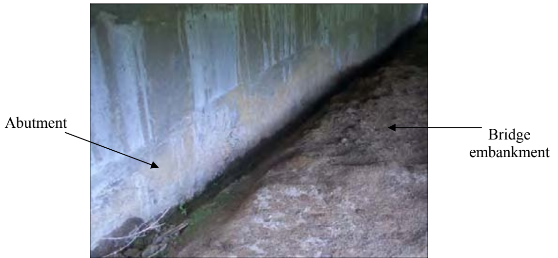
Figure 155. Erosion of the embankment soil (West end of WBL)
