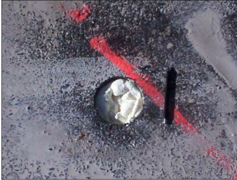
Figure 315. Expanding foam placed in the core hole of the approach slab (NBL)
