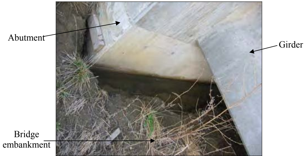
Figure 65. Ponding water at the abutment under the bridge
