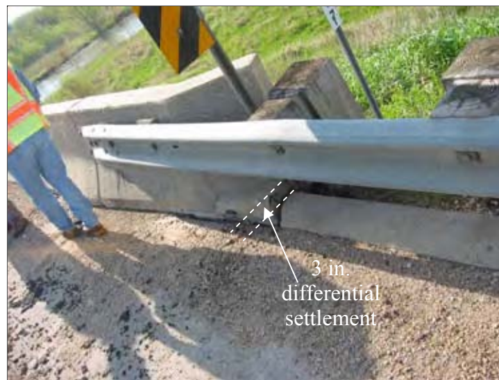
Figure 60. Differential settlement of 3 in. at the south-west corner
