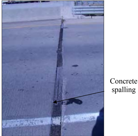
Figure 335. Poorly sealed expansion joint with concrete spalling (East end of EBL)
