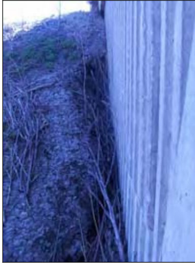
Figure 144. Erosion around the abutment (East end)
