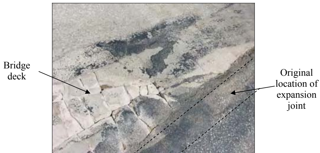
Figure 79. Breakage of bridge deck concrete
