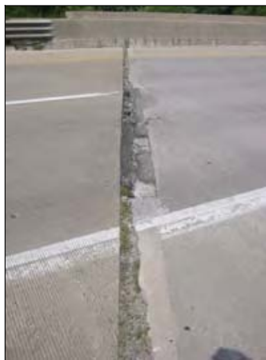
Figure 171. Concrete spalling and cracking at the expansion joint
