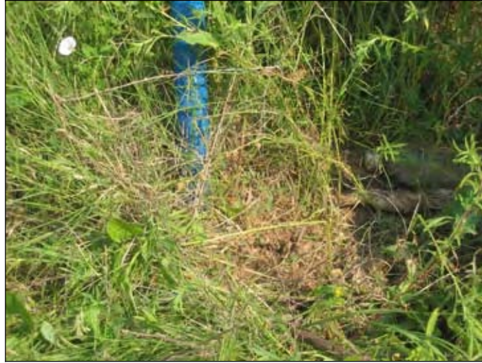
Figure 110. Drainage outlet could not be located
