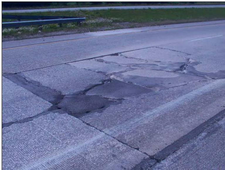
Figure 309. Severe cracking at the bridge approach pavement (North end of NBL)
