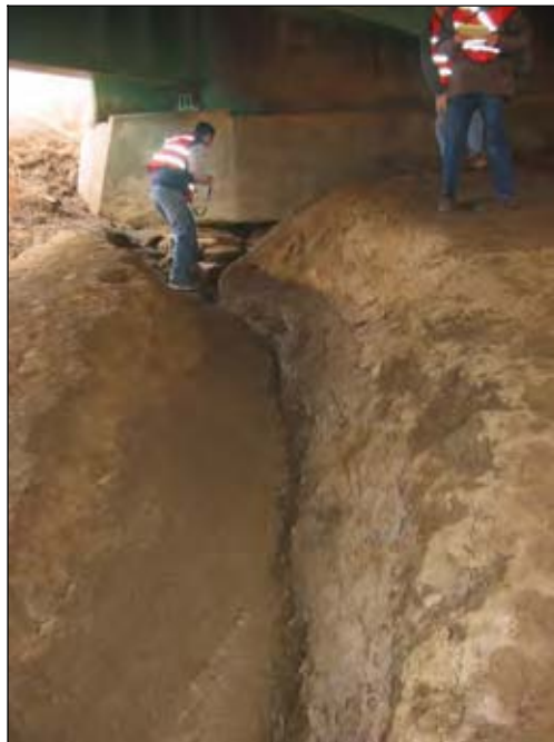
Figure A4. Soil erosion at the bridge embankment
