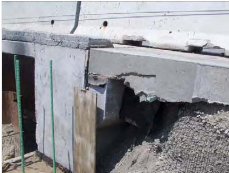
Figure 227. A closer image of the poorly-placed granular backfill (NBL)
