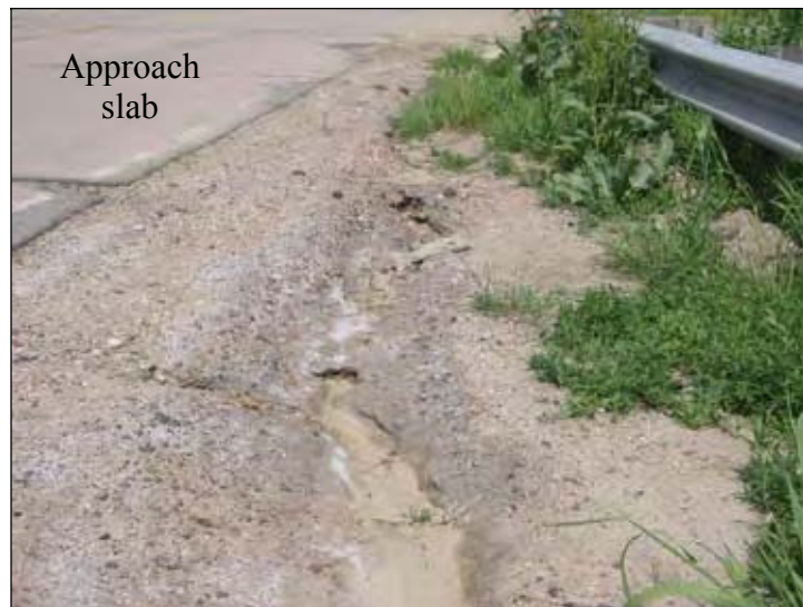
Figure 95. Erosion caused by runoff water at the approach slab shoulder
