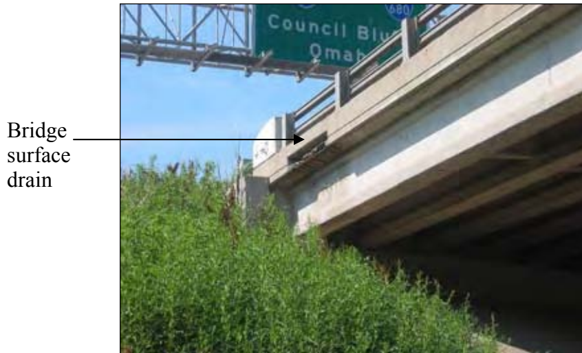
Figure 120. Surface drain of the bridge deck allowing water to fall on the embankment
