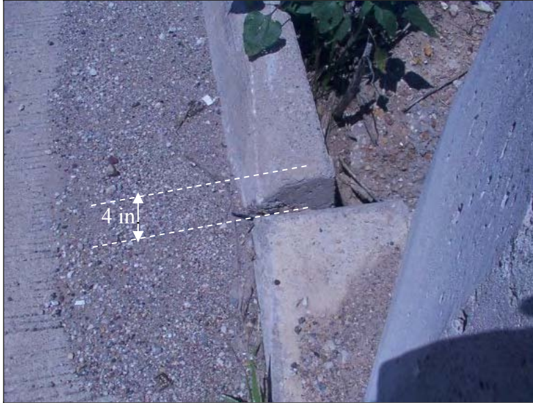
Figure 262. Differential settlement at the bridge approach (North end of NBL)
