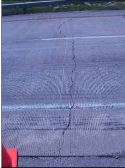
Figure 307. Transverse cracks at the bridge approach
