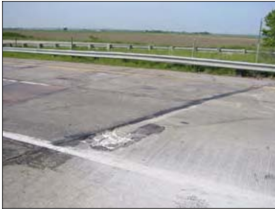
(a) Cracks on the bridge deck
