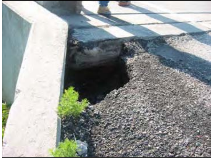
Figure 118. Failure at the shoulder of the approach slab (WBL)
