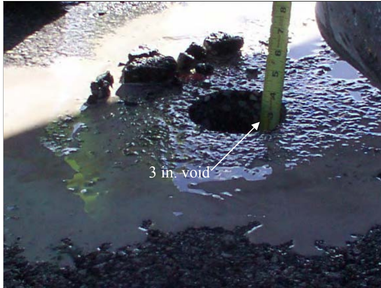
Figure 283. A 3-inch-void under the approach slab estimated by measuring the distance the core dropped (North end of SBL, edge line)
