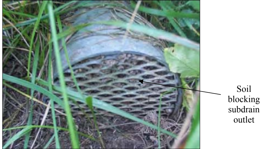
Figure 156. Subdrain outlet blocked with soil (West end of WBL)
