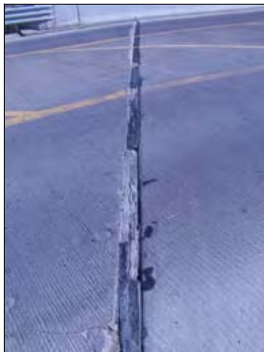
Figure 139. Deteriorated expansion joint filler
