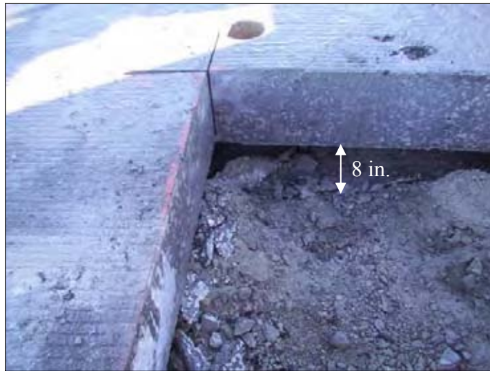
Figure 56. Eight-inch void observed under the approach slab
