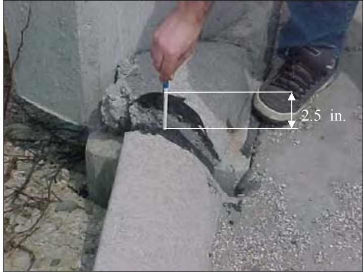
Figure 19. Differential settlement of 2.5 inches at the end of the abutment wingwall (South end SBL)
