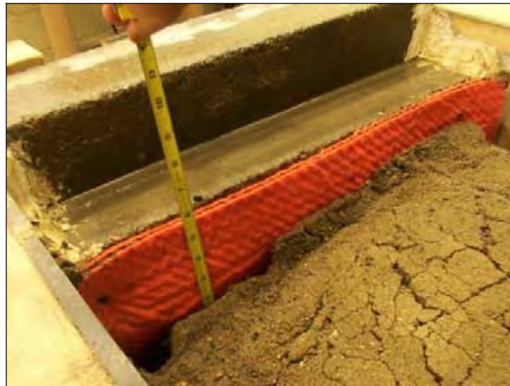
Figure 383. Void developed under the approach slab
