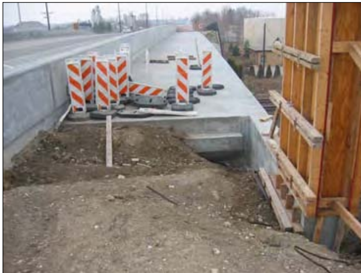
Figure 42. Non-compacted granular backfill behind the bridge abutment
