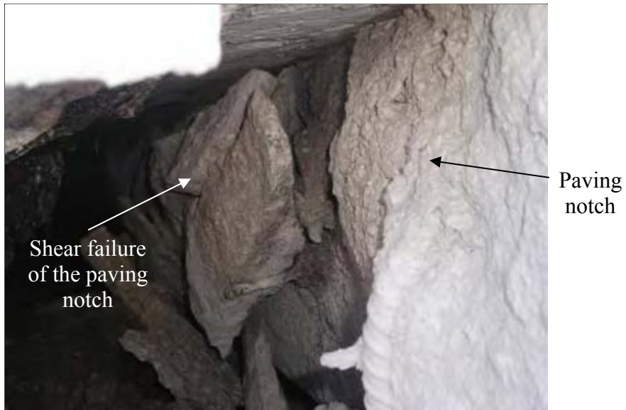
Figure 273. Shearing of paving notch (North end of SBL)
