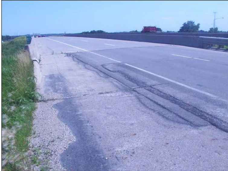
Figure 323. Asphalt overlay placed to compensate for the differential settlement (North of end NBL)
