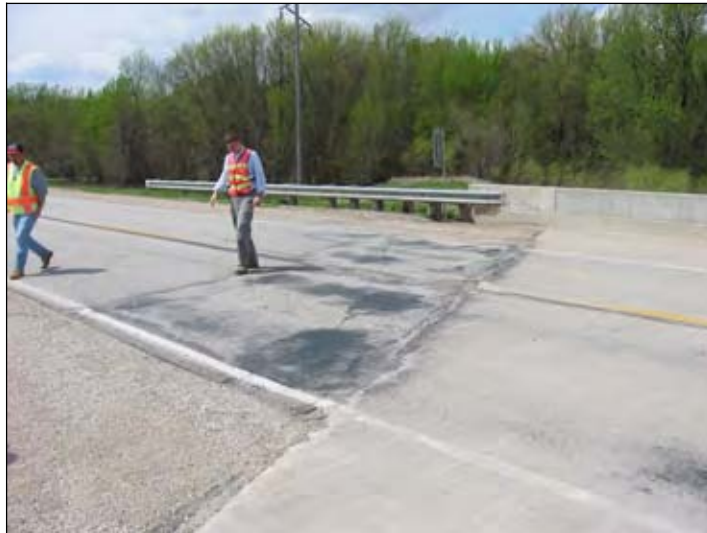
Figure 84. Cracking of asphalt overlay (East end)
