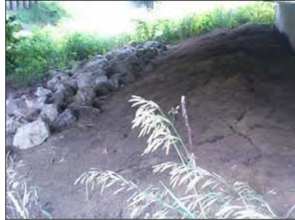
(b) Rip-rap used to control erosion
