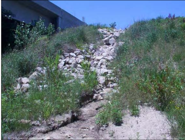
Figure 250. Rocks placed at the abutment side to prevent erosion (North end of NBL)
