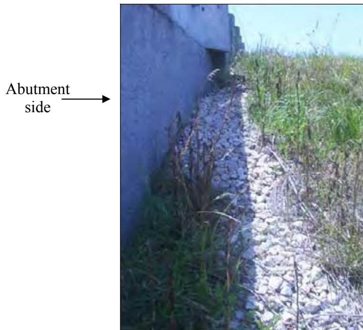
Figure 241. Aggregate placed at the sides of the abutment to control erosion (South end of SBL)
