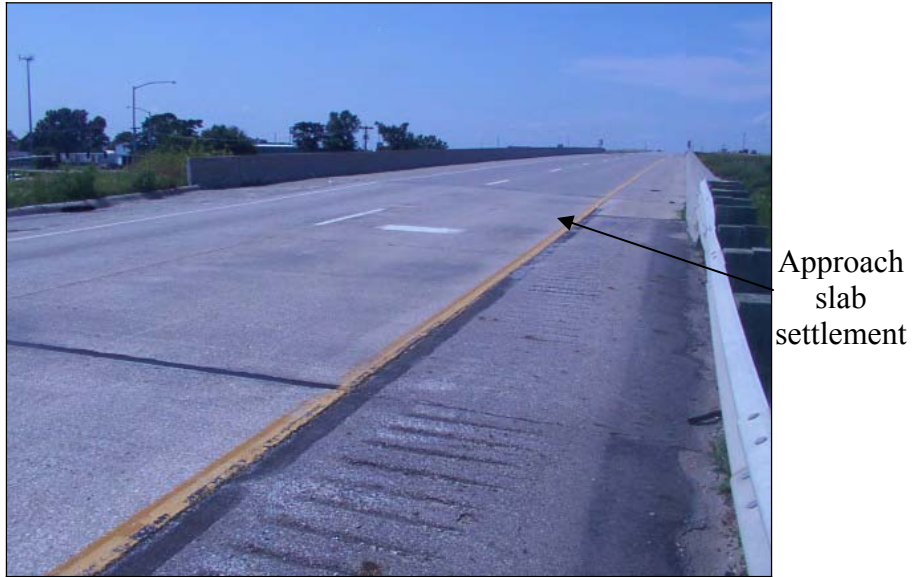
Figure 320. Bridge approach settlement (South end of SBL)
