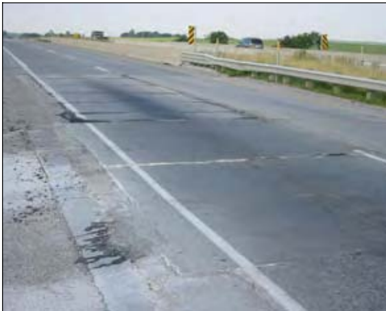
(a) Cracked approach slab panels
