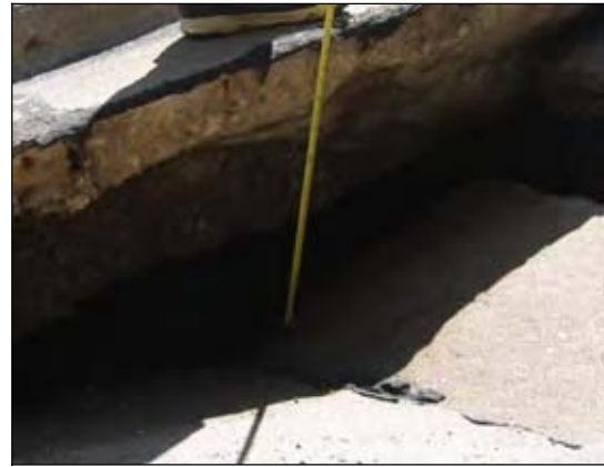
(b) Closer image of the damaged concrete
