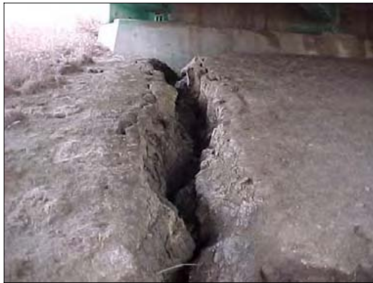
Figure 26. Erosion of the soil under the bridge (North end of SBL)
