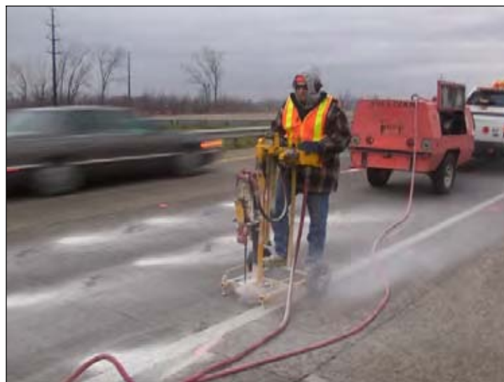
Figure 256. Holes drilled on the approach slab
