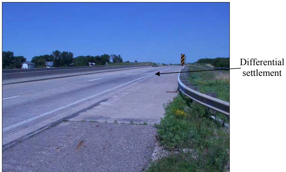
Figure 281. Differential settlement of the approach slab (North end of SBL)
