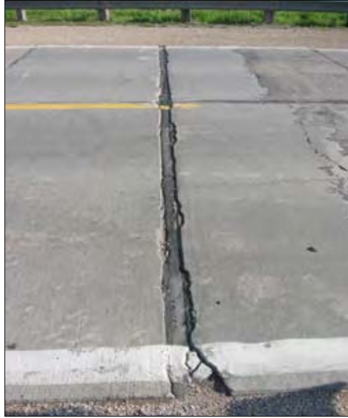
Figure 61. Concrete deterioration at the EF joint (West end)
