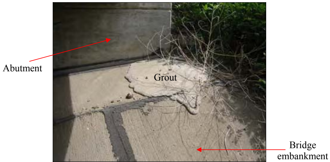
Figure 90. Grout observed on the concrete slope protection overlay indicating that void extended under the abutment
