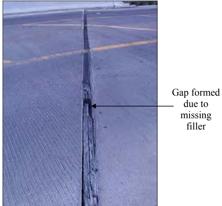
Figure 142. Missing and deteriorated filler material at the expansion joint (East end)
