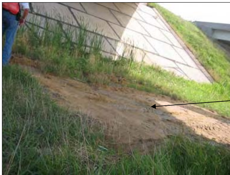
Figure 163. Grout seeping from the bottom of the embankment
