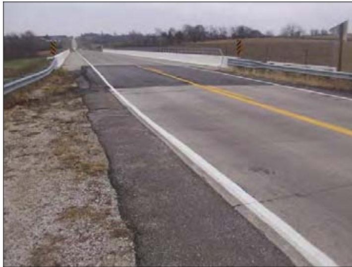
Figure 43. A view of the bridge showing recently placed asphalt overlay at the bridge approach (East end)
