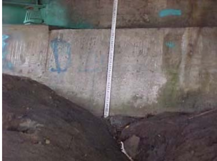
Figure 27. Erosion of the soil under the bridge (South end of SBL)
