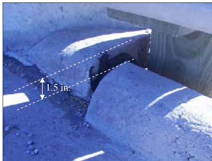
Figure 330. Differential settlement between the bridge approach and the approach slab (West end of EBL)
