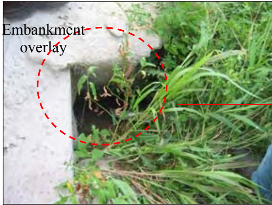
(a) Void under slope protection
