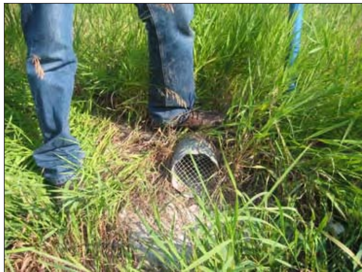
Figure 113. Dry end drain with no indication of water flowing out
