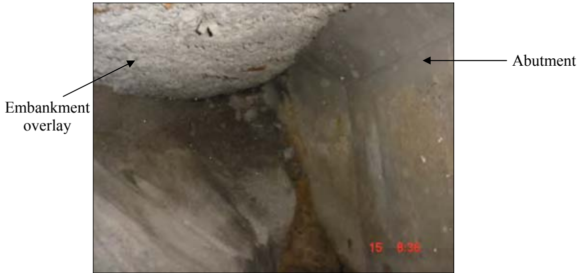
Figure 180. Erosion under the concrete slope protection (Side view)
