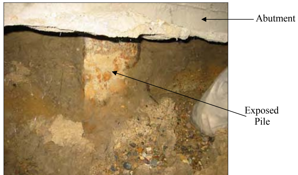
Figure 105. Exposed H-pile caused by soil erosion under the abutment
