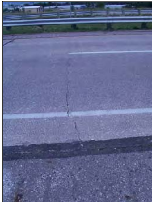
Figure 319. Transverse cracking at the bridge approach (North end of SBL)
