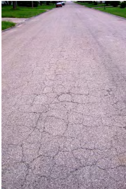
Figure 25. Reflected alligator cracking (no chipmat)
