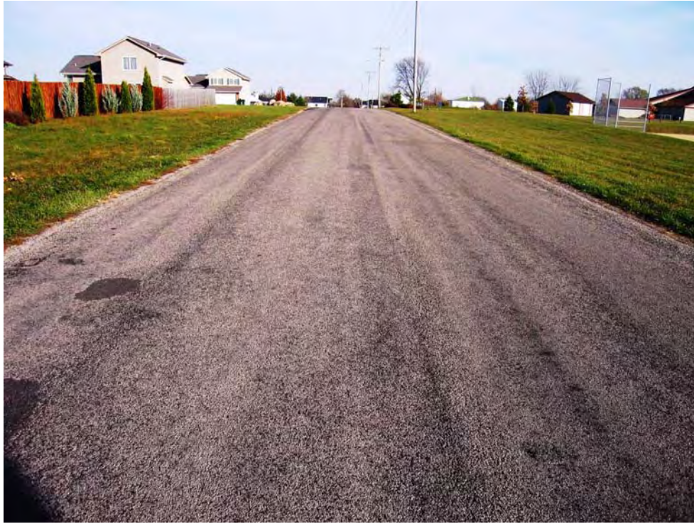
Figure F.7. Typical view of double seal coat on 74th Street (digitally enhanced photo)
