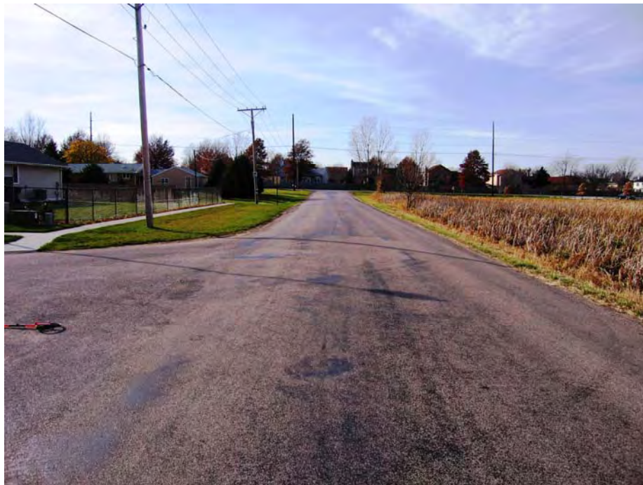
Figure F.4. Typical view of pre-coated limestone on 74th Street (digitally enhanced photo)
