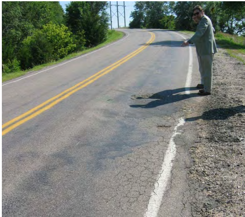
Figure 13. College Road alligator cracking, potholes, and bleeding
