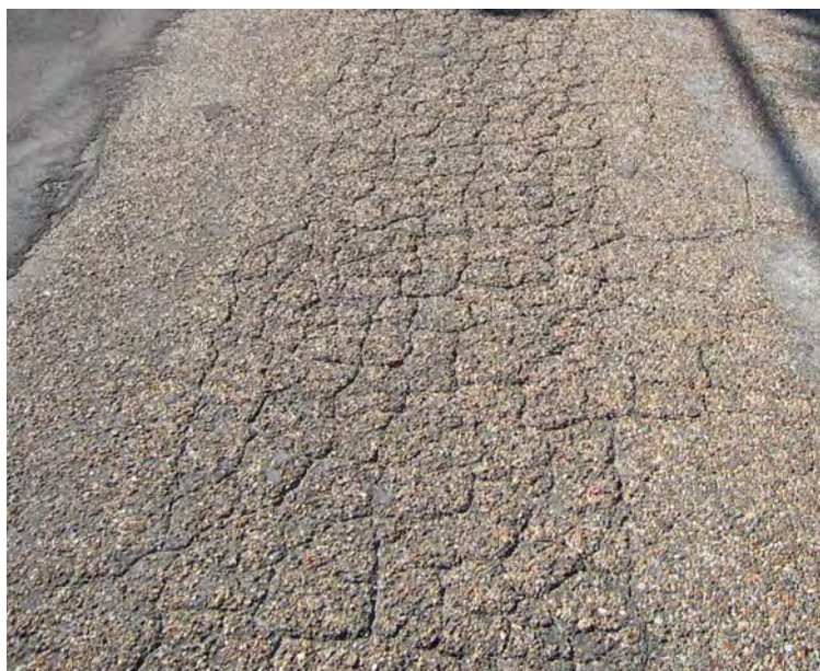
Figure 4. Alligator cracking on Vermont Avenue
