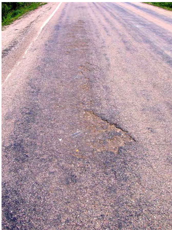
Figure 34. College Road alligator cracking
