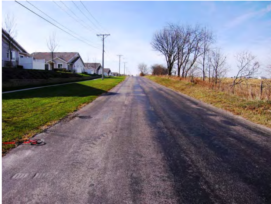
Figure F.5. Typical view of washed limestone on 74th Street (digitally enhanced photo)
