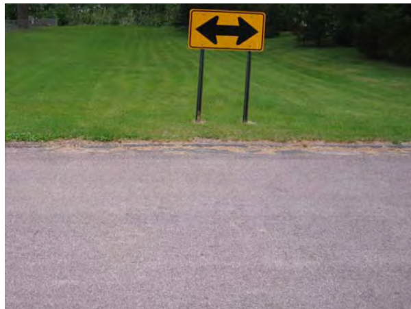
Figure 24. No reflected alligator cracking (chipmat)
