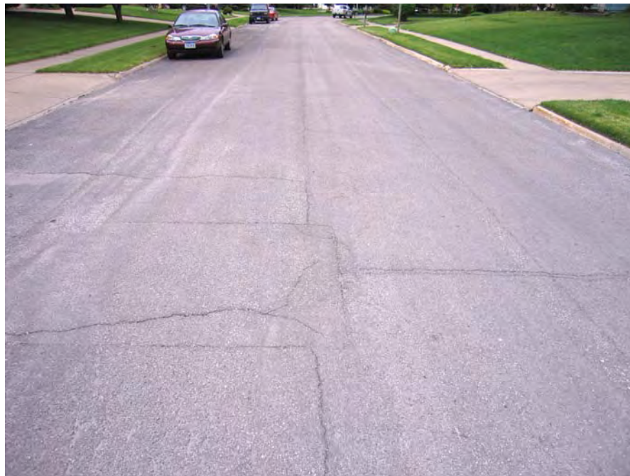
Figure 38. Reflective cracking on Aspen Drive
