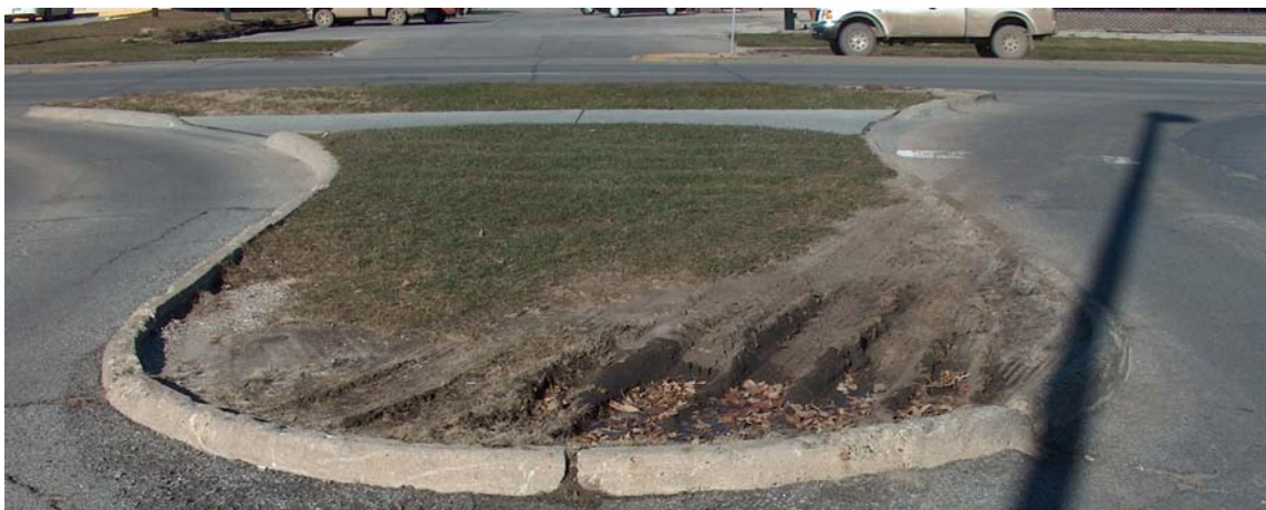
Figure 2-1. Wheel ruts in a median with an inadequate turning radius for trucks
