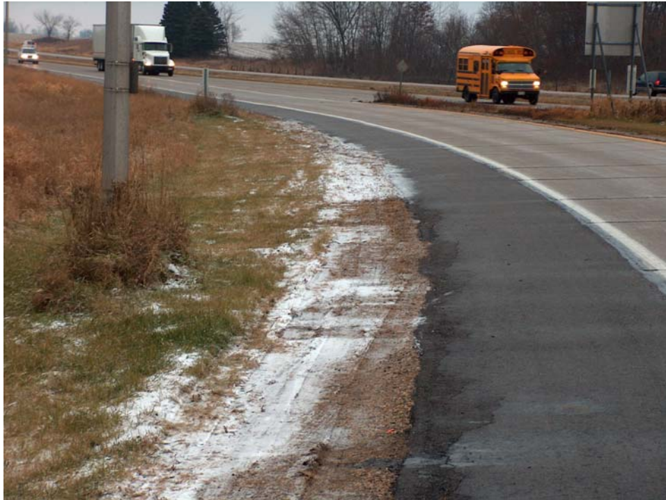
Figure 4-4. Truck tire tracks on ramp shoulder
