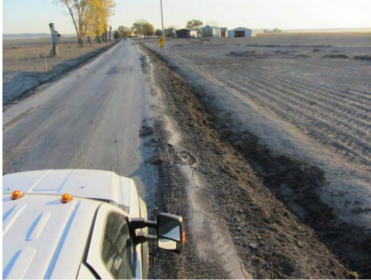
Figure 48. Rutting along right wheel path on chipseal surfaced gravel road and erosion of granular shoulder during flooding – 220th Street, Fremont County (Photo taken 10/26/11)
