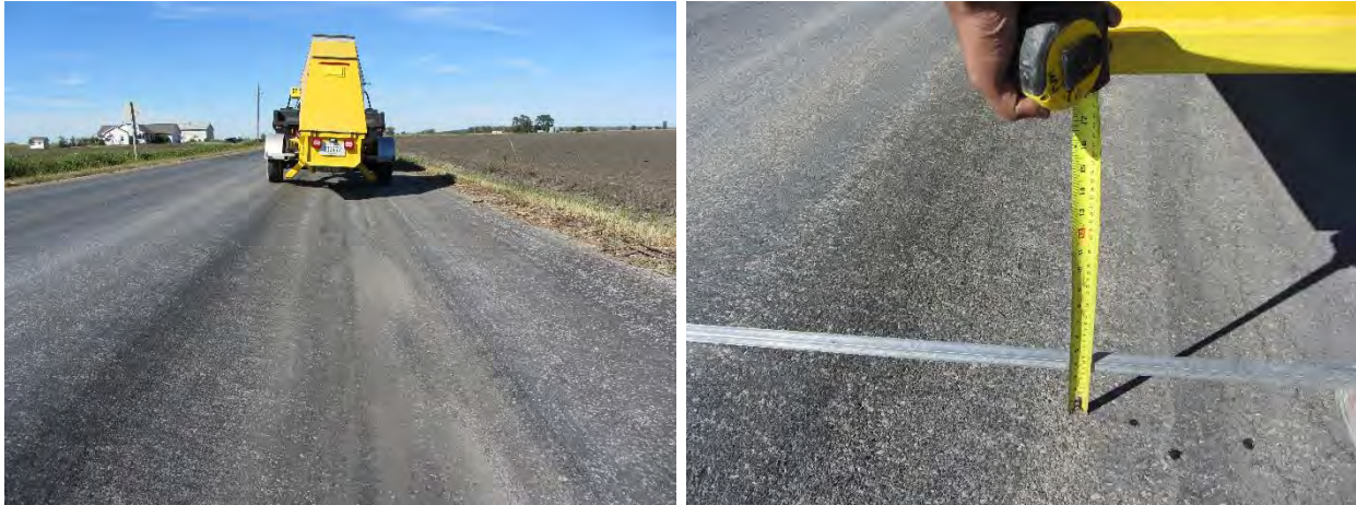
Figure 82. Rutting observed near the east end of the test segment (near test location D-38) (photo taken on 9/23/11) on TS4 – Pottawattamie County
