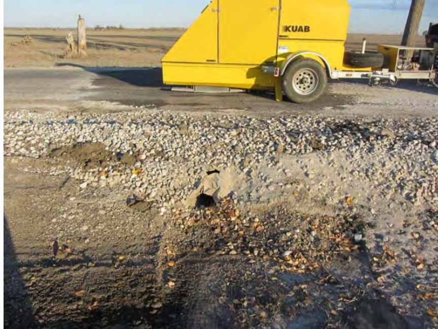
Figure 163. Surface patch repair over a culvert on TS4 – Fremont County (Picture taken 10/28/11)
