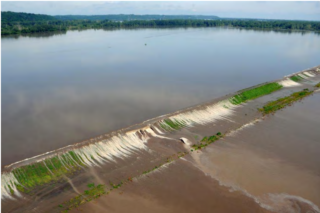
Figure 13. Aerial photo of the overtopping of Federal levee 550 near Highway 136 in Atchison County, Missouri, on June 19, 2011 (Image Courtesy of USACE http://www.flickr.com/photos/usacehq/5849817627/in/photostream/ )
