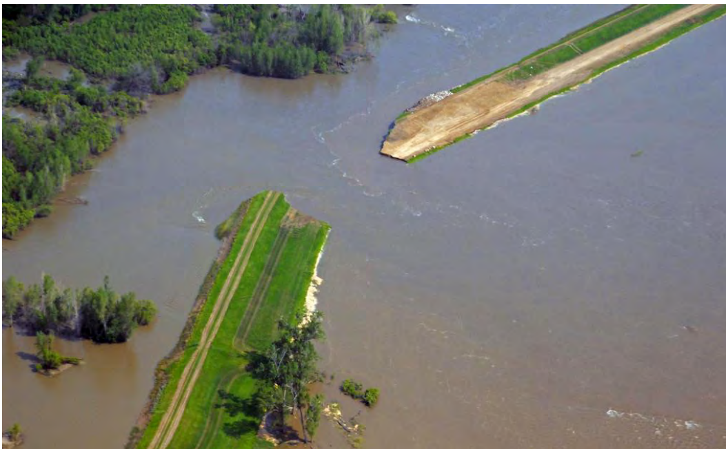
Figure 11. Aerial photo of the full breach at Federal levee 575 near Hamburg, Iowa, on June 14, 2011 (Image Courtesy of USACE http://www.flickr.com/photos/usacehq/5837117182/in/photostream/ )
