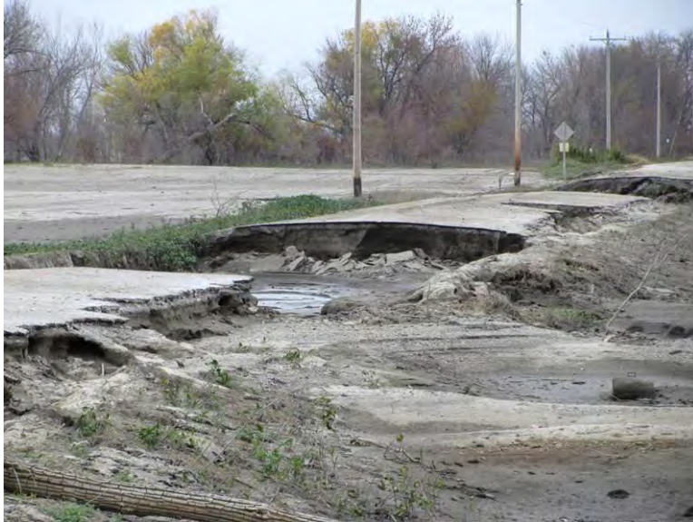
Figure 52. Gravel road segments washed away during floods – Fremont County (Photo taken on 10/26/11)
