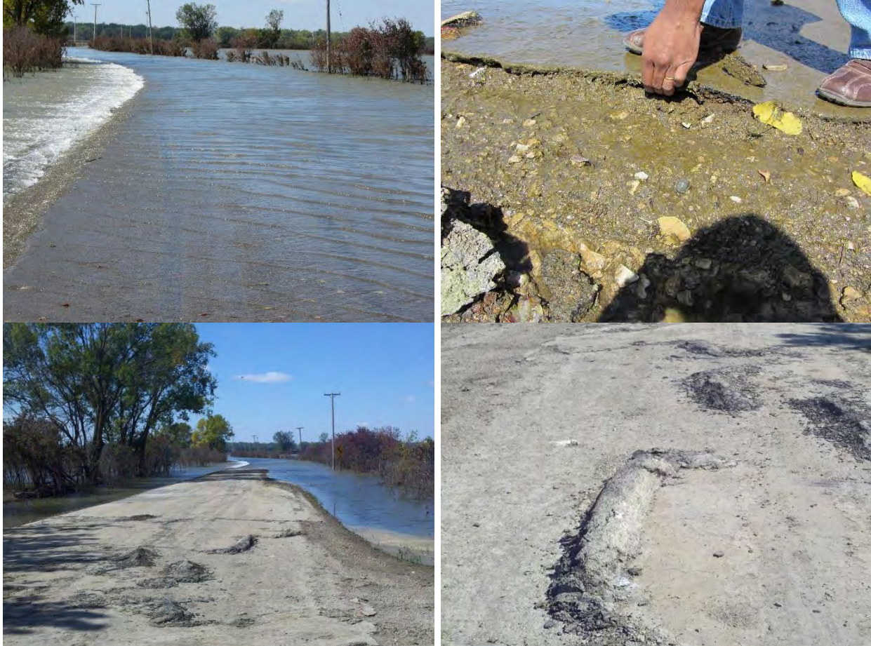
Figure 42. Water overtopping a thin chipseal coat surfaced road underlain by oil stabilized granular base on 9/21/11 showing delamination of chipseal and rolled asphalt at the surface – Desoto Avenue, Pottawattamie County (Photos taken on 9/21/11)
