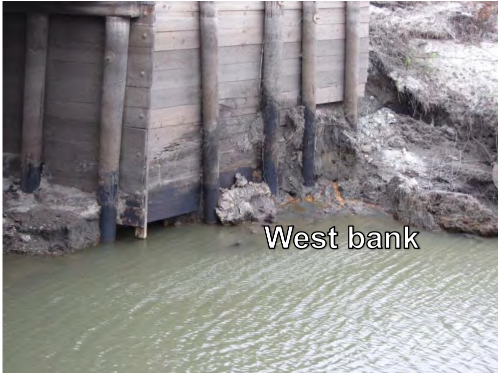
Figure 132. Erosion of embankment material along the west bank near abutment wing walls on TS1 (Picture taken on 10/26/11) – Fremont County
