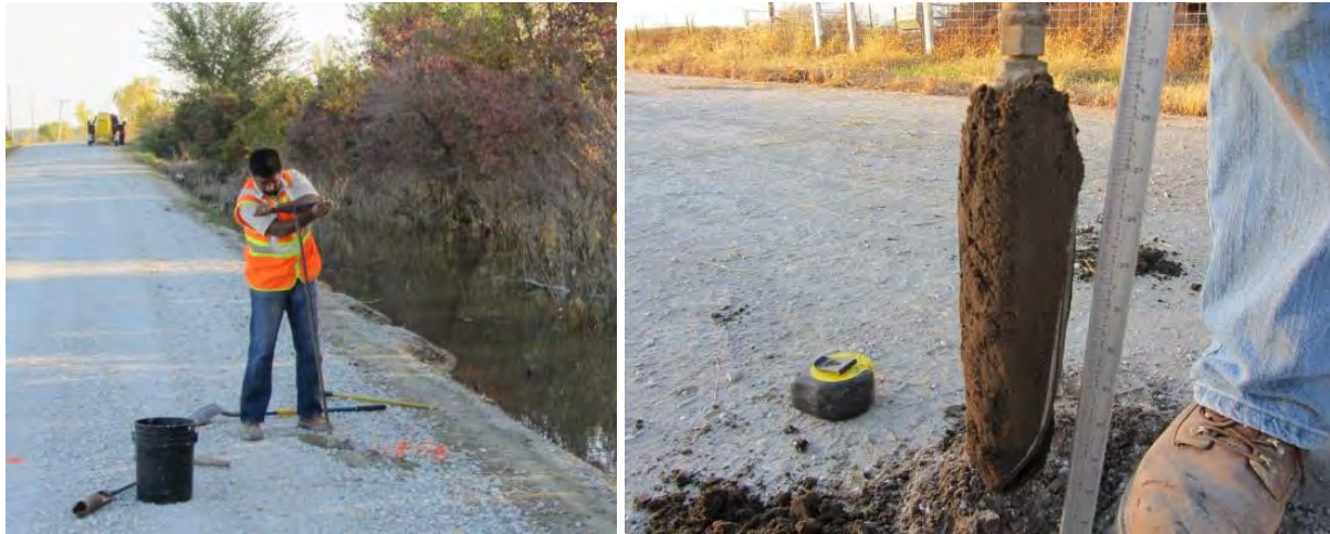
Figure 24. Extracting soil samples using a hand auger equipped with a Dutch auger head
