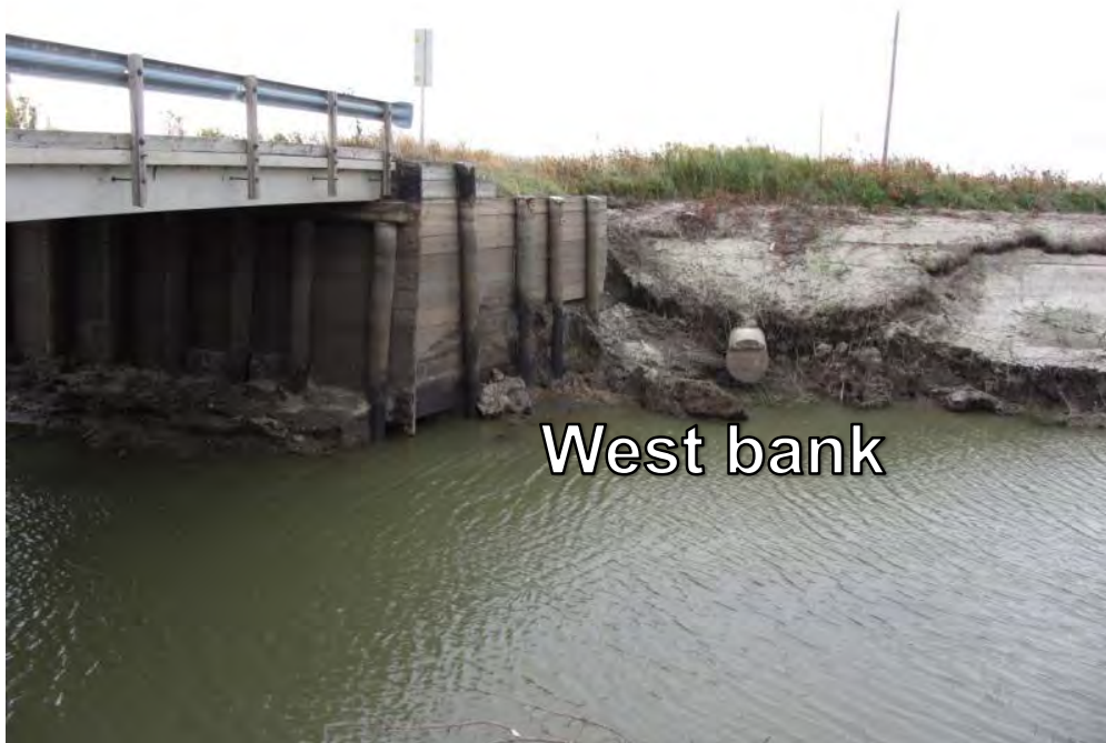
Figure 131. Erosion of embankment material along the west bank on TS1 (Picture taken on 10/26/11) – Fremont County
