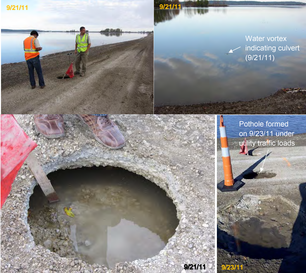
Figure 46. Potholes (with about 0.5 m (1.5 ft) diameter) under gravel road due to erosion of backfill material around a culvert located beneath the road – Pottawatamie County (Photos taken on 9/21/11 and 9/23/11)
