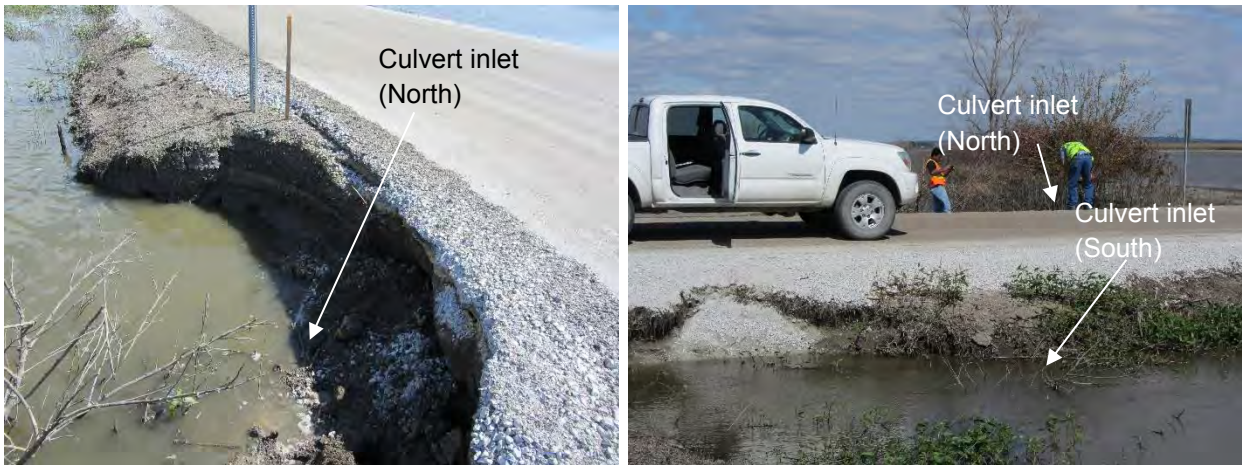
Figure 43. Clogged culvert inlets due to scouring and erosion of embankment material beneath chipseal coat surfaced road on 9/21/11 – Desoto Avenue, Pottawatamie County (Photos taken on 9/21/11)
