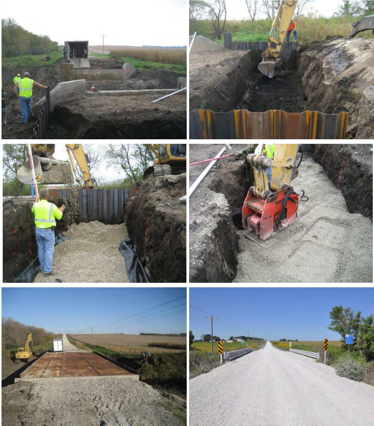
Figure D40. Pictures of a bridge site in Buchanan County (250 th Street) during construction of GRS fill in bridge abutments, placement of rail road flat cars for superstructure, and after final placing the final gravel surface in 2011 (Vennapusa et al. 2012)
