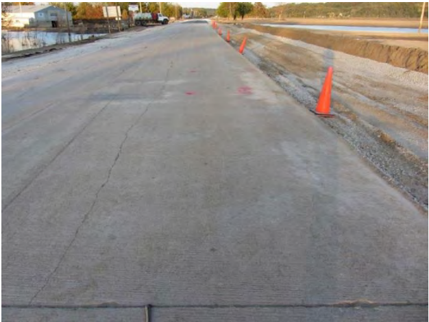
Figure 64. Longitudinal cracks on PCC pavement with undermined base material on TS2 (Photo taken on 9/21/11) – Pottawattamie County
