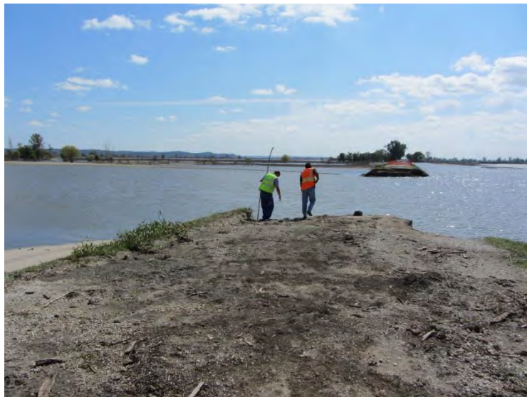
Figure 45. Full breach of about 150 m (500 ft) long unsurfaced access road – Pottawatamie County (Photo taken on 9/21/11)
