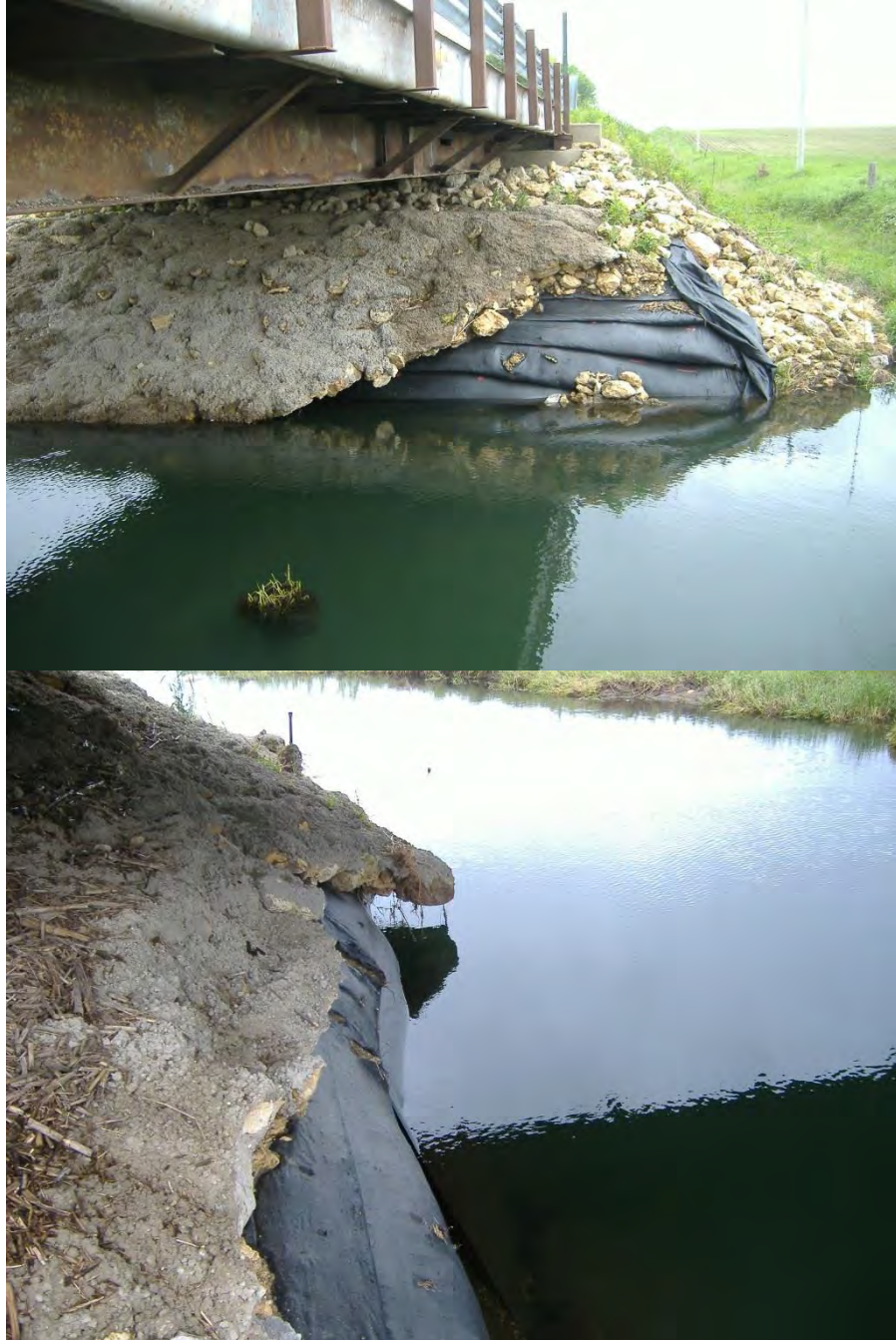
Figure D41. Pictures of a bridge site in Buchanan County (Olympic Ave.) after flash flooding occurred in May 2013
