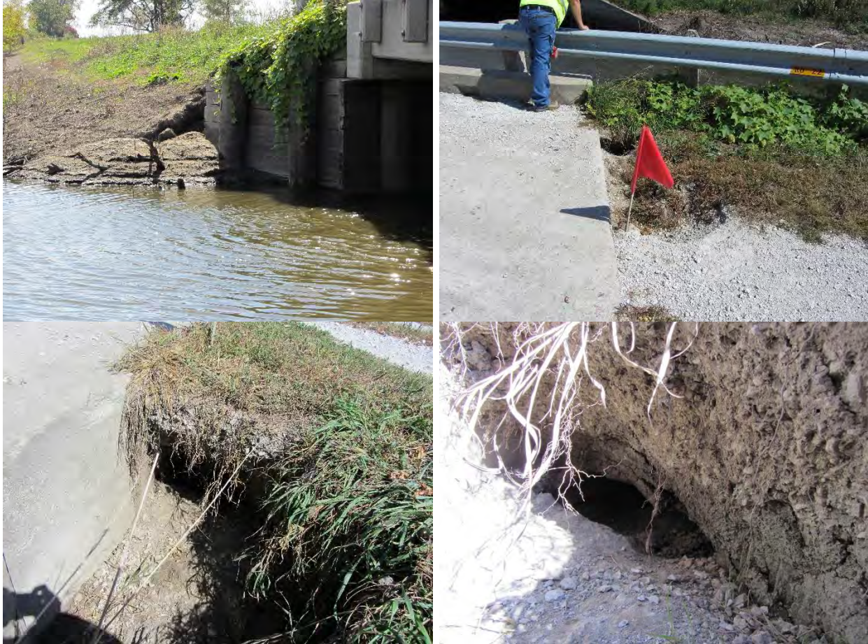
Figure 44. Scouring and erosion of bridge backfill material around a timber abutment supporting a concrete bridge deck – Pottawatamie County (Photos taken on 9/21/11)
