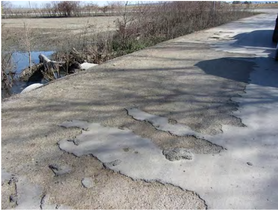
Figure 121. Delaminated surface chipseal on Desoto Avenue due to flood waters overtopping the roadway (Pictures taken on 10/25/11) – Pottawattamie County
