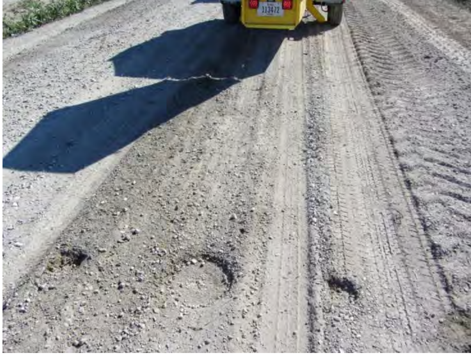
Figure 110. FWD plate depression and rutting under truck wheels near culvert (Picture taken on 9/23/2011) – Pottawattamie County
