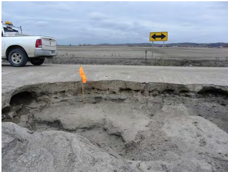
Figure 49. Erosion of shoulder and roadbed on a chip seal surfaced gravel road – Fremont County (Photo taken on 10/26/11)
