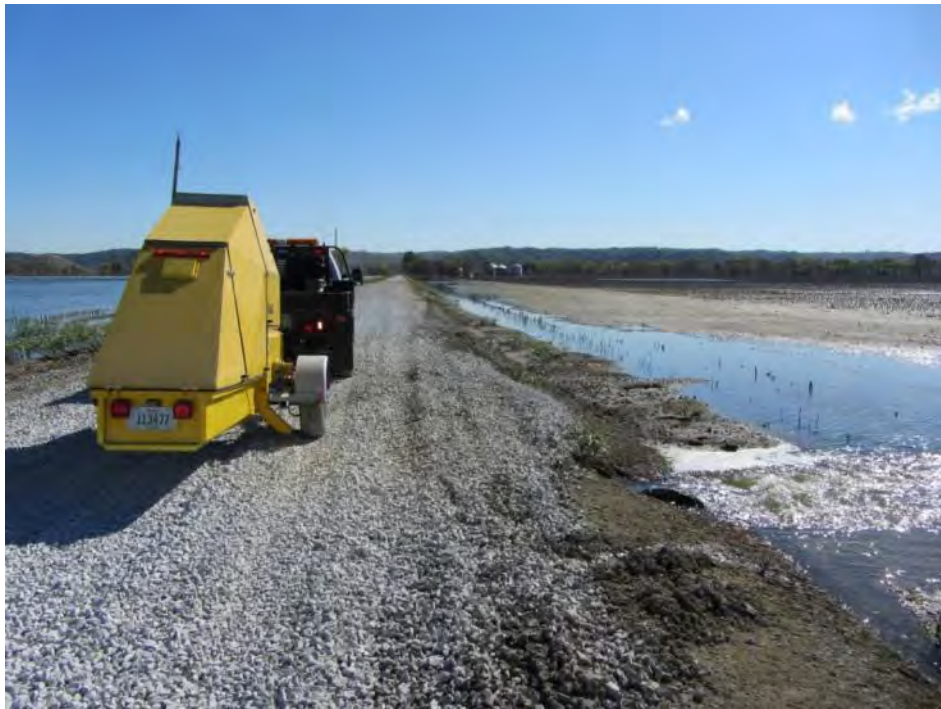
Figure 111. Newly placed gravel showing rutting near culvert (Picture taken on 9/23/2011) – Pottawattamie County
