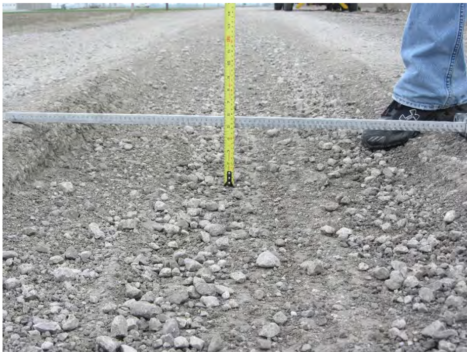
Figure 156. Rutting observed near 3000 m station on TS2 (Picture taken 4/4/12)
