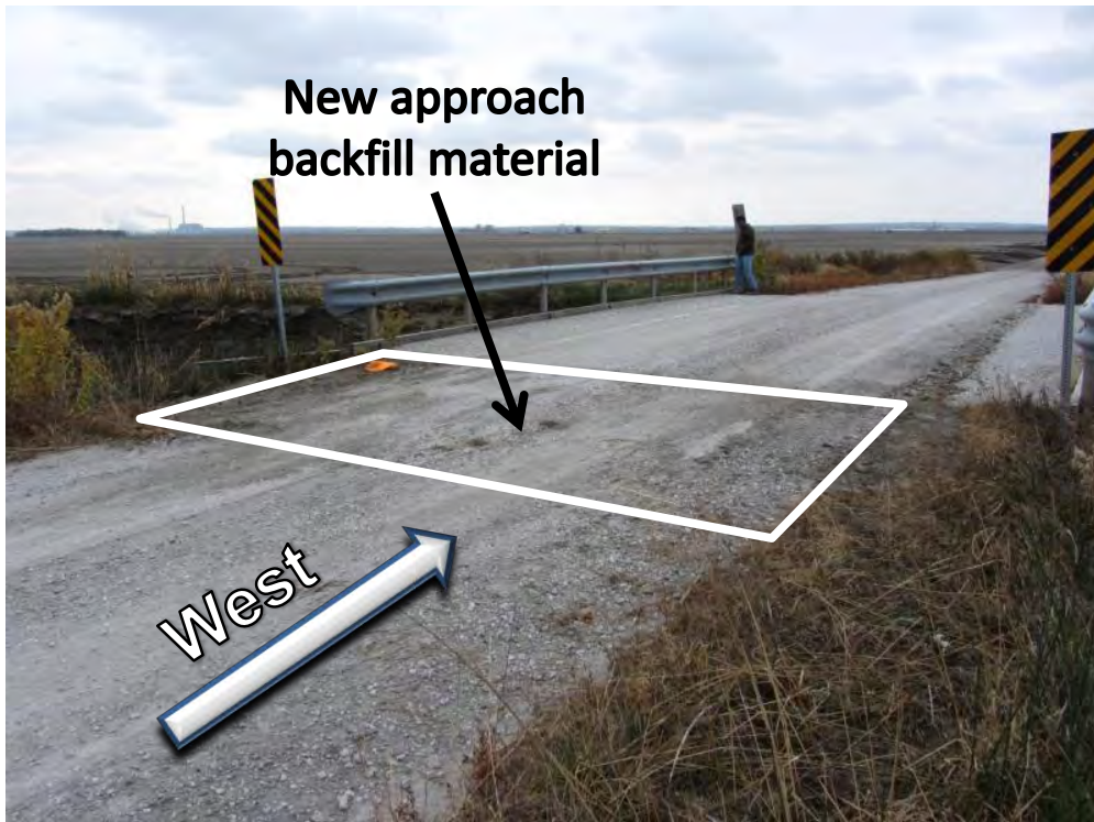
Figure 130. New bridge approach backfill material placed along the east approach on TS1 (Picture taken on 10/26/11) – Fremont County
