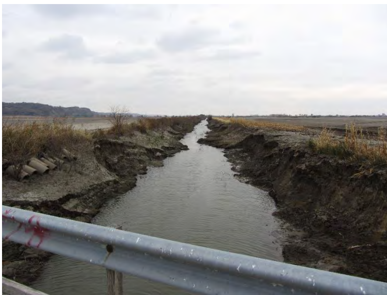
Figure 54. Erosion of backfill material around timber back wall supporting a timber bridge crossing a creek – Fremont County (Photos taken on 10/26/11)
