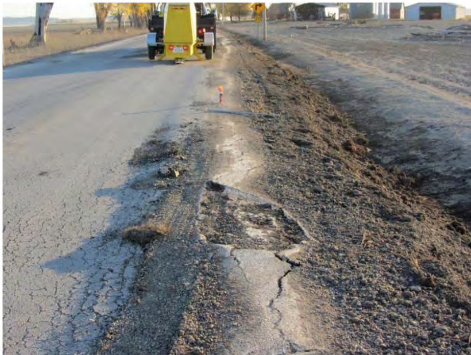
Figure 162. Rutting observed on the surface and washed out shoulders during flooding on TS4 – Fremont County (Picture taken 10/28/11)
