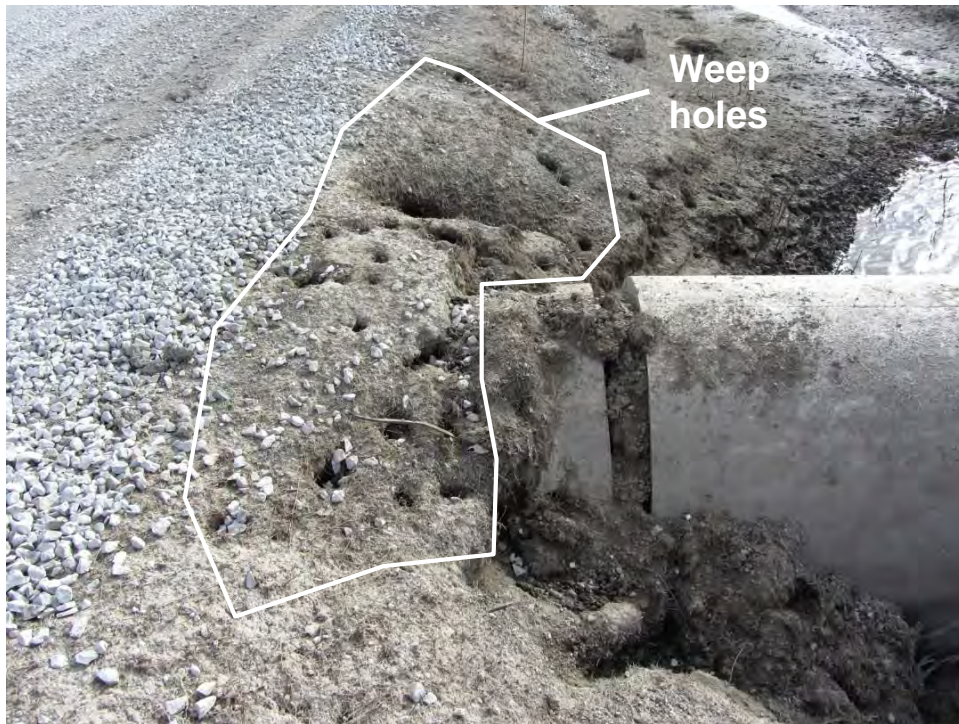
Figure 91. Weep holes (20+) around the culvert observed after flood waters receded on TS5 (Photo taken on 10/25/11) – Pottawattamie County
