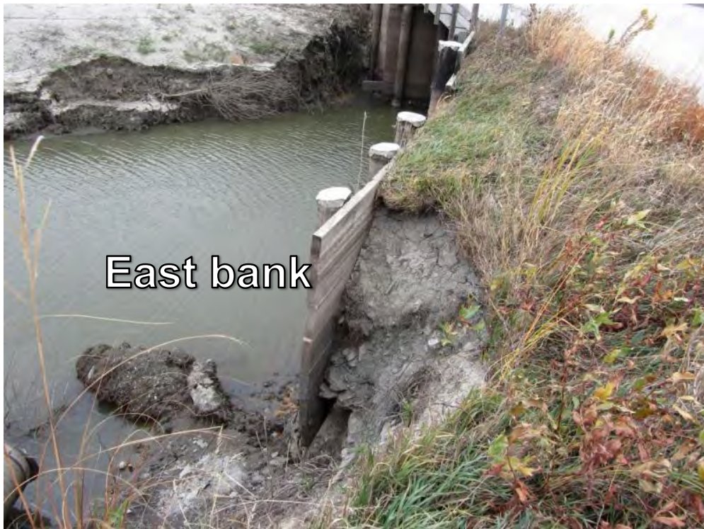
Figure 133. Erosion of backfill material behind the wing wall on TS1 (Picture taken on 10/26/11) – Fremont County
