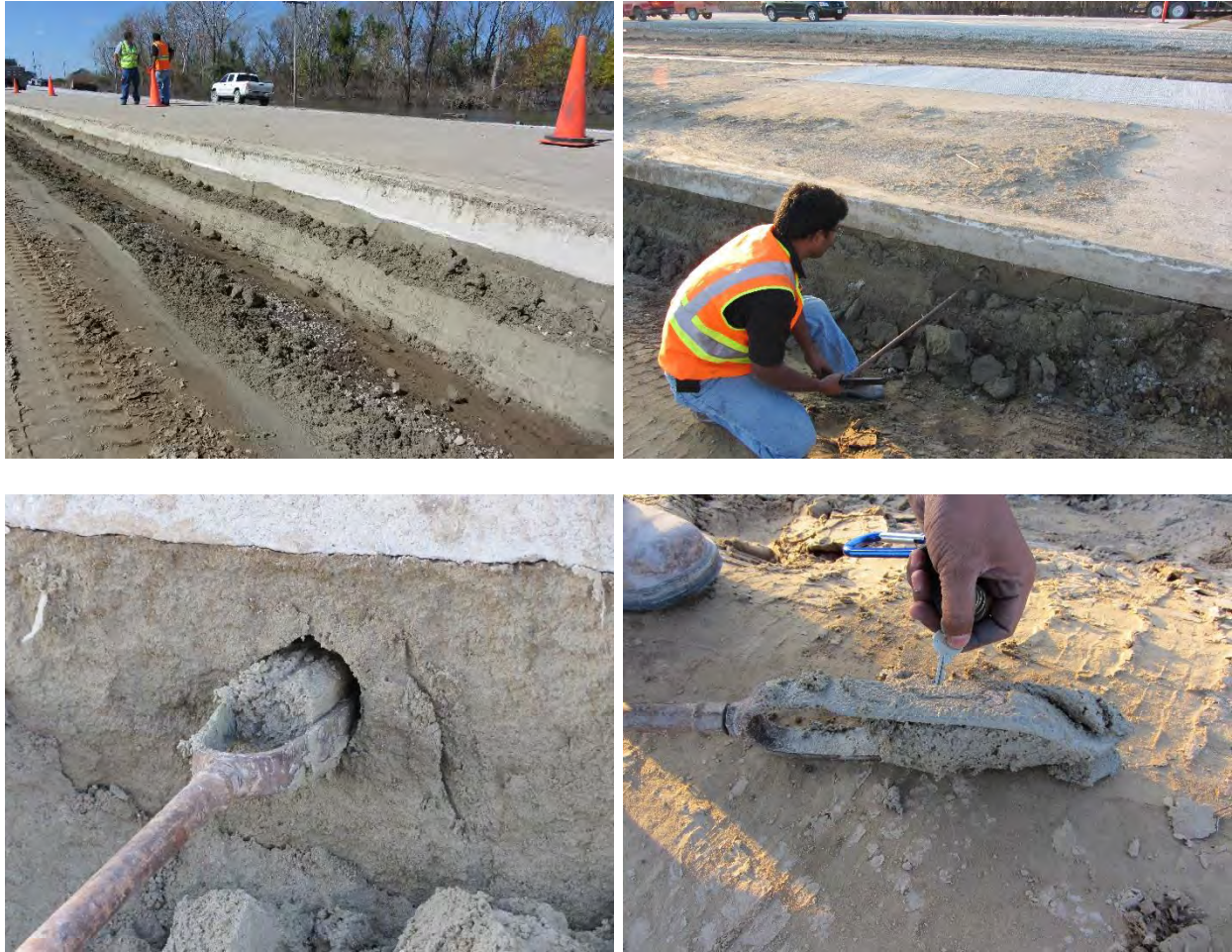
Figure 63. Eroded base material and voids under PCC pavement filled with cement grout – TS2 [Note: Cement grout was placed two days prior to taking these photos] (Photos taken on 9/21/11) – Pottawattamie County
