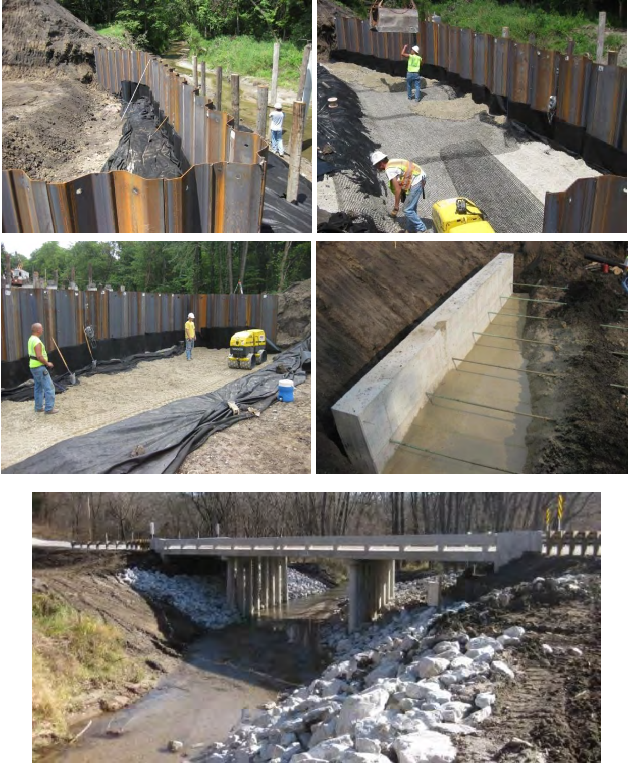
Figure D37. Pictures of a bridge site in Boone constructed with sheet pile abutments with geogrid-reinforced backfill material (Evans et al. 2012)
