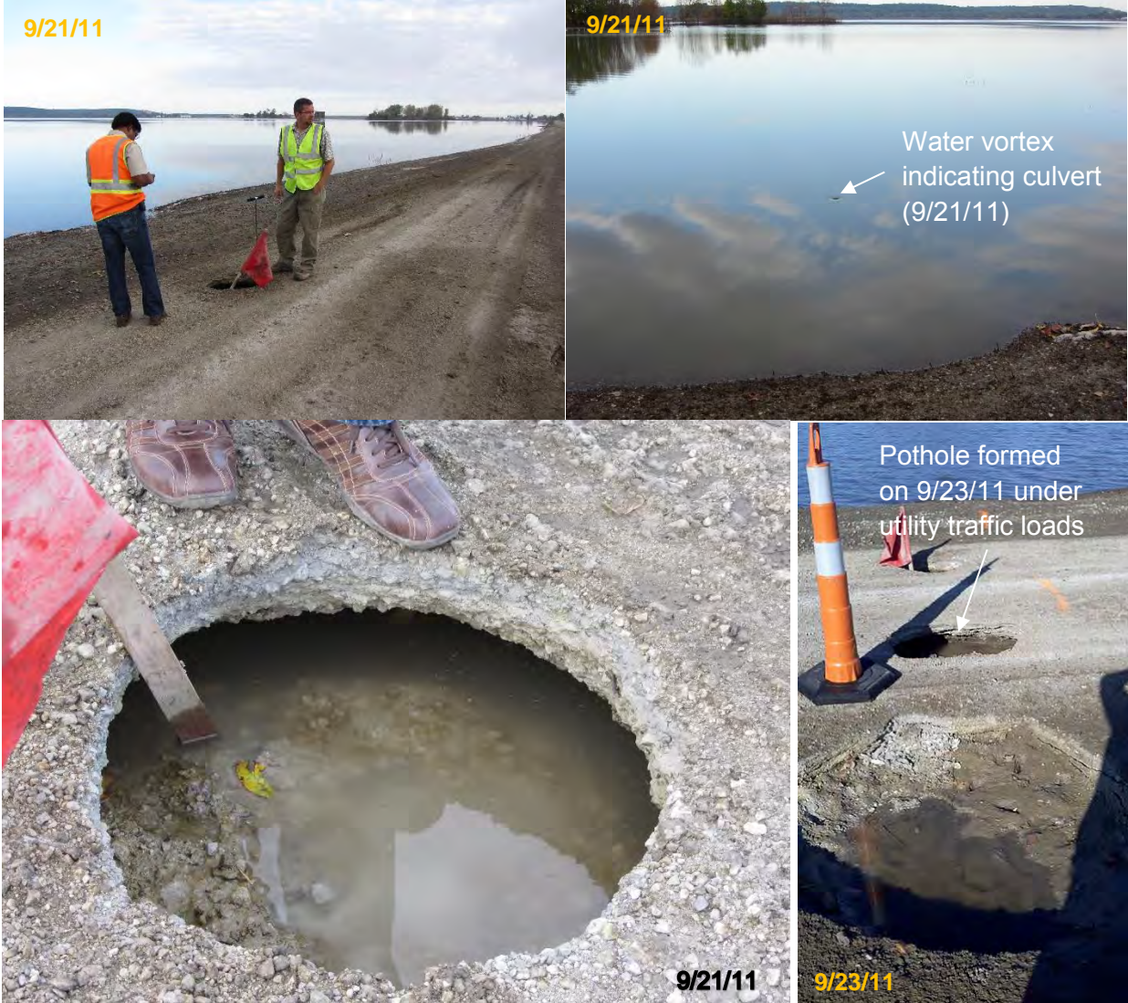
Figure 89. Potholes (with about 0.5 m (1.5 ft) diameter) under gravel road due to erosion of backfill material around a culvert located beneath the road TS 5 (Photos taken on 9/21/11 and 9/23/11) – Pottawatamie County
