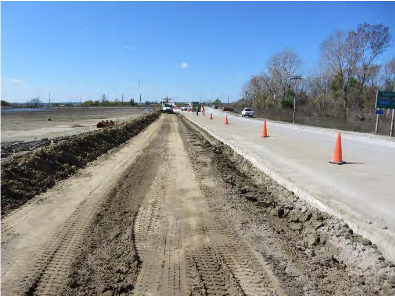
Figure 41. Eroded shoulder next to PCC pavement being reconstructed on 9/21/11 – Old Mormon Road (looking west towards I-680 and I-29 intersection), Pottawatamie County (Photos taken on 9/21/11)
