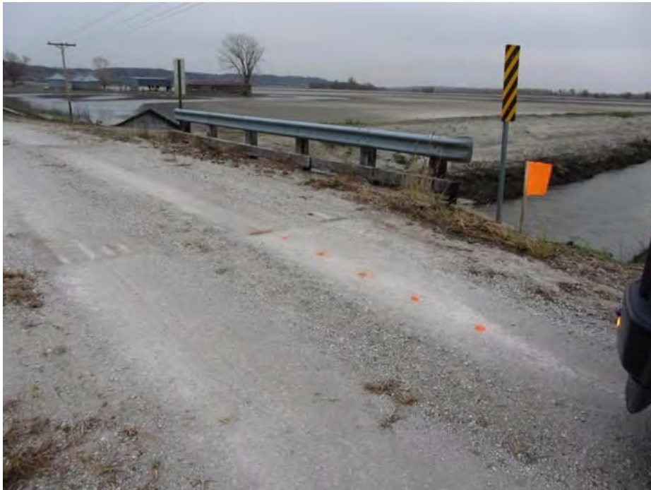
Figure 145. Bridge approach on TS2 (Picture taken 10/26/11)
