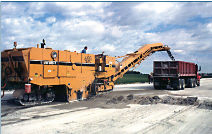
Figure 54. Typical concrete pavement milling operation (Photo courtesy of Randell Riley, P.E., Illinois Chapter ACPA)
