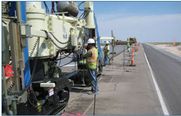
Figure 37. Typical clearance on a concrete overlay project (Photo courtesy of Matt Ross, P.E., Missouri/Kansas Chapter ACPA)
