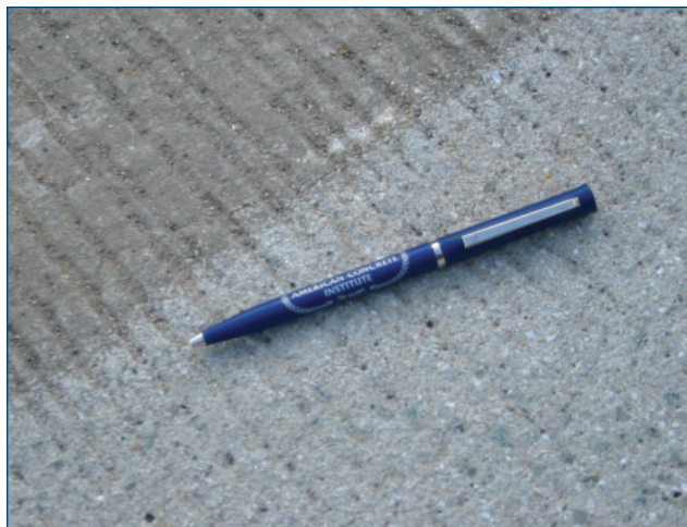
Figure 49. Compare the surface texture of the non-shotblasted area (upper left half of image) to the roughened surface texture on the shotblasted section of pavement (under the pen) (Photo courtesy of Leif Wathne, P.E., American Concrete Pavement Association)
