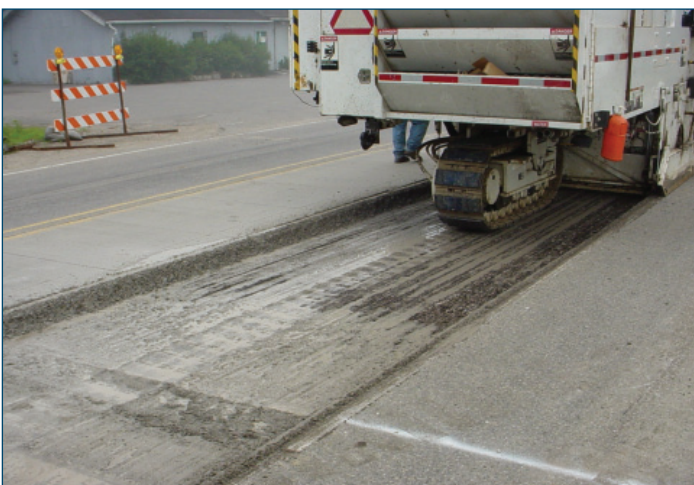
Figure 55. Typical concrete pavement milling operation (Photo courtesy of Dan DeGraaf, P.E., Michigan Concrete Paving Association)
