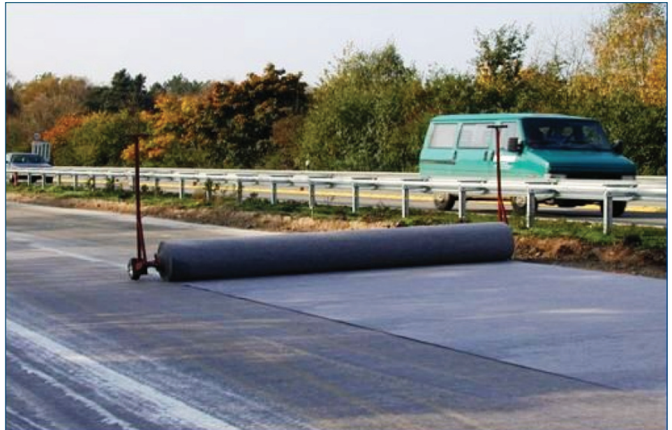
Figure 35. Roll of geotextile fabric being placed prior to overlay (Photo courtesy of Prof. Gunther Leykauf, Technische Universität München)
