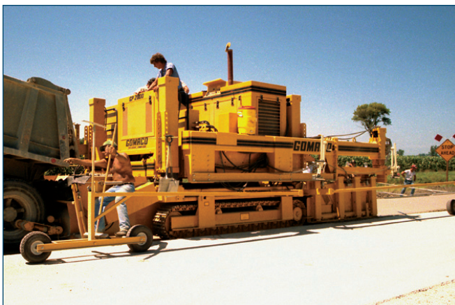
Figure 40. Controlling paving profile using a moveable stringline on the adjacent lane (Photo courtesy of Kevin Klein, Gomaco)
