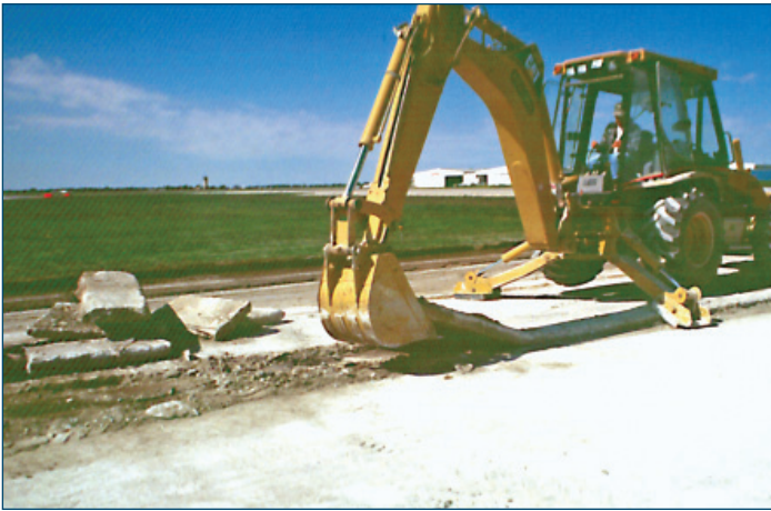
Figure 52. Removing overlay panels (Photo courtesy of Randell Riley, P.E., Illinois Chapter ACPA)
