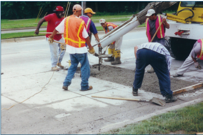
Figure 53. Finish and cure of concrete overlay repair (Photo courtesy of Dan DeGraaf, P.E., Michigan Concrete Paving Association)
