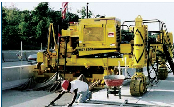
Figure 38. A three-track, zero-clearance paver placing concrete along a median barrier (Photo courtesy of Kevin Klein, Gomaco)
