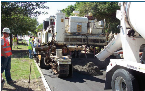
Figure 39. A typical, four-track paver modified to three tracks, providing zero clearance in a curb-and-gutter situation in Oklahoma (Photo courtesy of Jim Duit, Duit Construction Co., Inc.)
