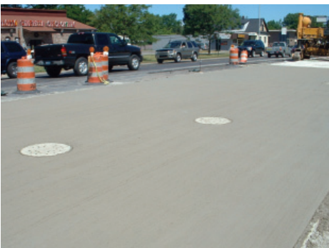
Urban concrete overlay construction (Photo courtesy of Kerry Sutton, P.E., Michigan Concrete Paving Association)
