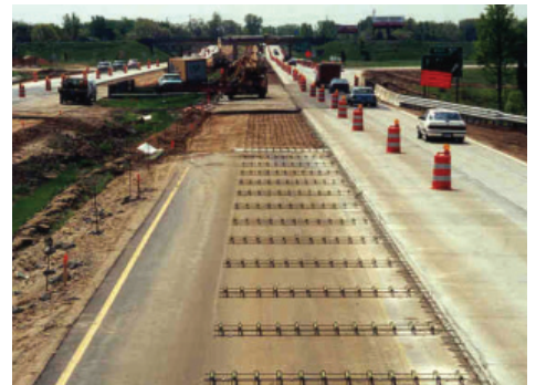
Interstate highway concrete overlay construction (Photo courtesy of Dan DeGraaf, P.E., Michigan Concrete Paving Association)
