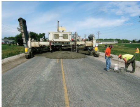
Rural concrete overlay construction with widening (Photo courtesy of Gordon Smith, P.E., Iowa Concrete Paving Association)
