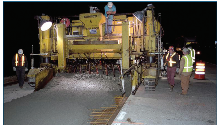
Figure 41. Controlling paving profile using a paver ski on the adjacent lane (Photo courtesy of Wouter Gulden, P.E., Southeast Chapter ACPA)
