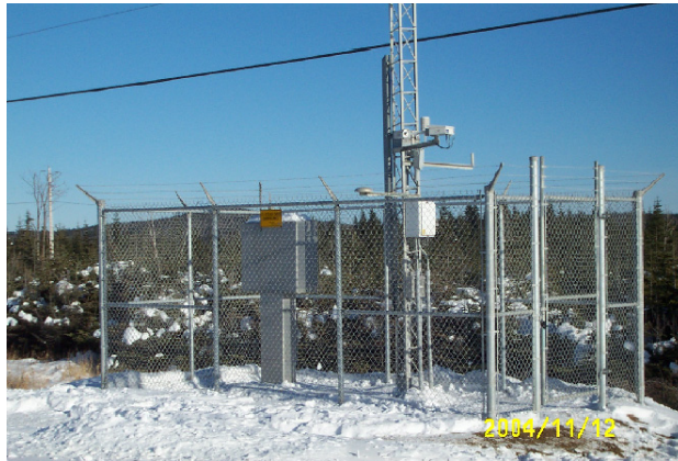
Figure 32. The road weather station
