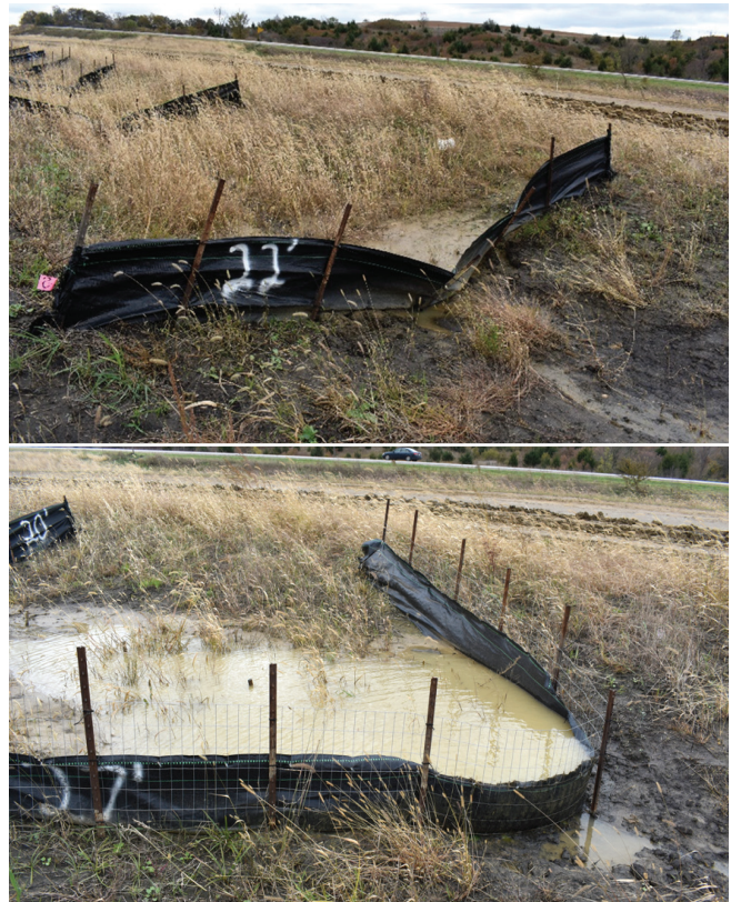
Observed T-post deflection and undercutting on standard silt fence ditch check installation, top, and impoundment on modified silt fence installation, bottom
