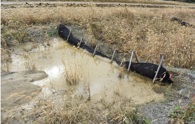
Observed undercutting on standard wattle ditch protection, top, and sedimentation upstream of a modified wood chip wattle installation, bottom
