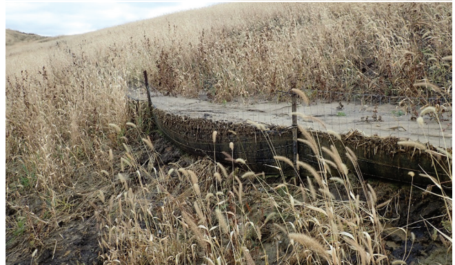
Observed T-post deflection and overtopping on standard silt fence perimeter control practice, top, and sediment retention on modified silt fence perimeter control with 5 ft T-post spacing, middle, and 8 ft T-post spacing, bottom
