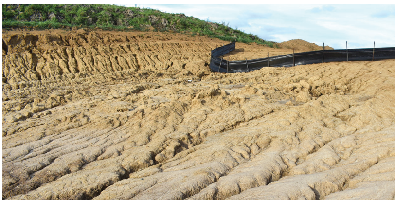
Observed site erosion on Iowa US 30 highway expansion project
