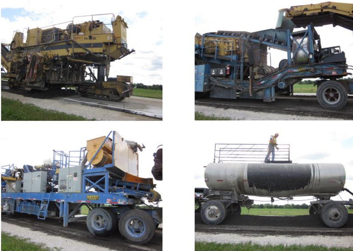
Figure 9. Cold in-place recycling train with milling machine (top left), crushing and screening unit (top right), pug mill (bottom left), and oil tank trailer (bottom right)
