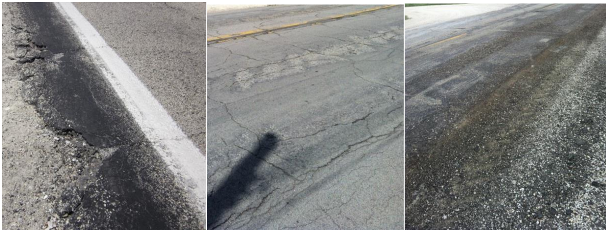
Figure 19. Existing pavement surface condition
