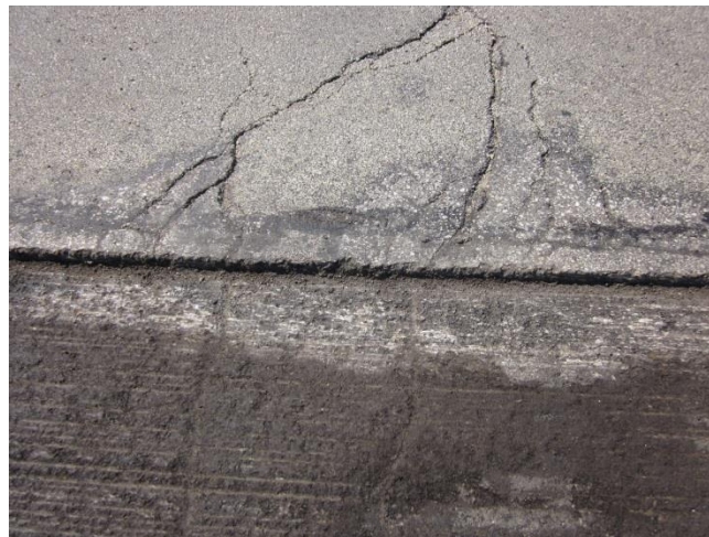
Figure 8. Cracks that had propagated deeper than milling depth
