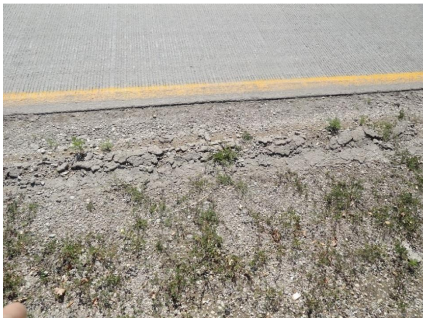
Figure 27. Northbound inside shoulder of US 63 near Denver, Iowa
