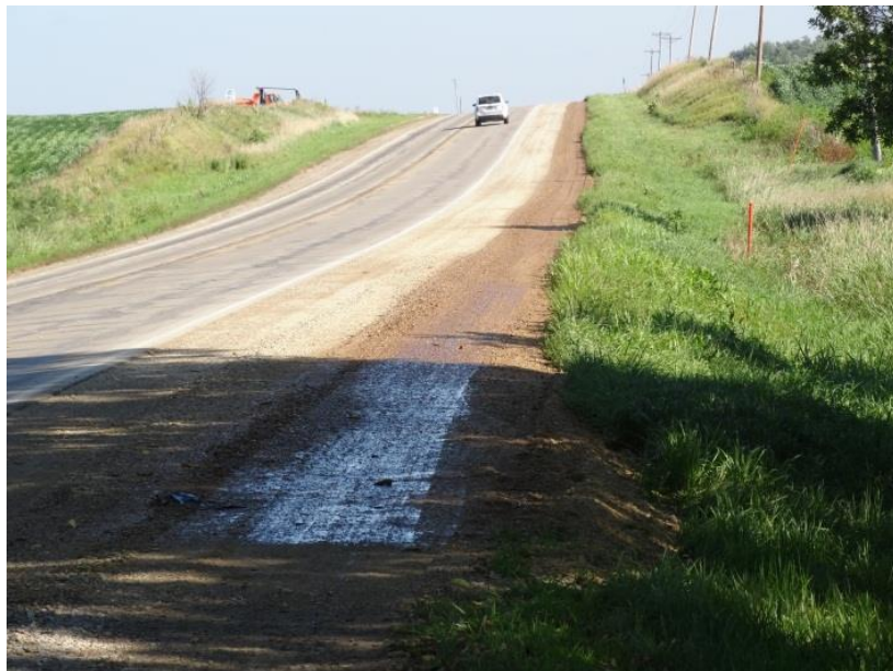
Figure 9. Soapstock applied on the shoulder of US 69 up the hill near Leland, Iowa
