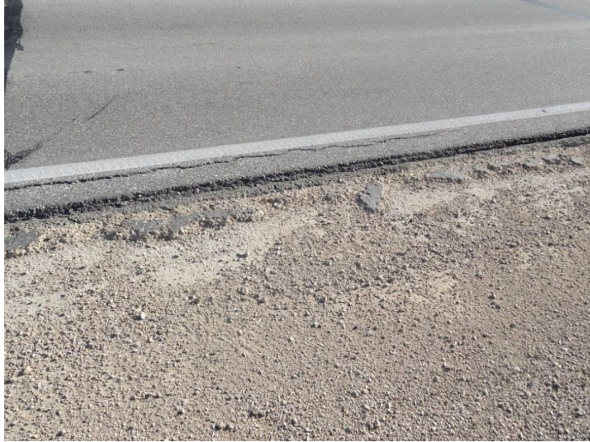
Figure 26. Soapstock missing east of Allison, Iowa
