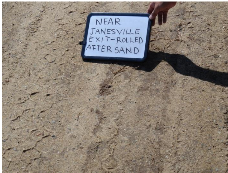
Figure 14. Surface rolled after sand application for the shoulder of US 63 near Denver, Iowa
