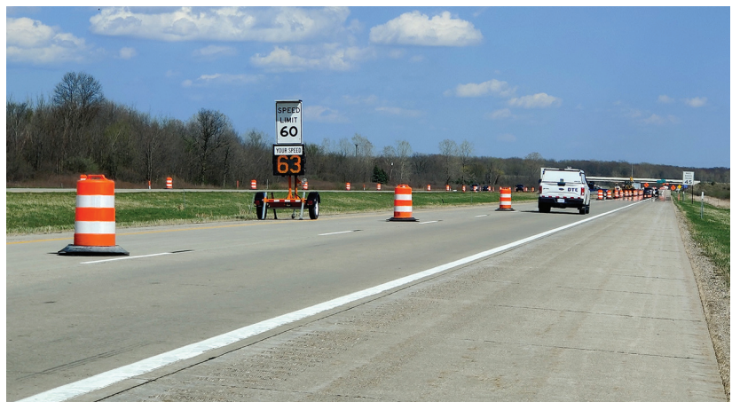
Speed feedback trailer positioned at the end of lane closure taper on westbound I-69 work zone in Michigan
