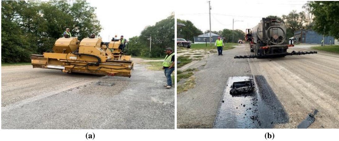
Figure 34. Calibration of equipment prior to Otta seal application: (a) adjusting aggregate application rate and (b) adjusting binder application rate
