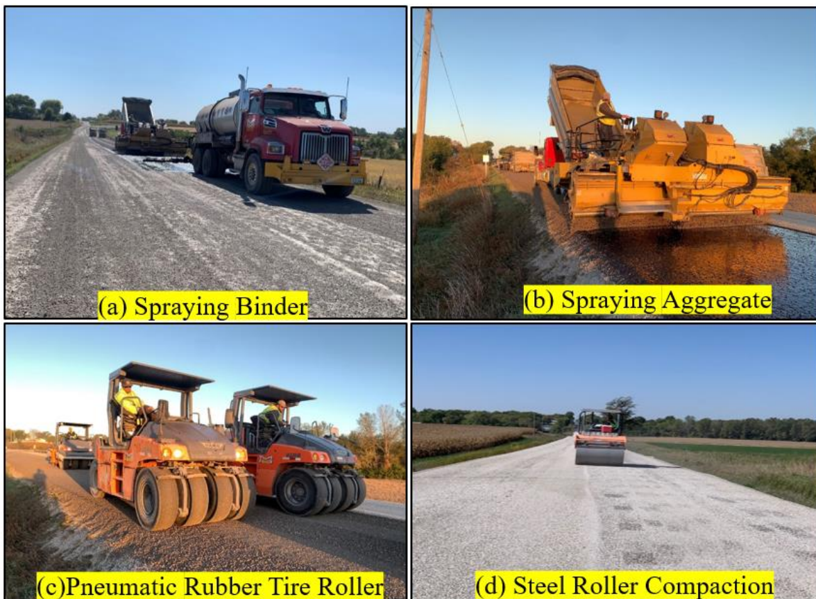
Figure 35. Otta seal construction on County Road J55: (a) spraying of MC 3000 binder, (b) distribution of limestone aggregate, (c) compaction using pneumatic rubber tire roller, and (d) center line compaction using steel drum roller
