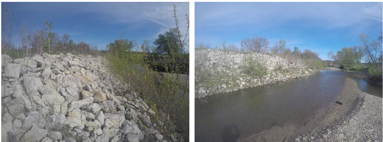
Figure 29. Loose riprap during low water levels in Madison County, Iowa
