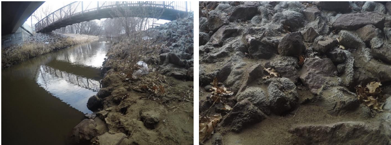
Figure 16. Minnesota Site 1: Partially grouted riprap
