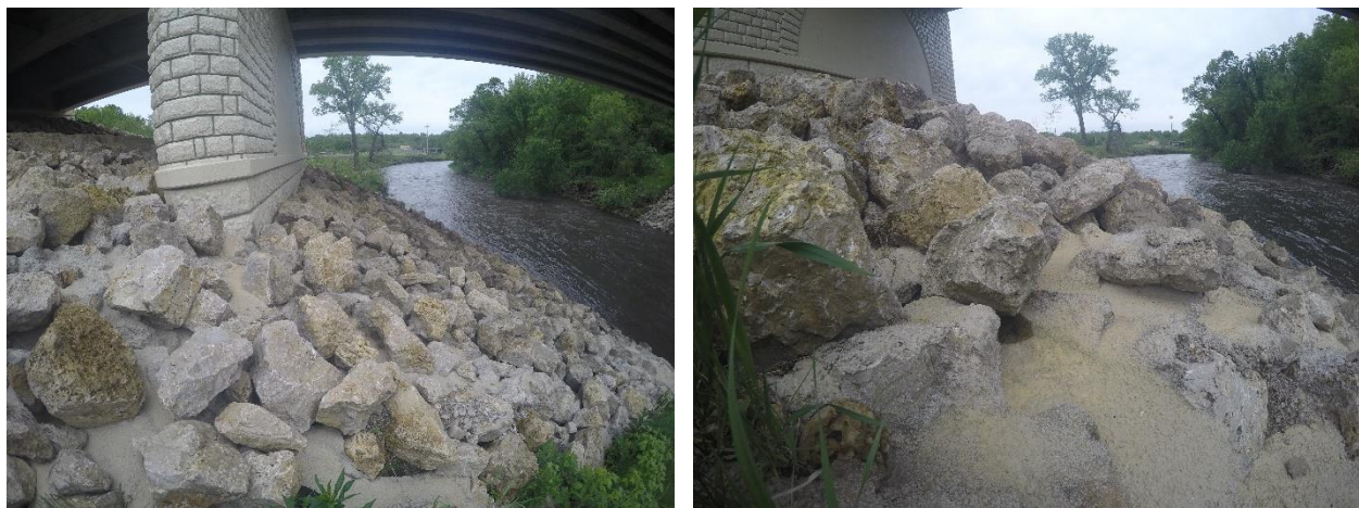
Figure 18. Minnesota Site 3: Partially grouted riprap—thin grout
