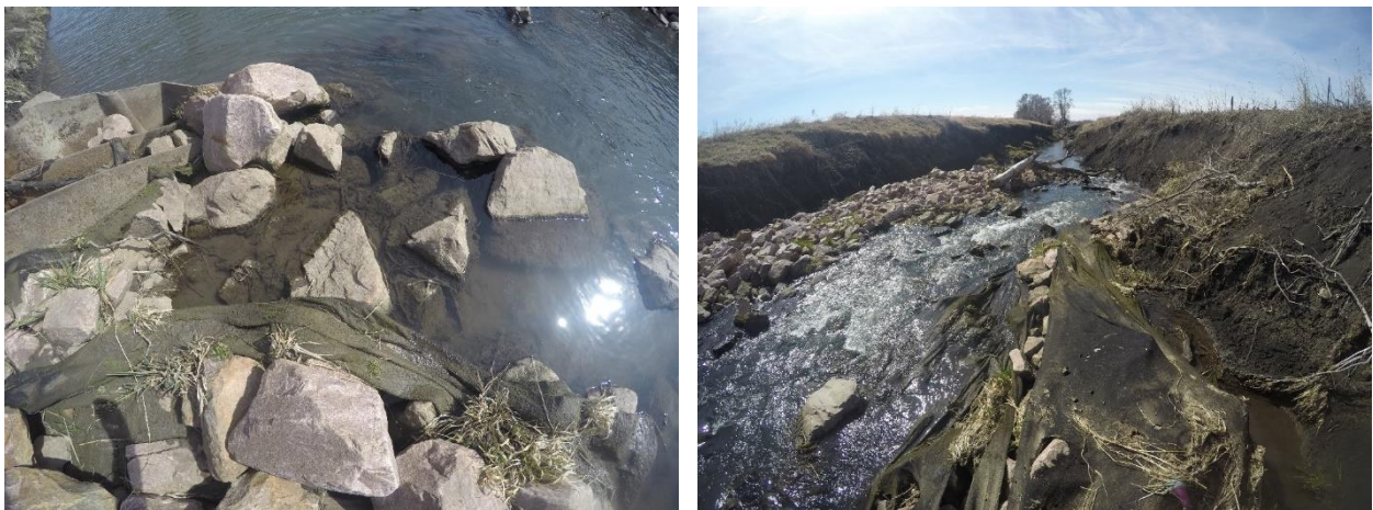
Figure 25. Failing stream grade control in Woodbury County, Iowa
